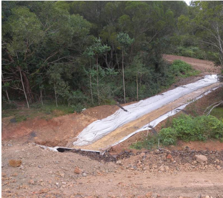
Stabilisation Matting Used to Stabilise Drainage Channel (Photo courtesy of O 2 Environmental)
