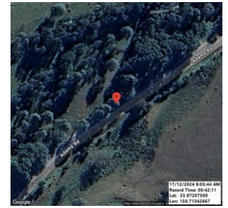
Alligator cracking in the roadway on Adams Road.
