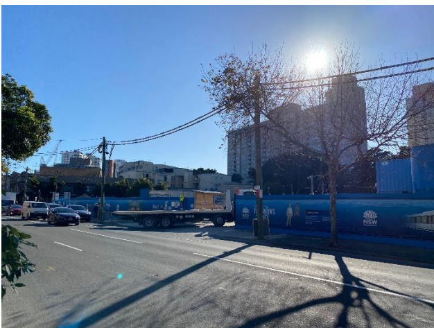
Picture 5 North western corner of site, looking north east illustrating station construction vehicular entrance
