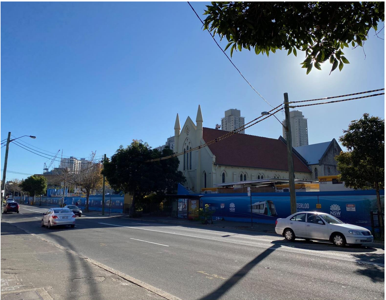
Figure 10 Photographs of existing site condition at Waterloo Metro Quarter site (dated 21 July 2020)
