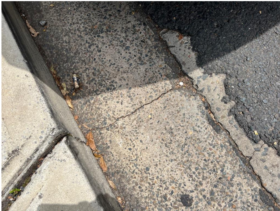
PHOTO 100 (Photo showing crack in gutter – Raglan Street)
