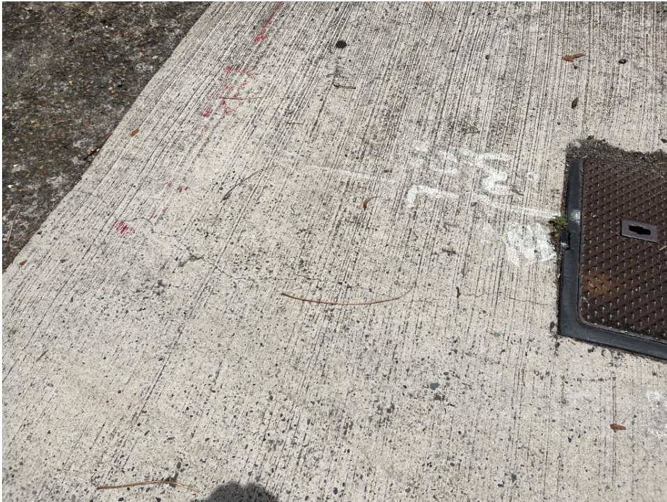
PHOTO 221 (Photo showing crack in footpath – Botany Road)
