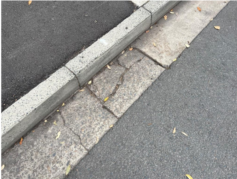
PHOTO 25 (Photo showing cracks in gutter – Raglan Street)
