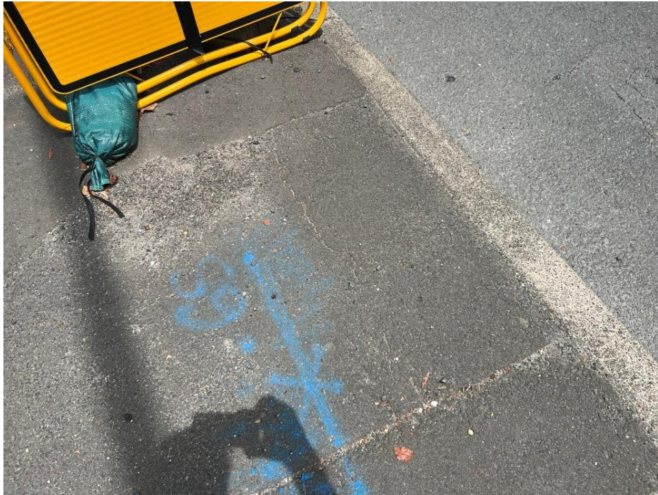
PHOTO 291 (Photo showing crack in footpath – Botany Road)
