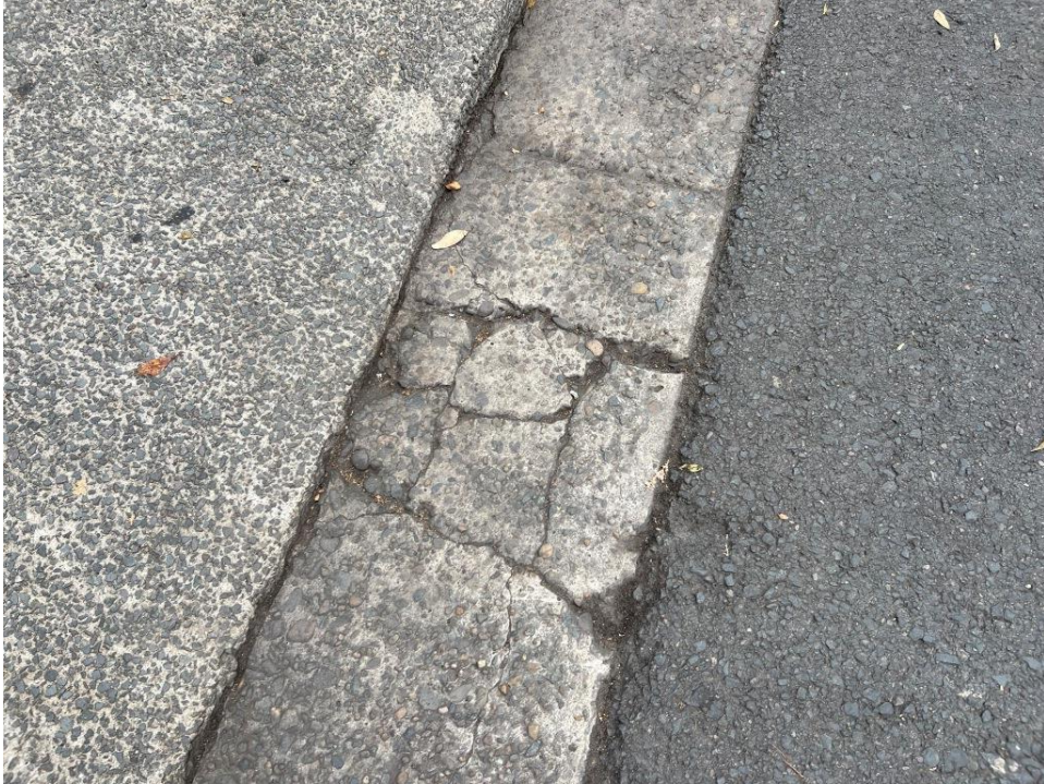
PHOTO 19 (Photo showing cracked gutter – Raglan Street)
