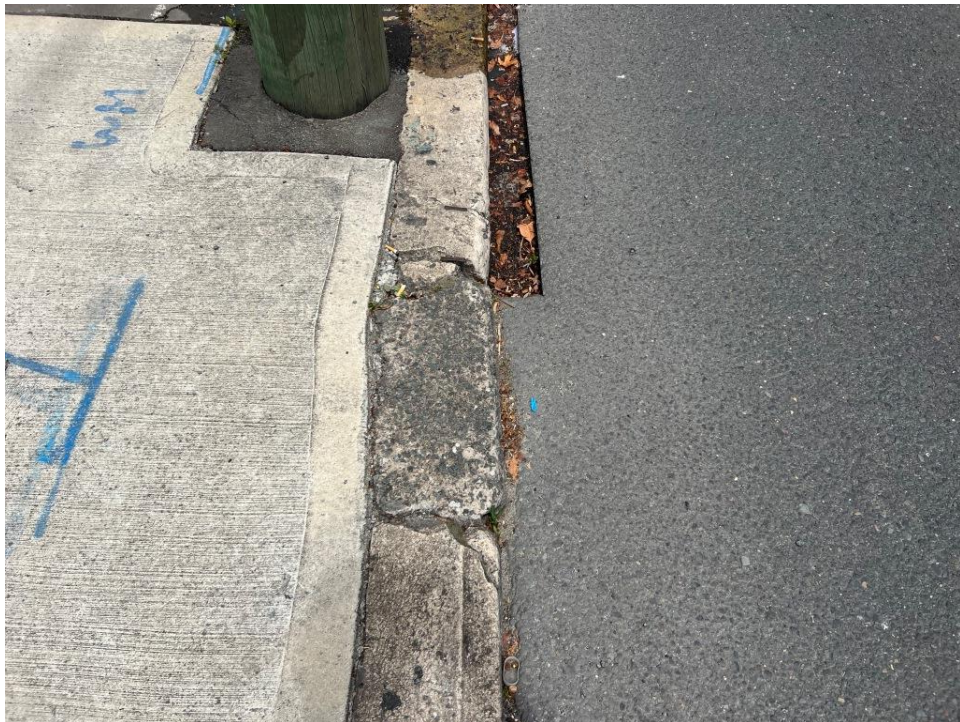
PHOTO 348 (Photo showing cracked/damaged kerb – Botany Road)
