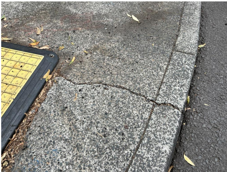
PHOTO 8 (Photo showing crack in footpath and kerb – Raglan Street)
