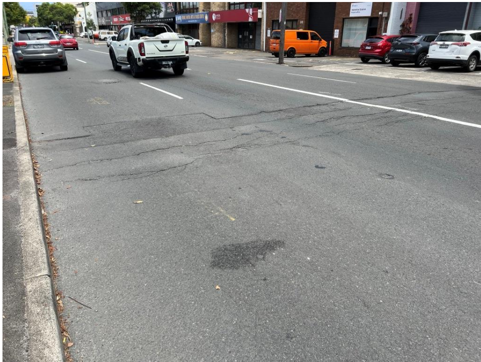
PHOTO 280 (Photo showing cracks in asphalt – Botany Road)
