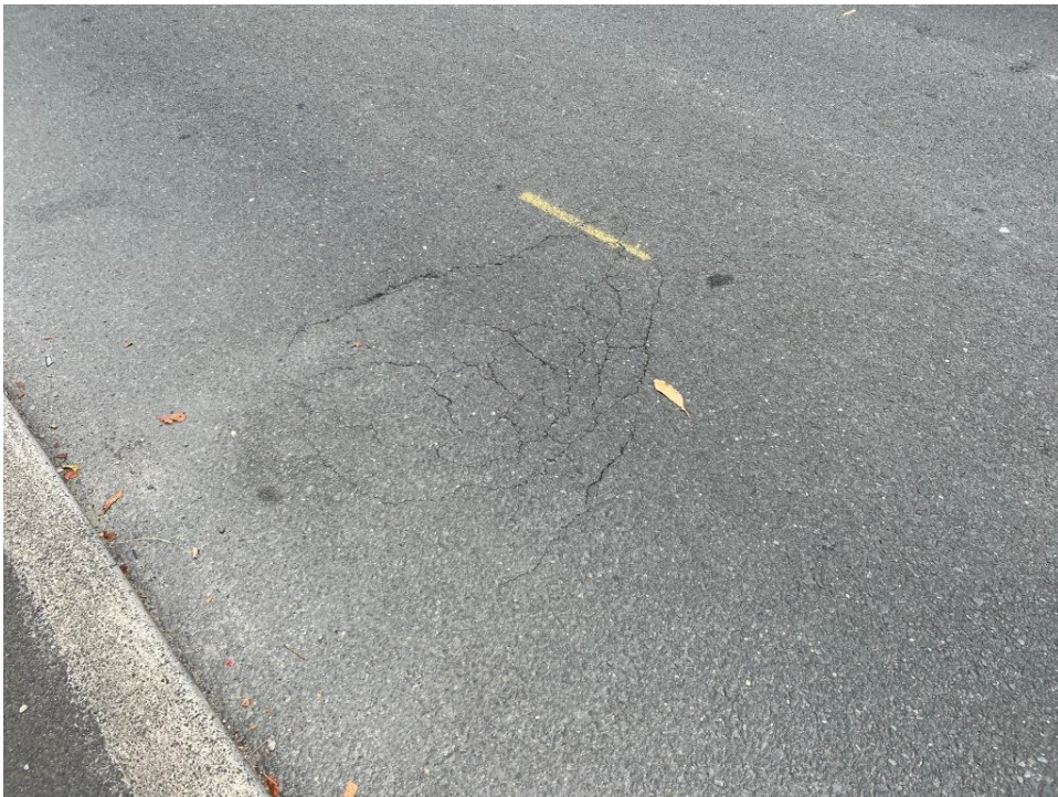
PHOTO 272 (Photo showing cracks in asphalt – Botany Road)
