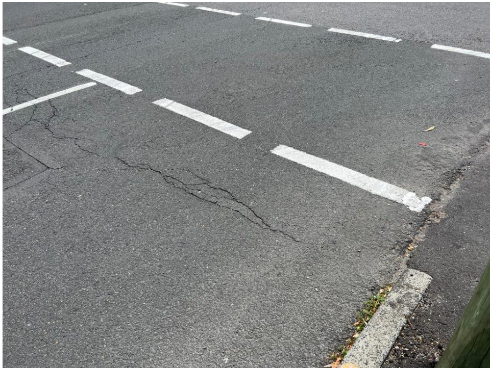
PHOTO 158 (Photo showing cracked asphalt – Botany Road)
