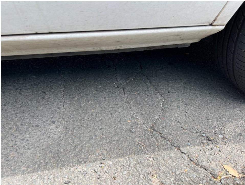
PHOTO 192 (Photo showing cracks in asphalt – Botany Road)
