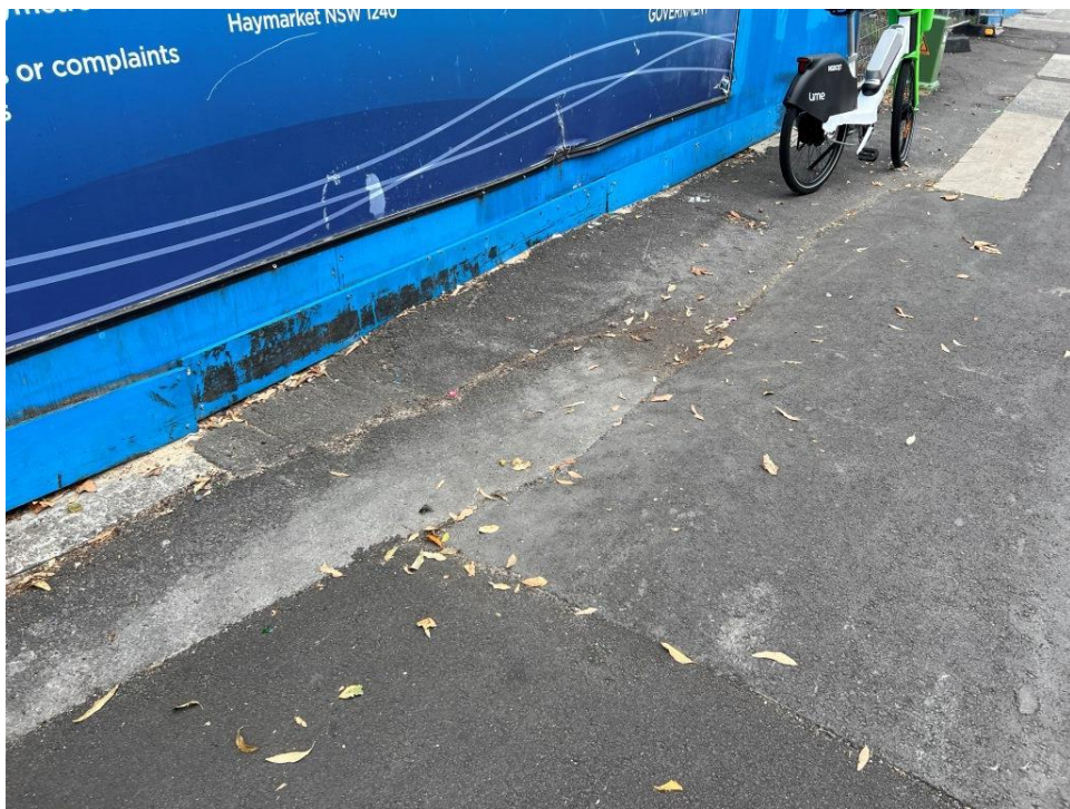
PHOTO 28 (Photo showing uneven footpath – Raglan Street)
