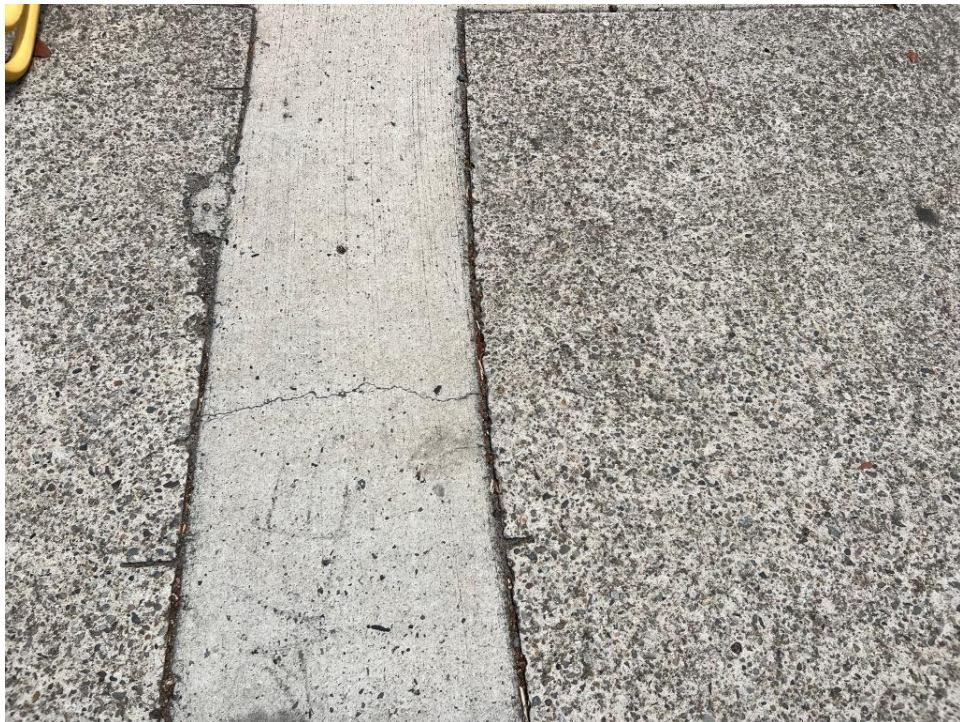
PHOTO 252 (Photo showing crack in footpath – Botany Road)
