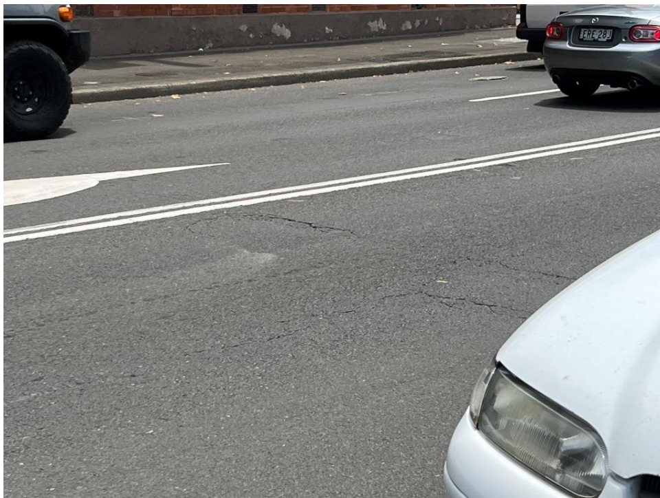
PHOTO 190 (Photo showing cracks in asphalt – Botany Road)
