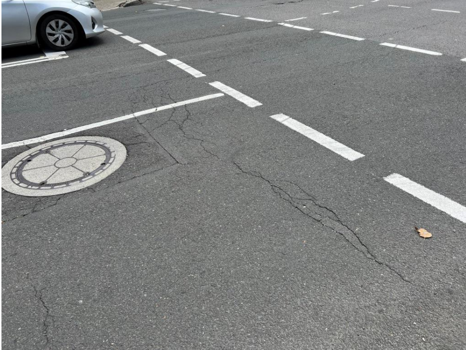
PHOTO 159 (Photo showing cracked asphalt – Botany Road)
