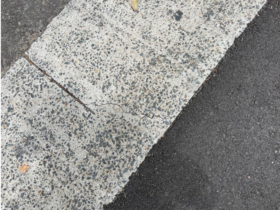
PHOTO 65 (Photo showing crack in footpath – Raglan Street)
