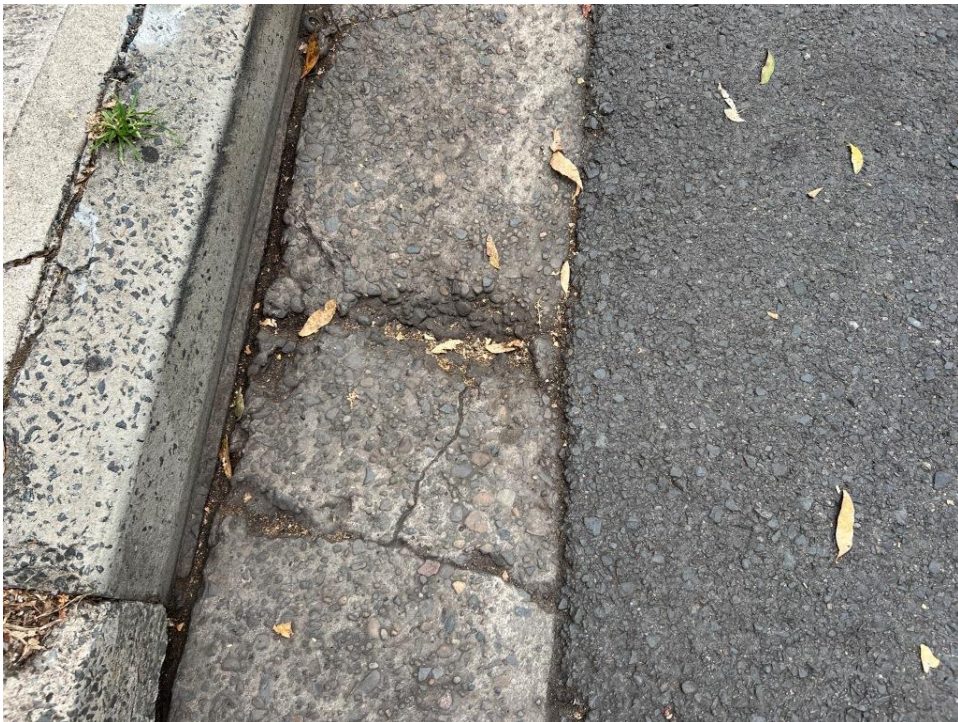
PHOTO 20 (Photo showing cracked kerb and gutter – Raglan Street)
