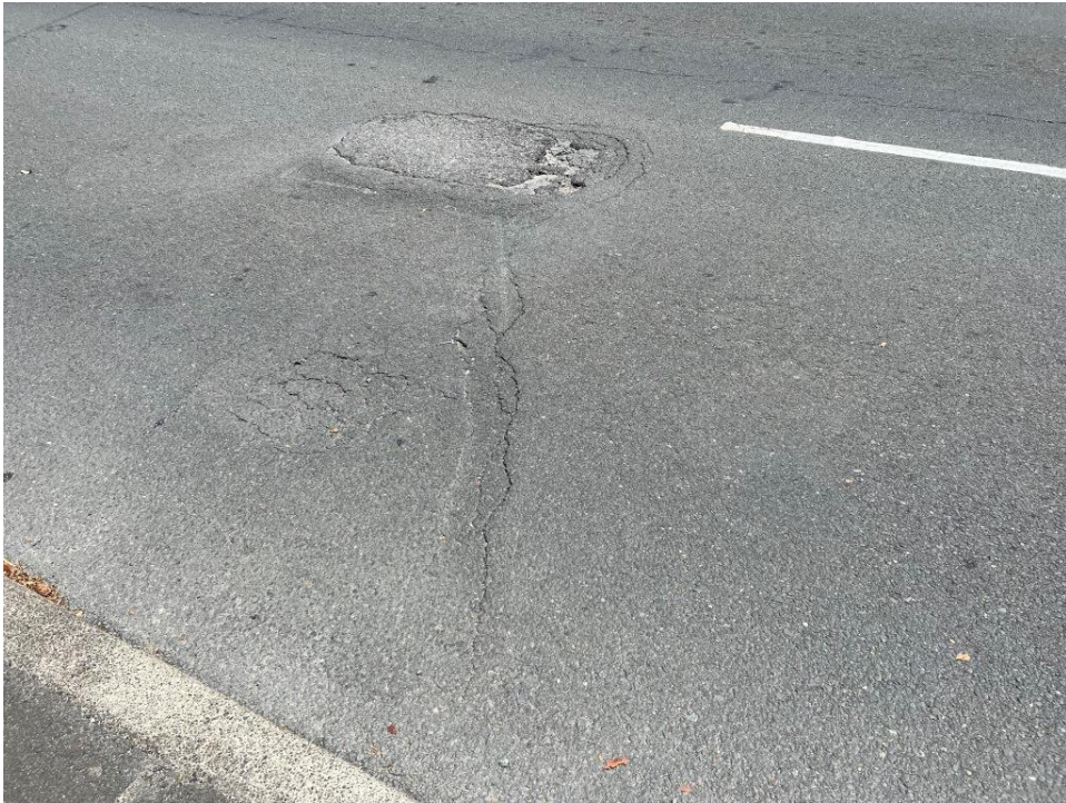
PHOTO 289 (Photo showing crack in asphalt – Botany Road)
