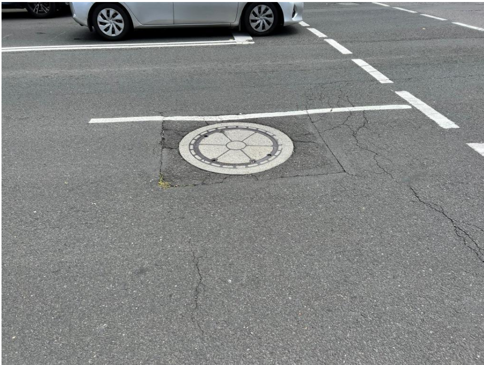
PHOTO 160 (Photo showing cracked asphalt – Botany Road)
