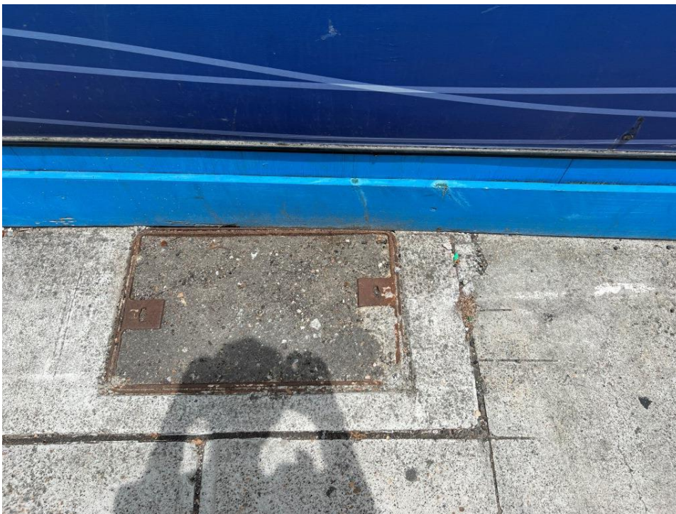
PHOTO 108 (Photo showing condition of footpath around pit – Raglan Street)
