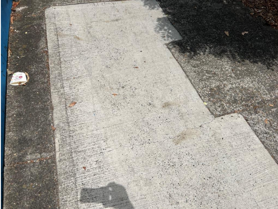
PHOTO 223 (Photo showing crack in footpath – Botany Road)
