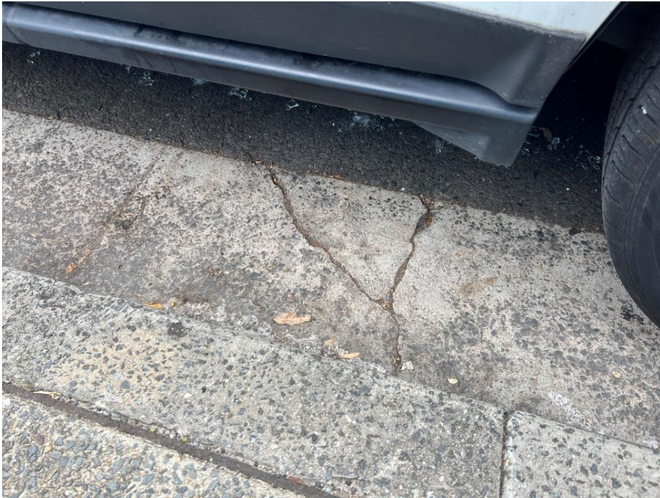
PHOTO 71 (Photo showing cracks in gutter – Raglan Street)
