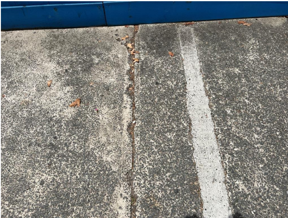
PHOTO 196 (Photo showing chipped concrete along footpath's joint – Botany Road)
