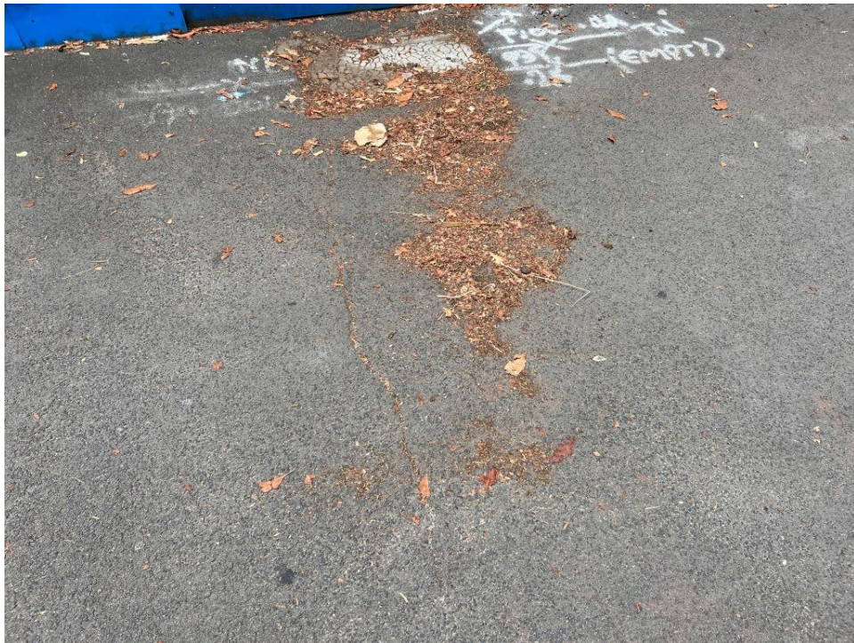
PHOTO 282 (Photo showing cracks and uneven footpath surface – Botany Road)
