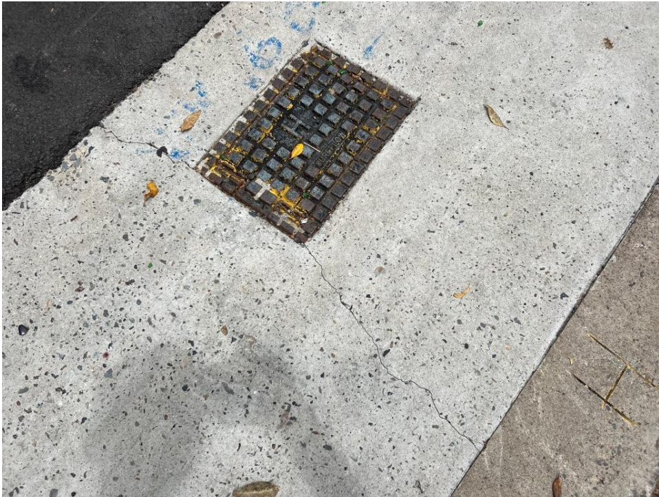
PHOTO 41 (Photo showing cracks in footpath – Raglan Street)
