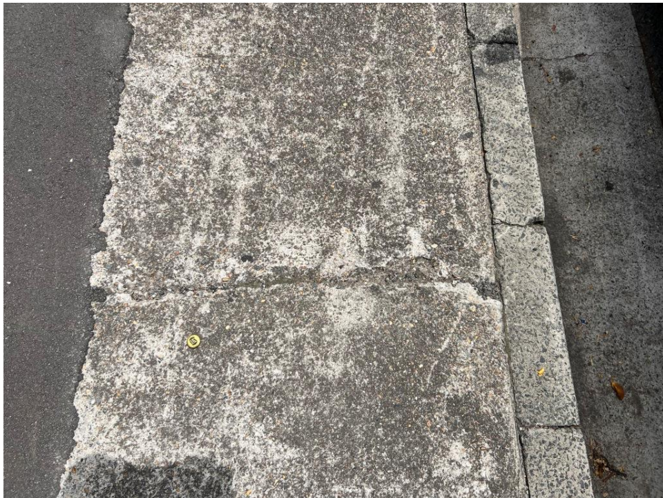
PHOTO 116 (Photo showing crack/missing concrete in footpath – Raglan Street)
