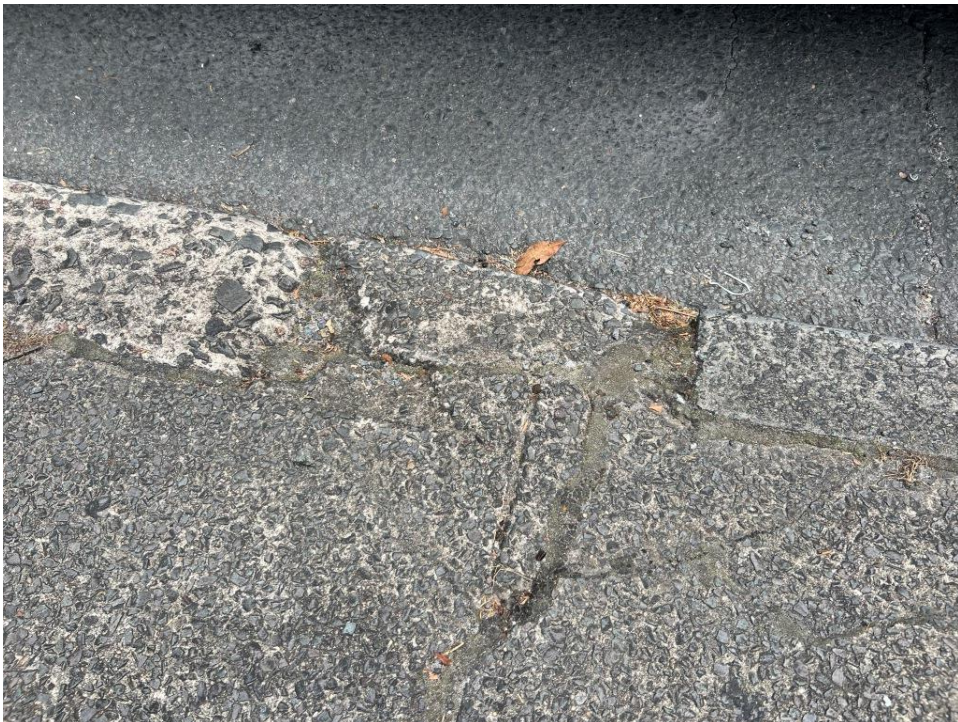
PHOTO 184 (Photo showing cracks/missing concrete in footpath and kerb – Botany Road)
