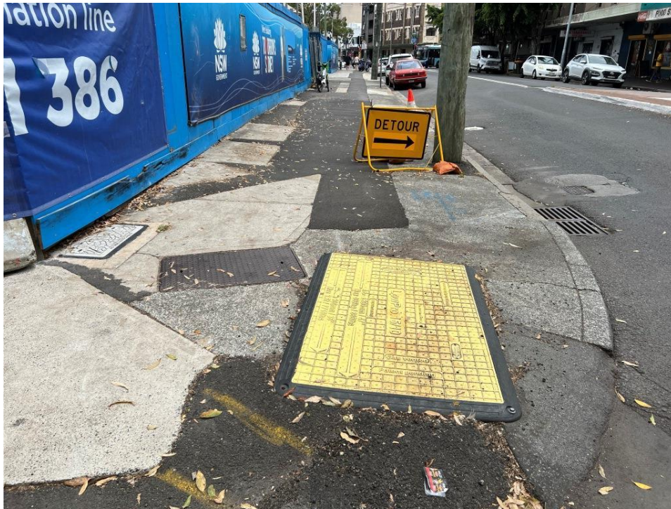
PHOTO 7 (Overview of uneven footpath – Raglan Street)
