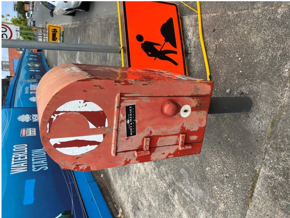
PHOTO 170 (Photo showing condition of mails drop off station – Botany Road)
