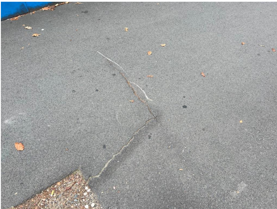
PHOTO 268 (Photo showing crack in footpath – Botany Road)
