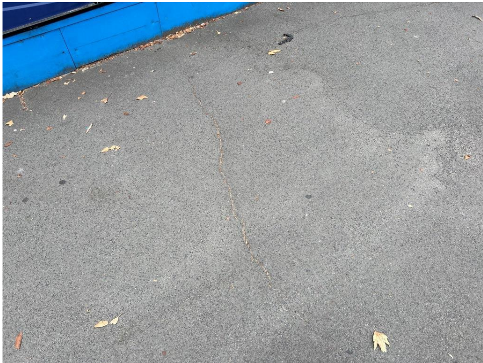
PHOTO 274 (Photo showing crack in footpath – Botany Road)
