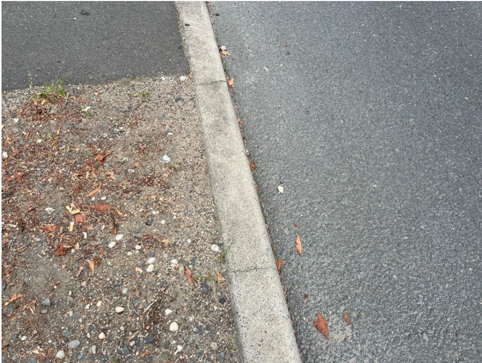
PHOTO 267 (Photo showing cracks in kerb – Botany Road)
