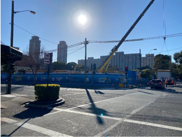
Picture 7 South western corner of site, located at the corner of Wellington Street and Botany Road
