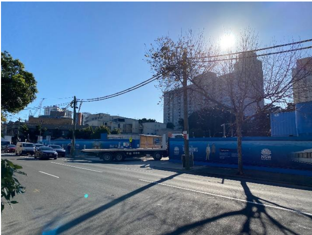
Picture 9 North western corner of site, looking north east illustrating station construction vehicular entrance
