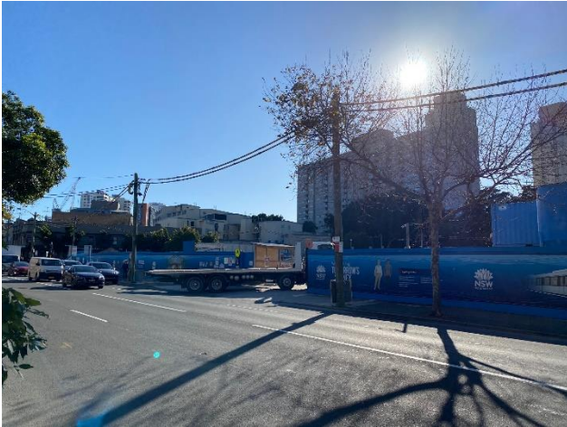
Picture 13 North western corner of site, looking north east illustrating station construction vehicular entrance
