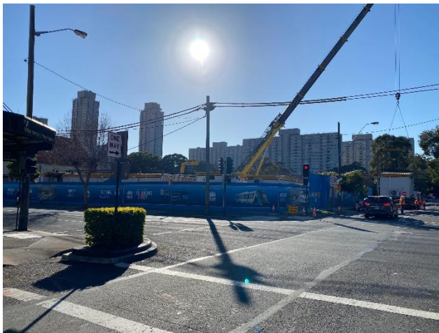
Picture 11 South western corner of site, located at the corner Wellington Street and Botany Road
