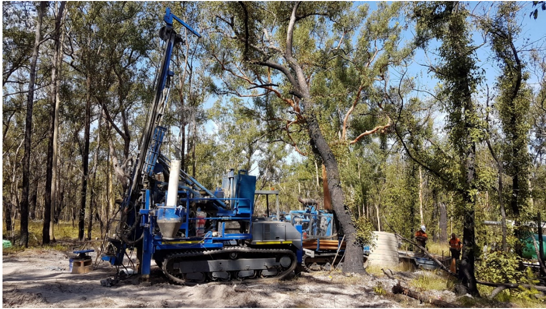
Plate 9 – Wallis Mantis 300 track mounted drill rig supported by track-mounted rod carrier with air compressor. Drill hole ARDG-DDH01 – January 2018
