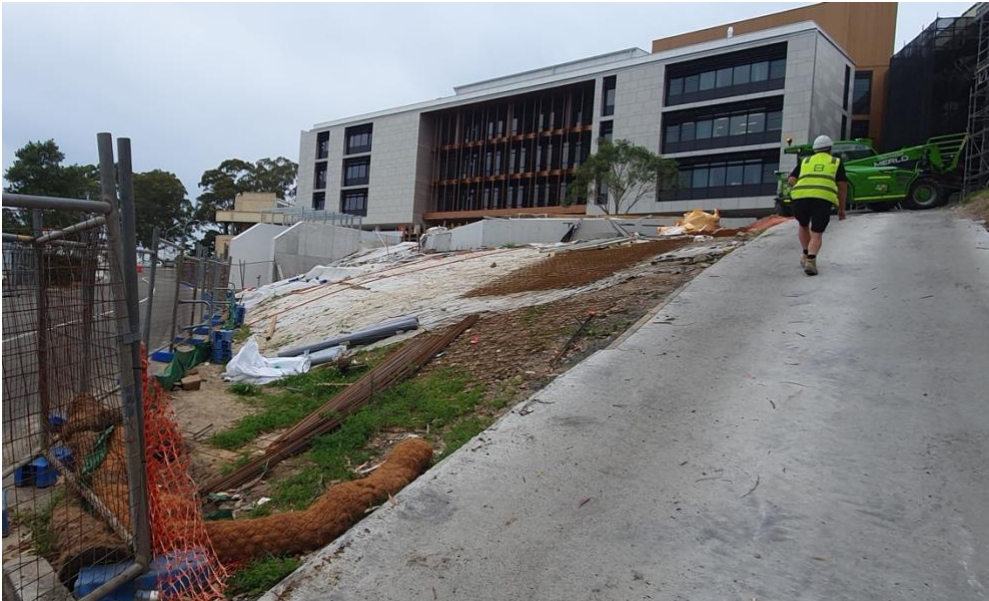
Figure 1-2 Geo-fabric and temporary concrete access on slope reducing the risk of sediment transportation through erosion.
