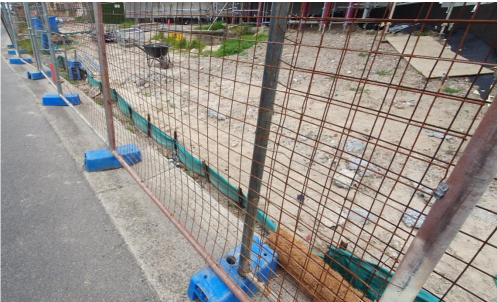
Figure 1-8 Sediment fence, in place, but removal of excess sedimentation required.
