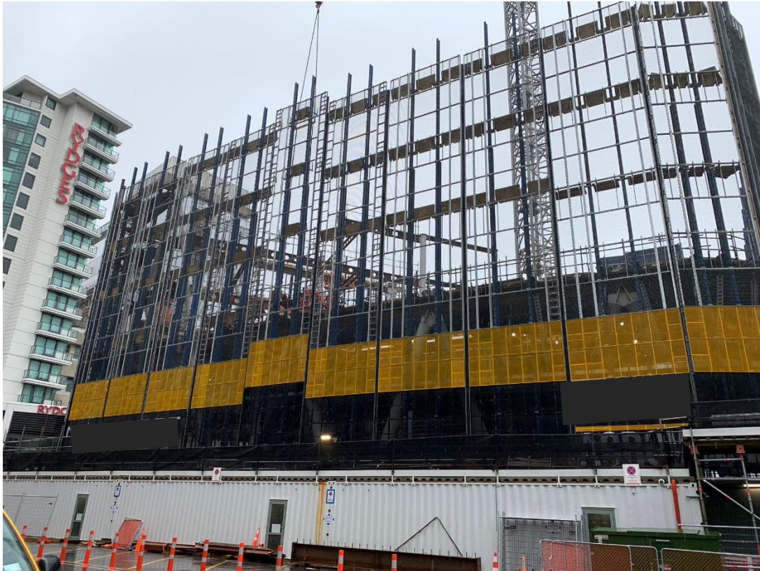
Figure 1-57a: Photo example of screens
