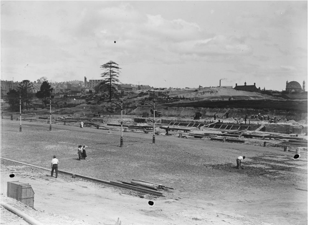
Figure 77 – Eddy Avenue, levelled site with tramline stanchions in place, before paving. Looking southeast, cleared land for Central Station
