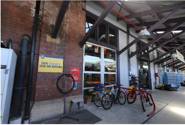
Figure 8 – East elevation of the shed, with the timber expressed frame and masonry and sandstone piers.
