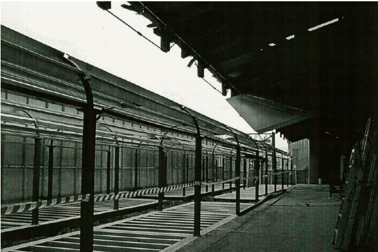
Figure 101 – Reproduction train carriages under construction at Inwards Parcels Shed, 2003. Source: City of Sydney Archives, DA1999/00684 Part 1.
