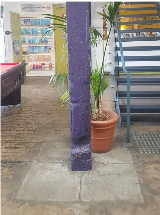
Figure 32 – Detail of timber column with signs of wear from original use
