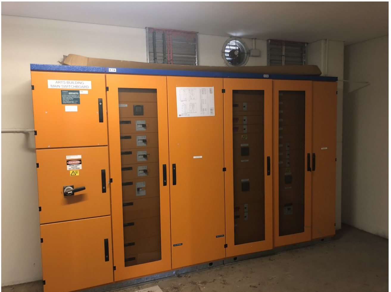
Figure 3 – Existing ARTS Main Switchboard (MSB) There is adequate spare capacity at this switchboard for the new building
