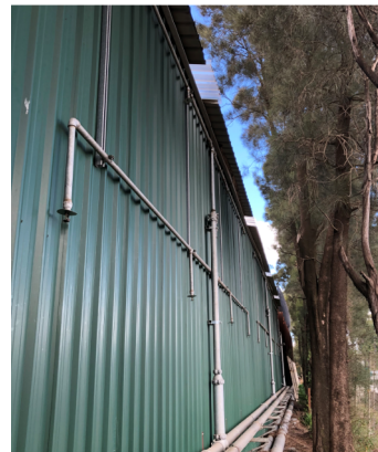
Wall wetting sprinkler connected to fire hydrant system.
