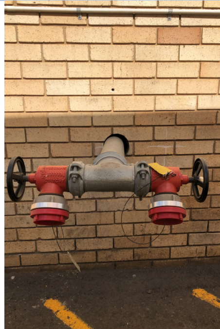
FH 3 missing adequate support
