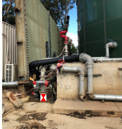
Isolation valve required for FH22 shown above
