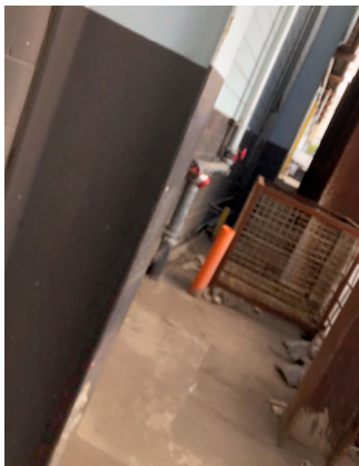
Fire hydrant (FH30) not shown on block plan.
