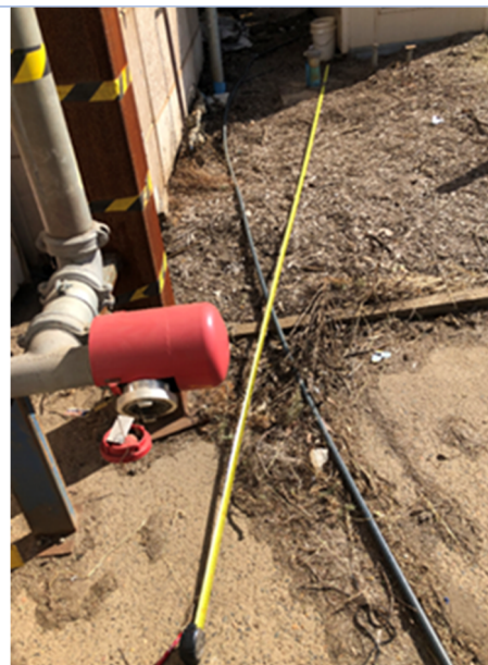
FH29 located too close to substation
