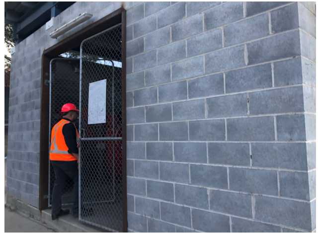
Fire hydrant pumproom missing signage.
