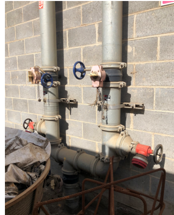
External fire hydrants (FH10 and FH11) and isolation valves (SV9, SV10, SV11) obstructed by plant equipment.
