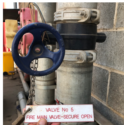
Numbered isolation valve (SV5).
