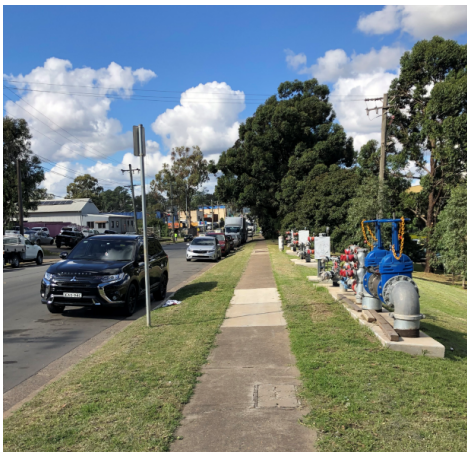
Vehicles parked on fire brigade hardstand.
