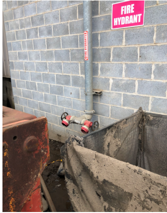
External fire hydrant (FH7) obstructed by plant equipment.
