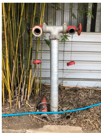
Existing external fire hydrant
