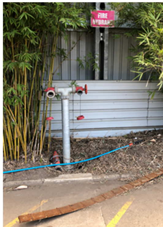
FH5 without bollard protection and storz
