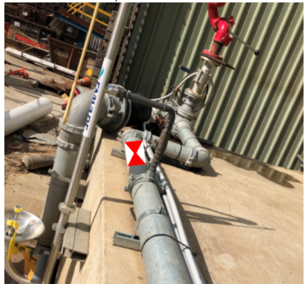
Isolation valve for connections from fire hydrant pipework, shown on block plan.
