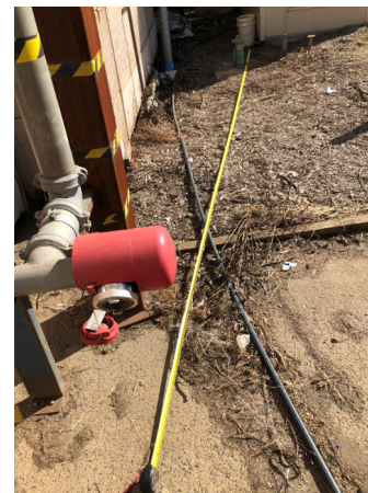
Fire hydrant located within 10m of substation.
