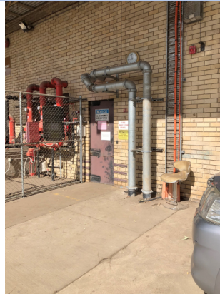
Risers entering Building B from SV1 and SV2 without bollard protection
