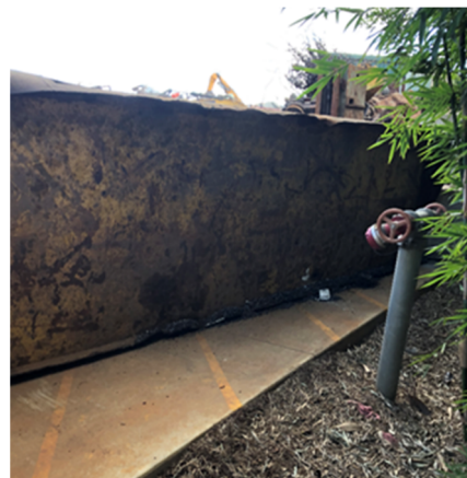
External fire hydrant obstructed by plant equipment
