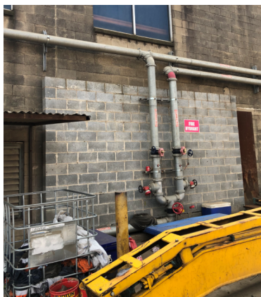
External fire hydrants and isolation valves obstructed by plant equipment
