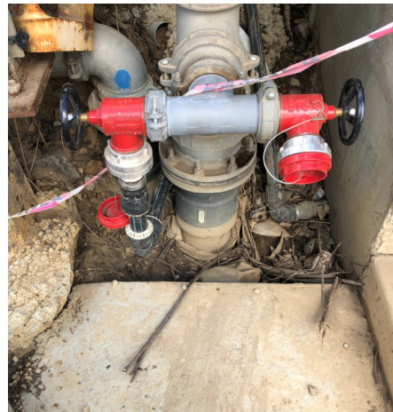
Fire hydrant installed too low (~600mm)
