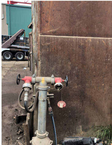
Foam fire hydrant (FH19).
