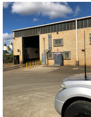
Risers entering Building B from SV19 and SV20 without bollard protection
