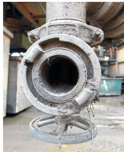
Fire hydrant (FH27) blocked with debris.
