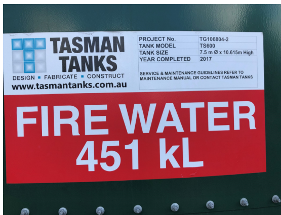
Fire hydrant tank label.
