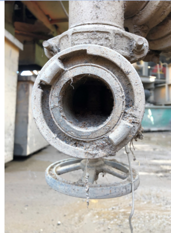
FH27 blocked by debris
