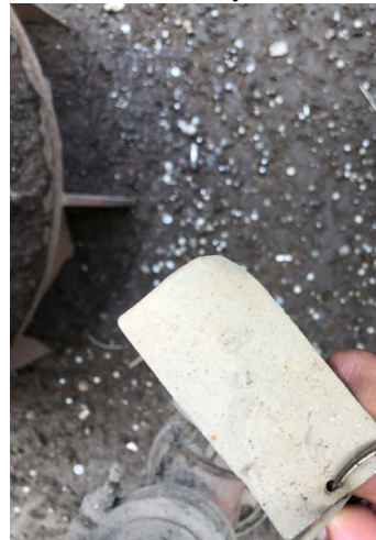
FH27 unreadable maintenance tag
