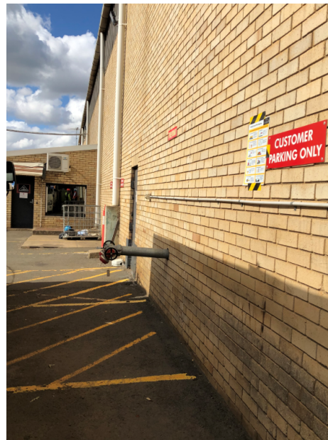
FH 3 missing adequate support and bollard
