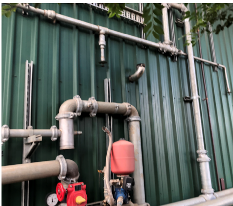
Drencher control valve.
