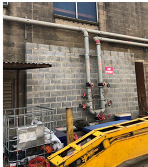
FH14 and FH15 obstructed by equipment
