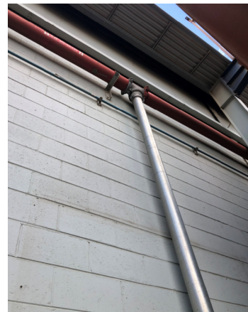
Supply from old sprinkler pipe for fire hydrant (FH30) not shown on block plan.
