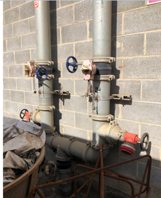
FH10 and FH11 obstructed by equipment
