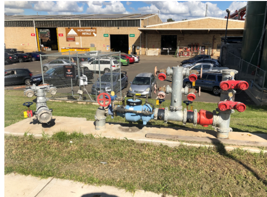
Fire hydrant booster assembly
