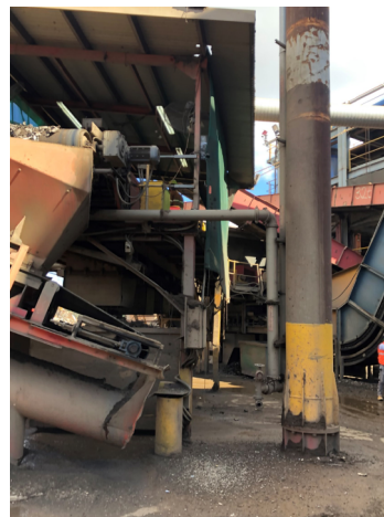
FH27 blocked by debris
