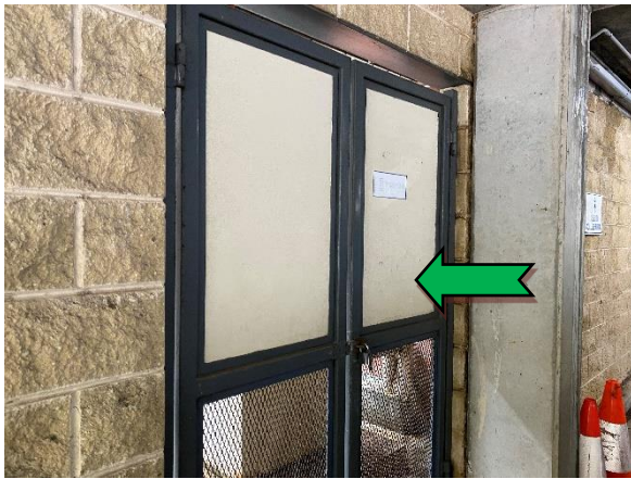
Photo 1 Exterior: carpark, plant room doors, infill panels – non-asbestos containing fibre cement sheeting.
