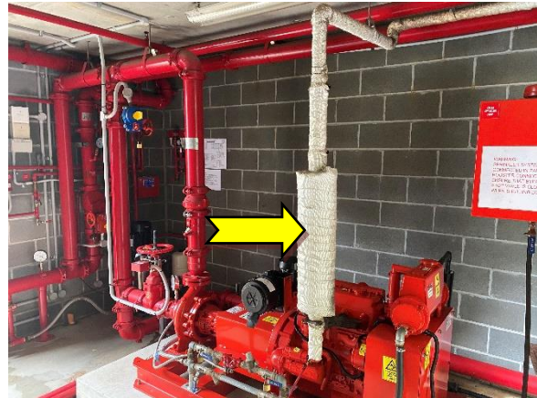
Photo 4 Interior: pump room, booster pump, pipe work – suspected SMF containing woven material.
