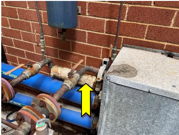
Photo 3 Exterior: AC plant room, pipe work – suspected SMF containing external insulation material.
