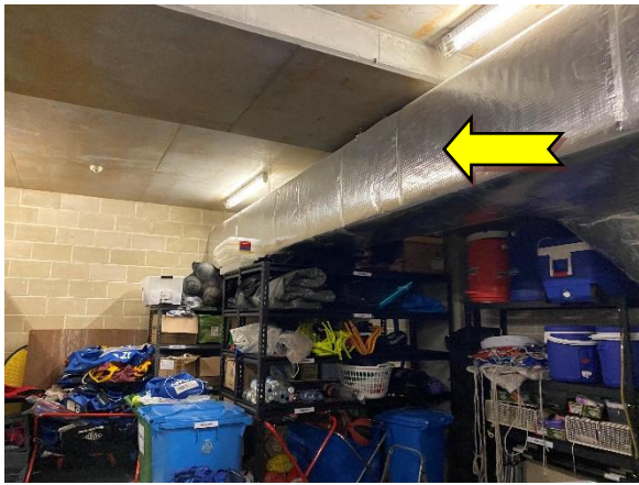
Photo 7 Interior: store room, air conditioning ductwork – suspected SMF containing external insulation material.
