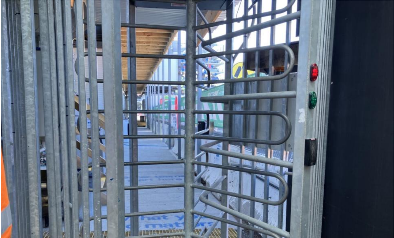
Access to site by turnstile and swipe card
