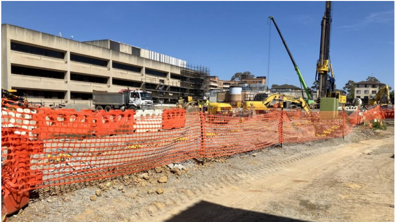
In-ground services occurring
