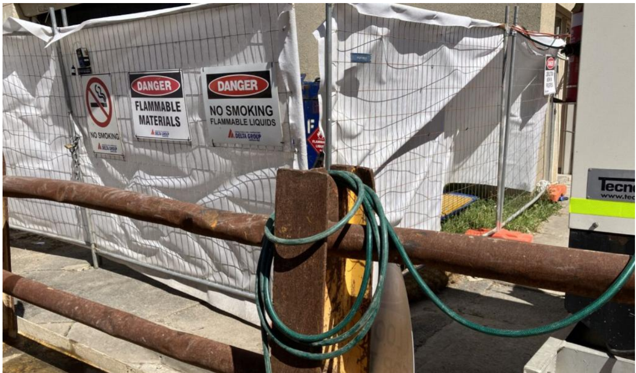
Hazardous substance storage. As per observation OBS-03, a spill kit is required.
