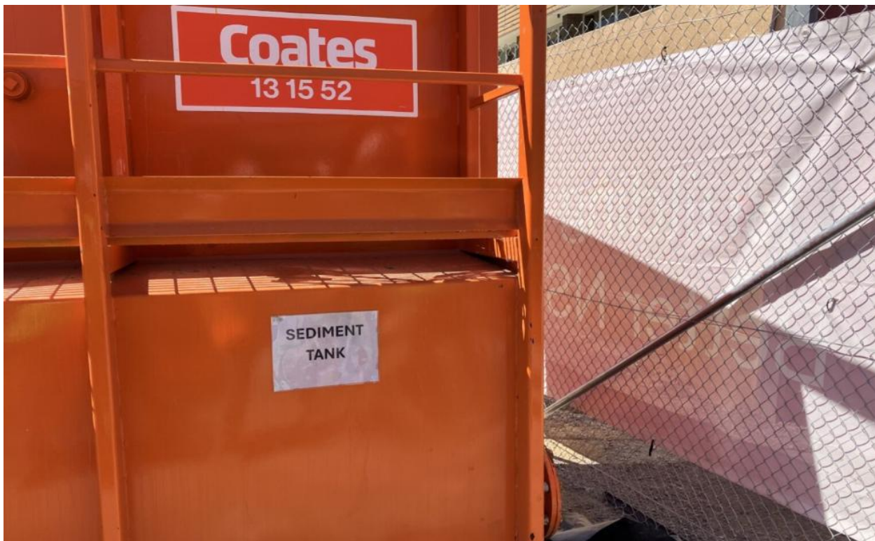
Coates sediment tank for water storage. LL confirmed no discharges have been required to date.
