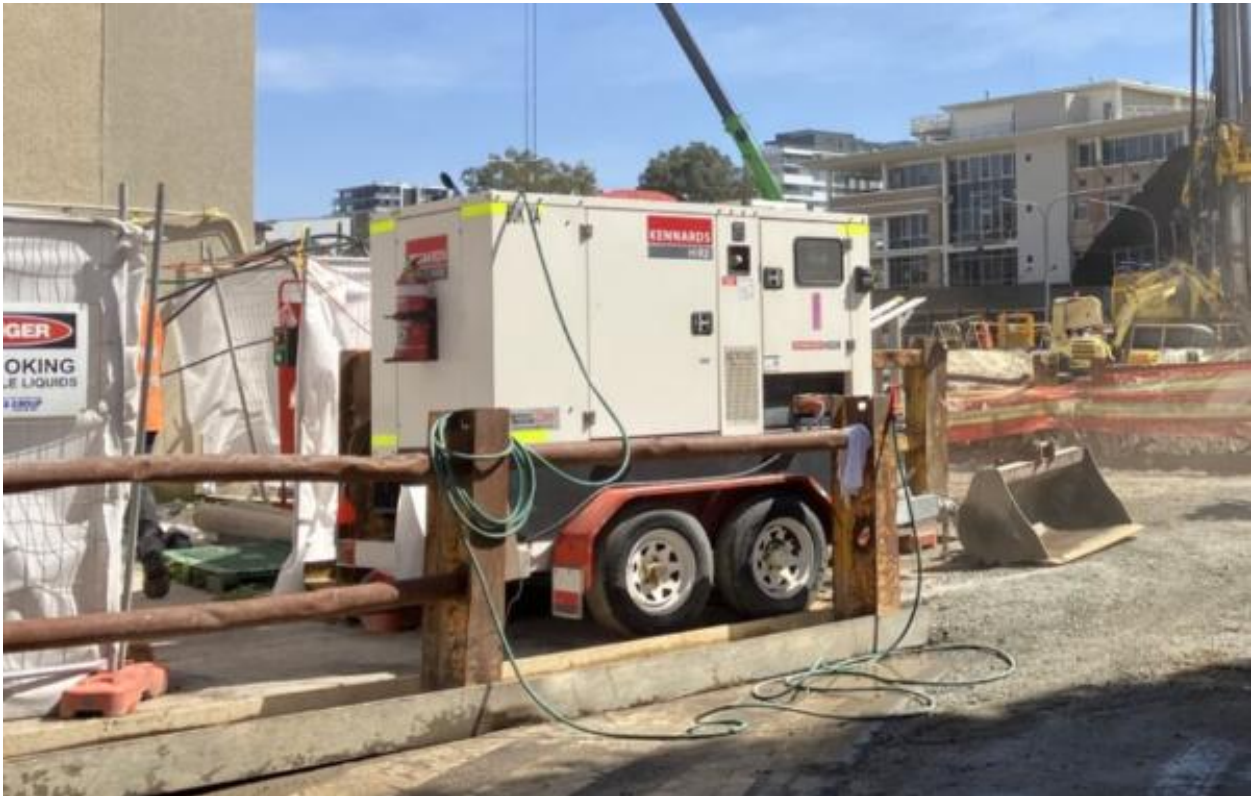
Generator onsite. As per observation OBS-03, a spill kit is required.
