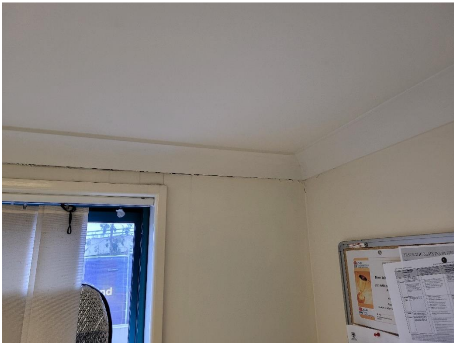
162. Water damage and cracking in plasterboard at wall and architrave around window opening to external wall
