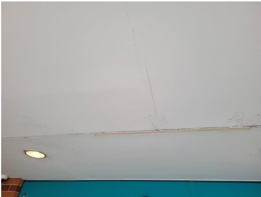
External 6. Damage and staining to external entrance way ceiling
