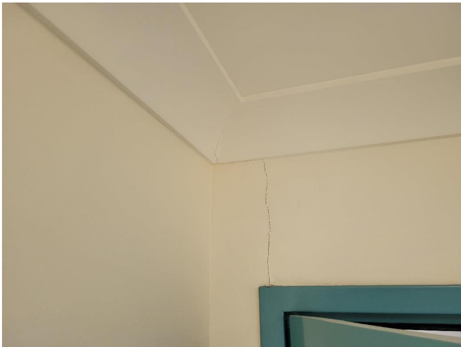
134. Crack in wall plasterboard from door frame to architrave
