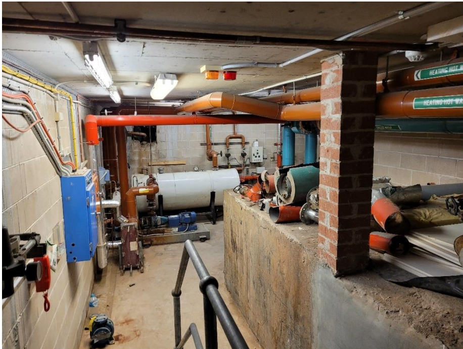
Service Tunnel 2. Access point under BIU, general abrasion or staining to surfaces
