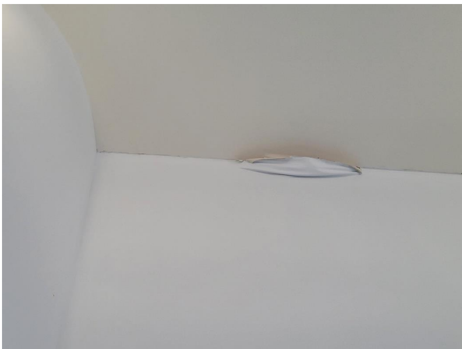
97. Damage to plasterboard at ceiling junction, uncertain whether water-borne or not
