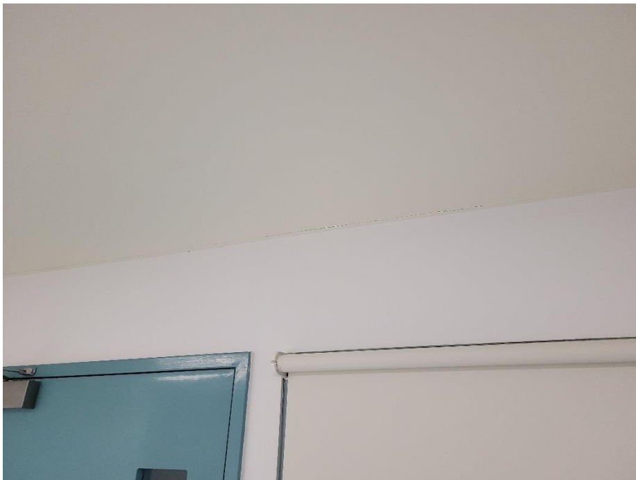
132. Crack in plasterboard at wall and ceiling junction
