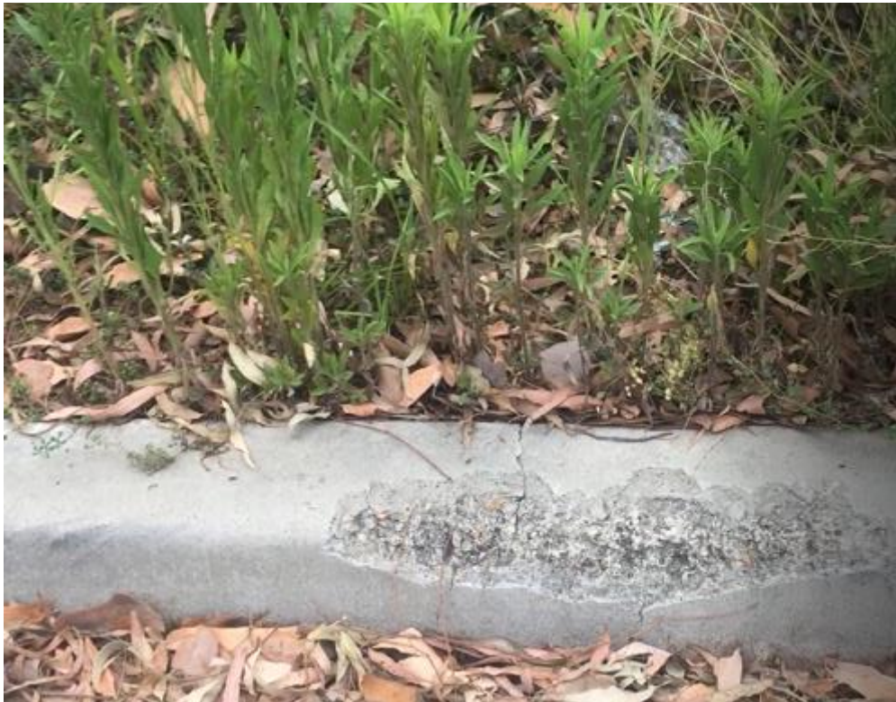
Burnside Drive 9. Cracked kerbing
