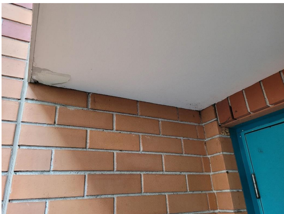
113. Water damage to eave soffit, cracking in external masonry adjacent door opening
