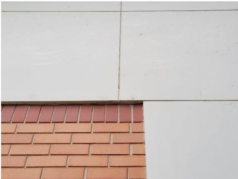
8. Damage to panel
