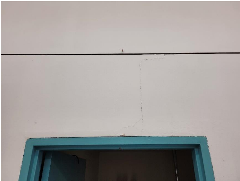
63. Vertical crack above door frame
