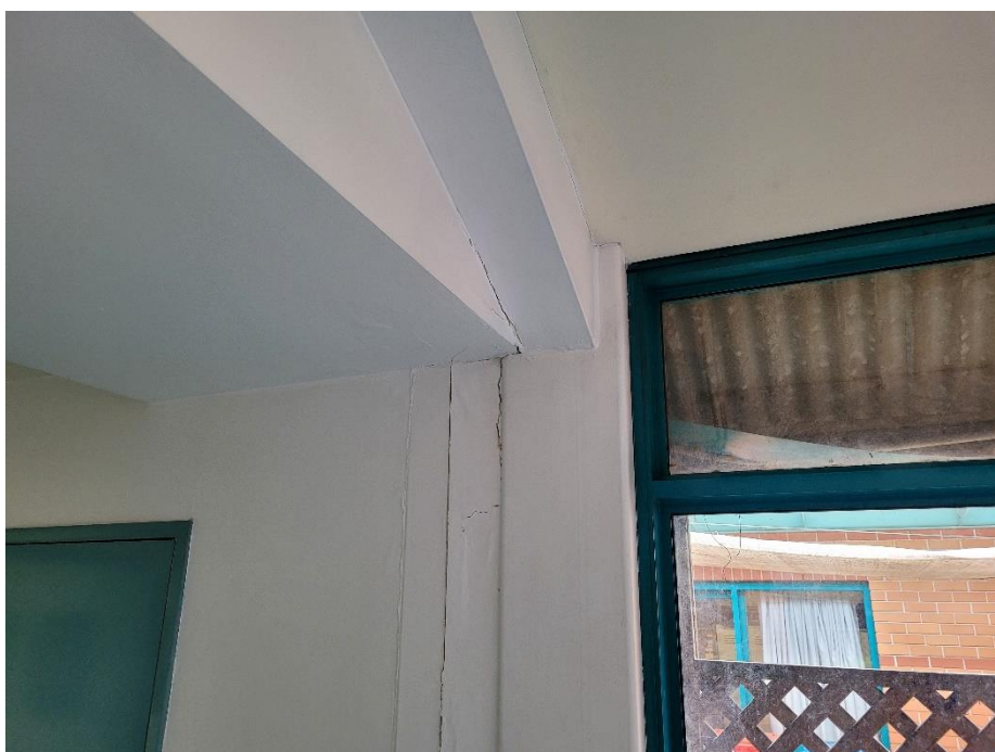
80. Cracking along junction with steel post, pitched ceiling, wall and lower ceiling
