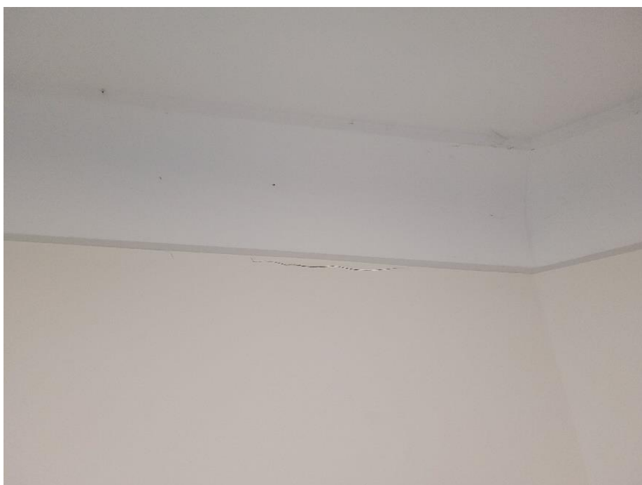
48. Crack in plasterboard at wall and ceiling junction
