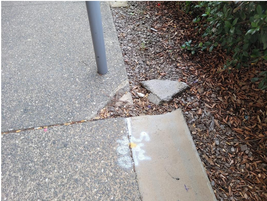
External 7a. Crack in kerb along walkway, parts of walkway surface coming away
