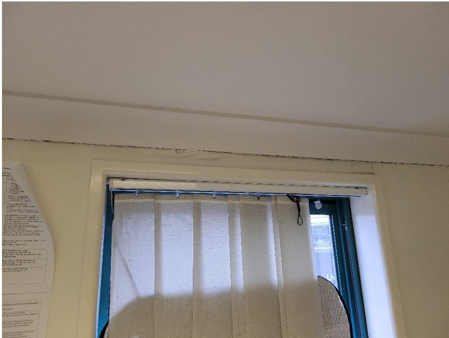
161. Water damage and cracking in plasterboard at wall and architrave around window opening to external wall
