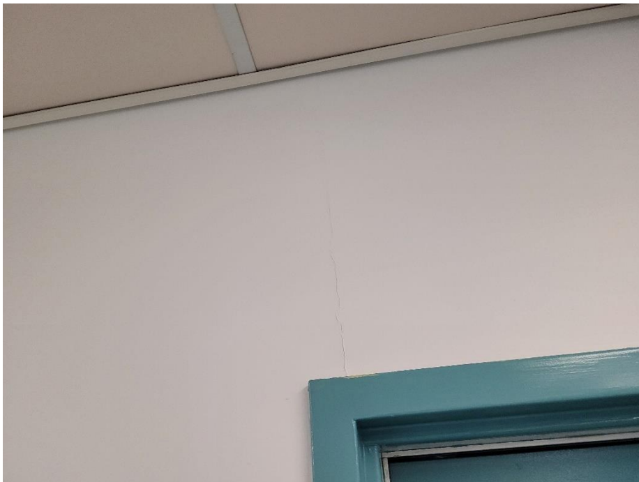
154. Vertical crack in plasterboard wall from door frame to false ceiling
