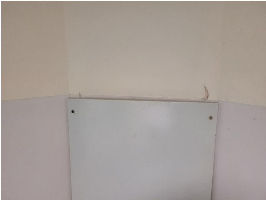
57. Damage to plasterboard around wall patch and anchor points
