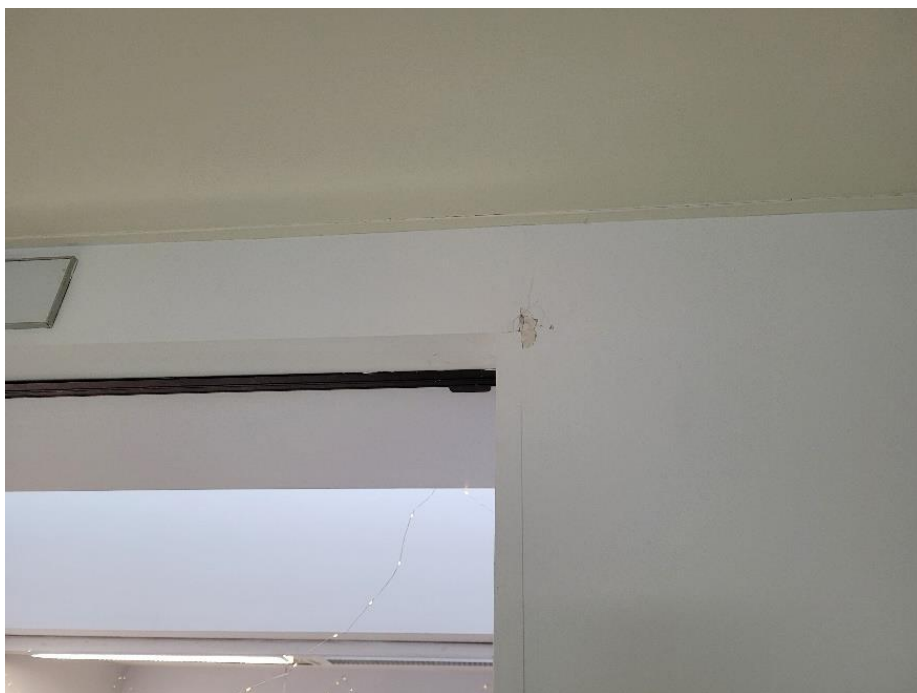
23. Damage to plasterboard in opening corner
