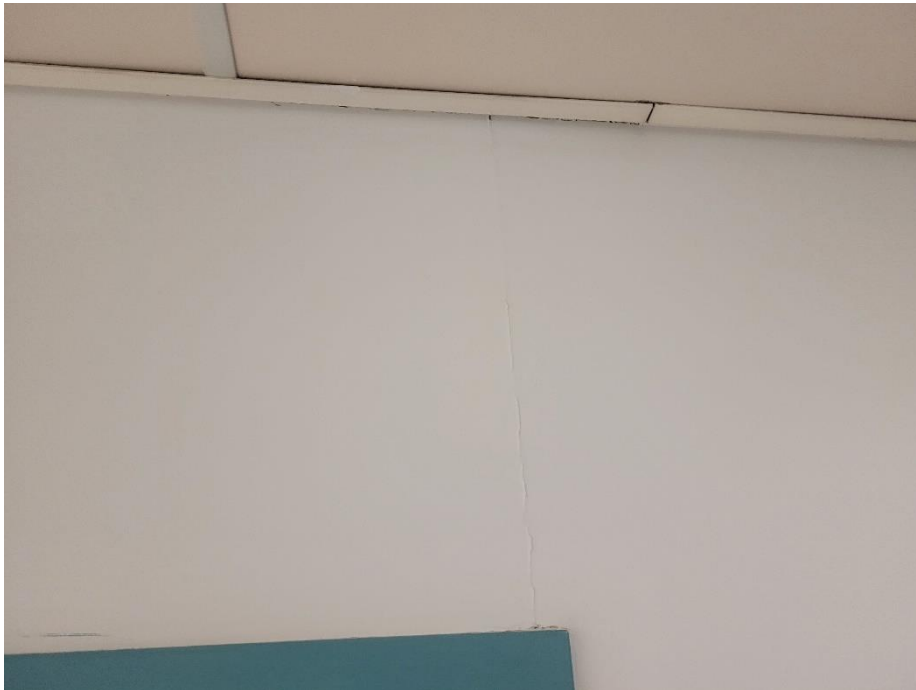
119. Vertical cracking from top of door frame to false ceiling
