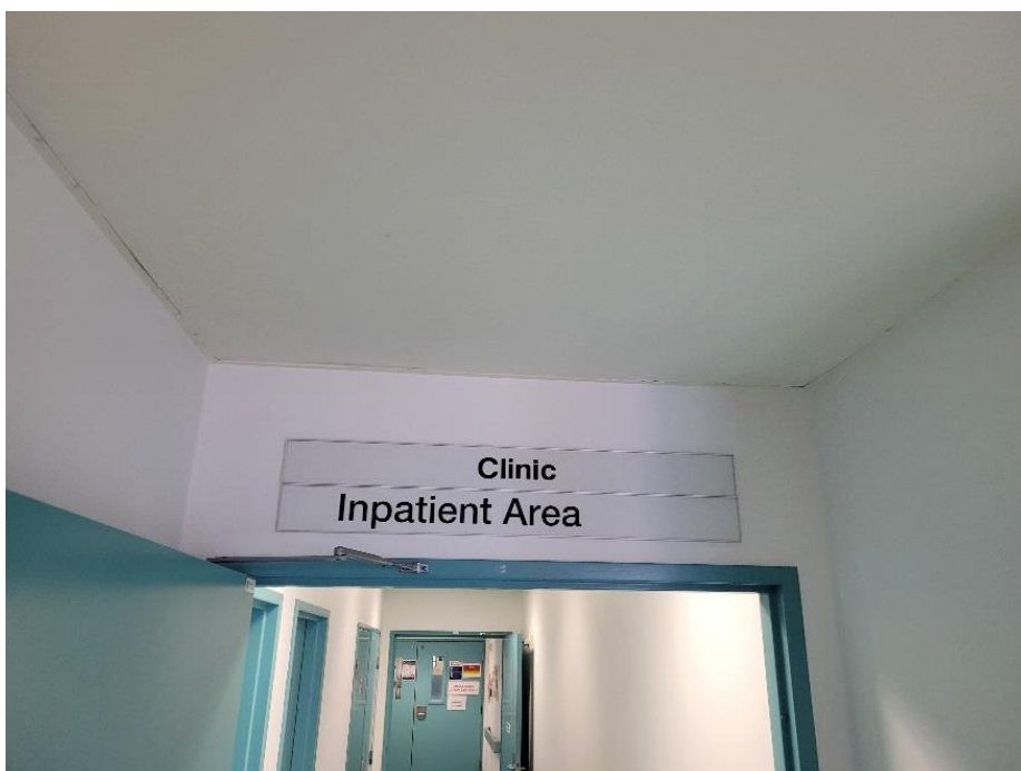
21. Crack in plasterboard at wall and ceiling junction
