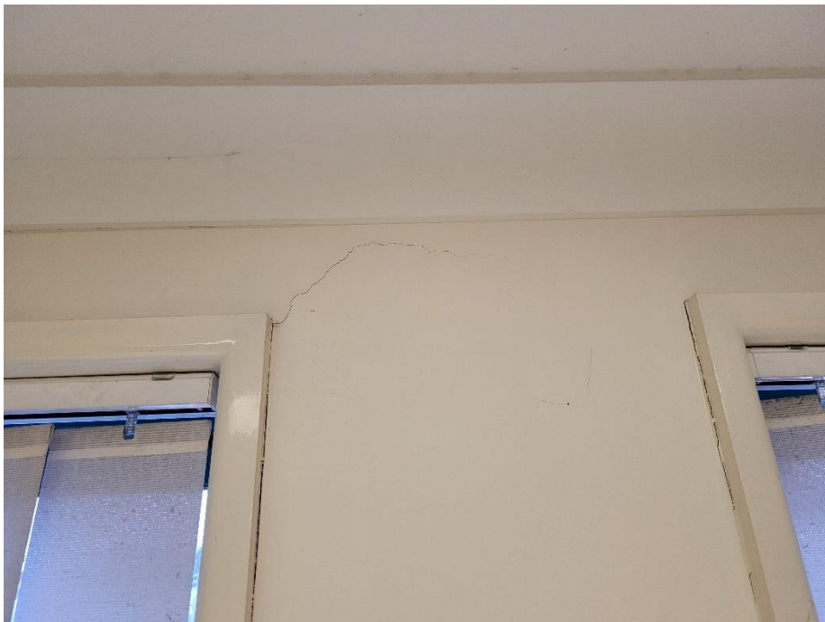
164. Cracking in plasterboard at wall and architrave around window opening to external wall
