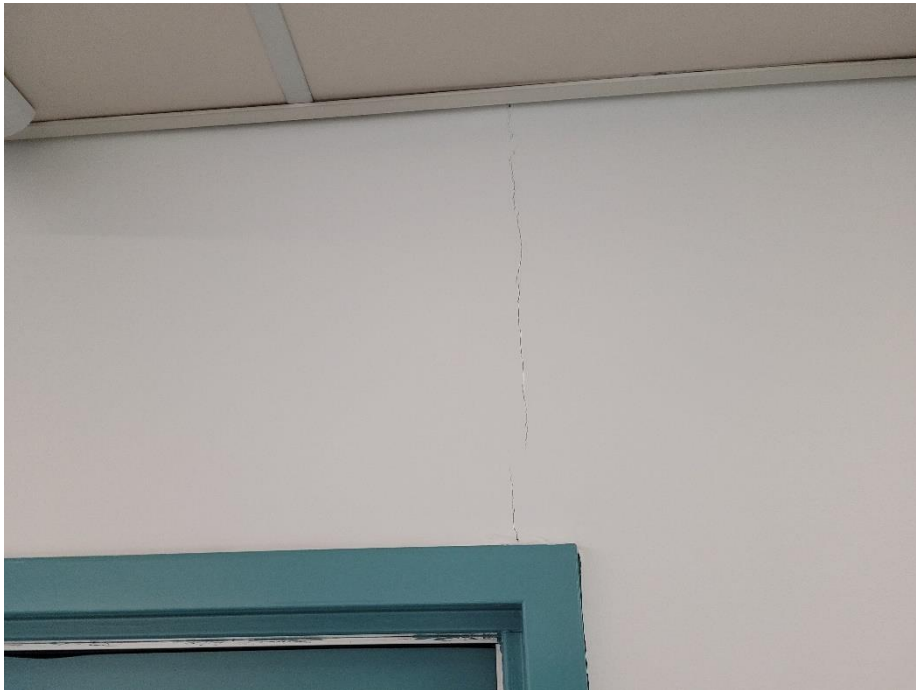
139. Vertical cracking in wall plasterboard from door frame to architrave
