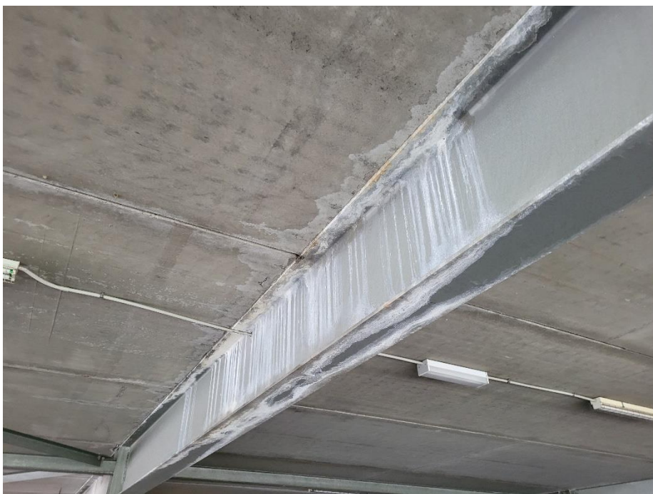
Existing Carpark 9. Water stains and potential surface corrosion to existing steel work
