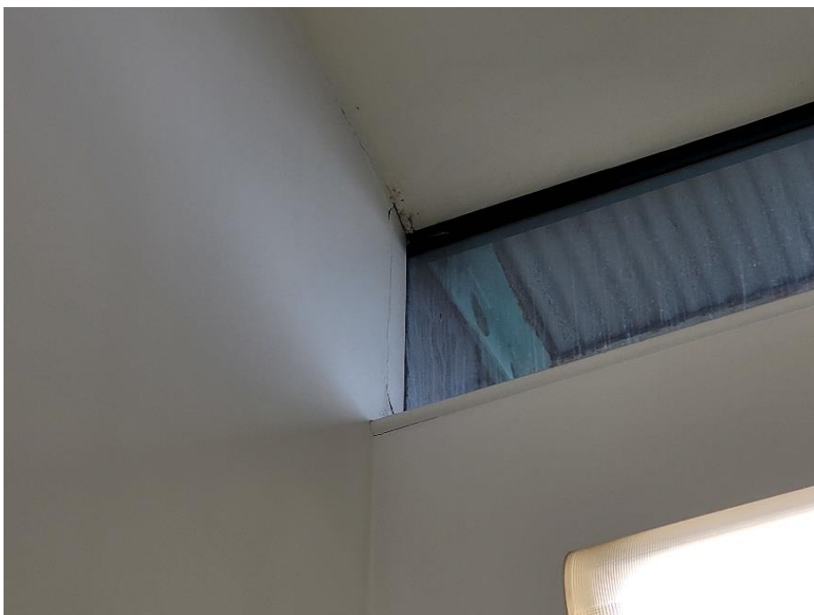
71. Cracking in plasterboard around window opening and water stains
