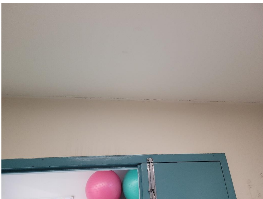
79. Crack in plasterboard at wall and ceiling junction
