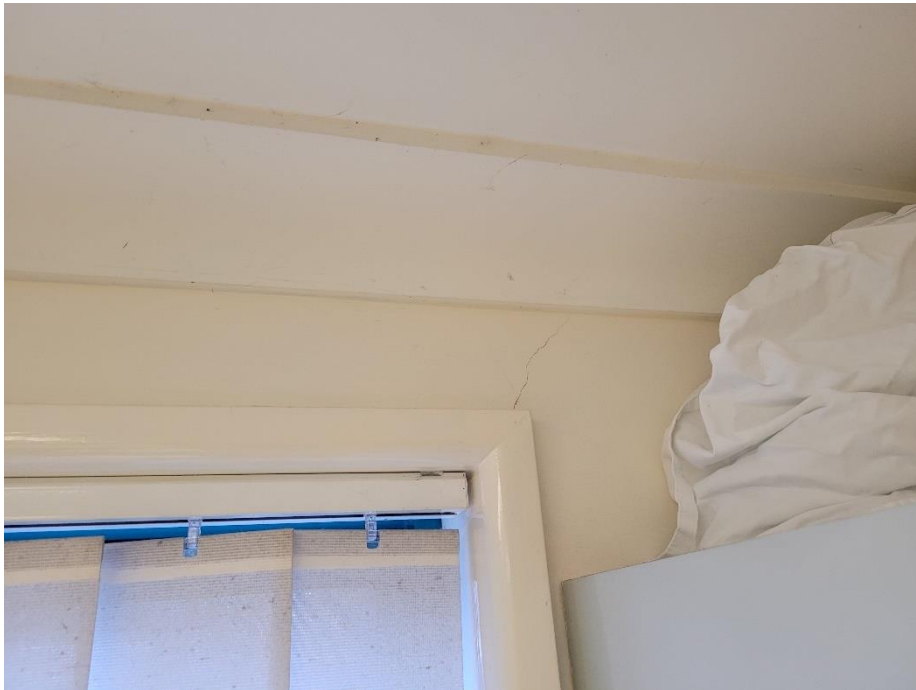
165. Cracking in plasterboard at wall and architrave around window opening to external wall
