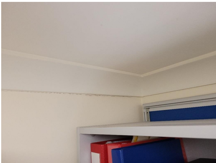
141. Crack in plasterboard at wall and architrave
