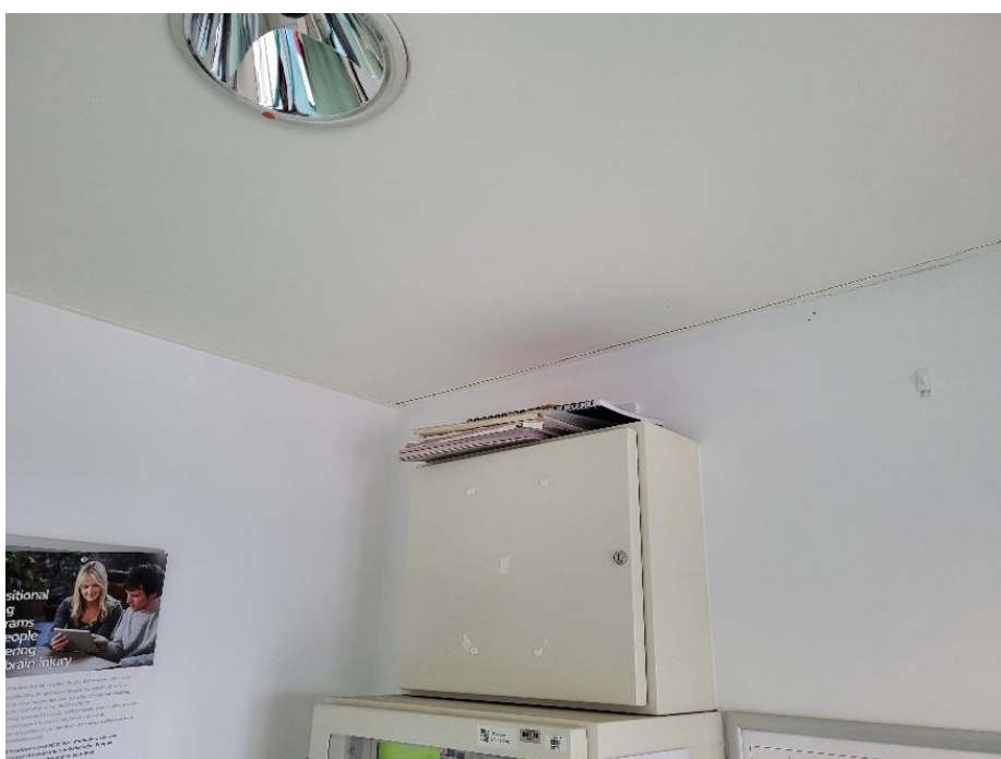
16. Crack in plasterboard at wall and ceiling junction
