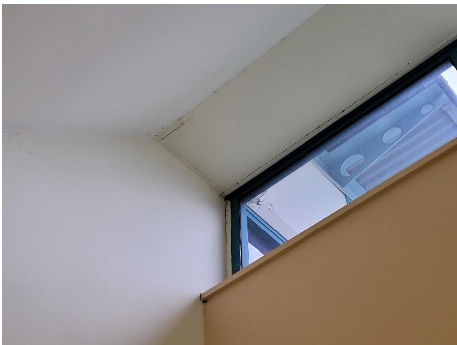
127. Crack in plasterboard at wall and ceiling junction, discolouring around window
