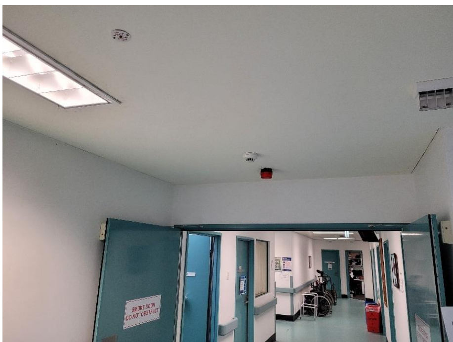
26. Crack in plasterboard at wall and ceiling junction around perimeter of door frame
