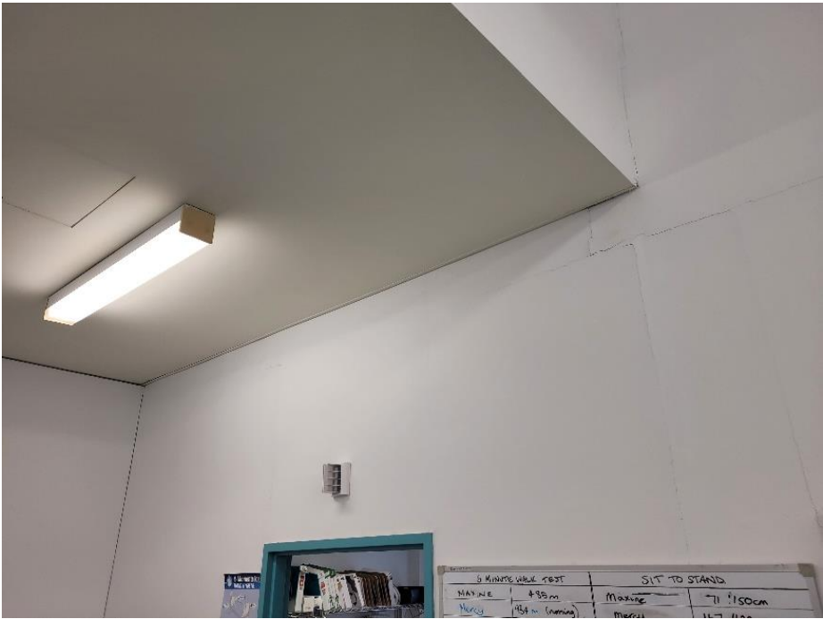
75. Extensive cracking to plasterboard around junction with ceiling, high wall section, lower wall section, light fitting, and external wall to lower ceiling
