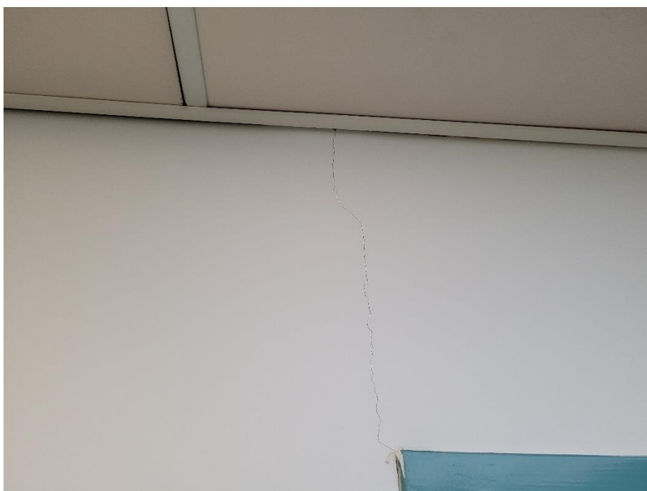
142. Vertical cracking in wall plasterboard from door frame to false ceiling
