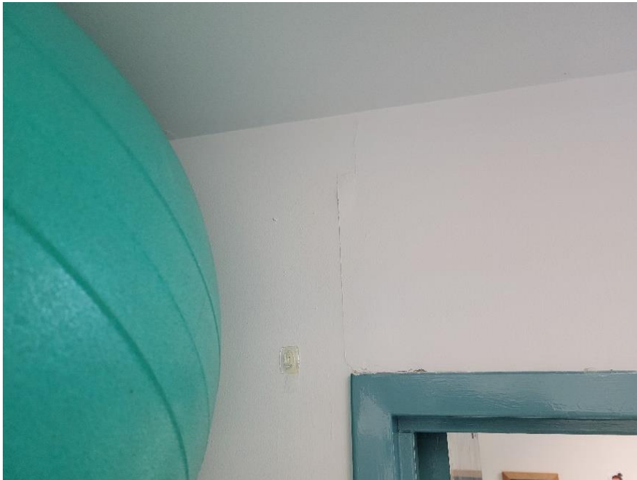
55. Vertical crack in plasterboard from door frame to ceiling
