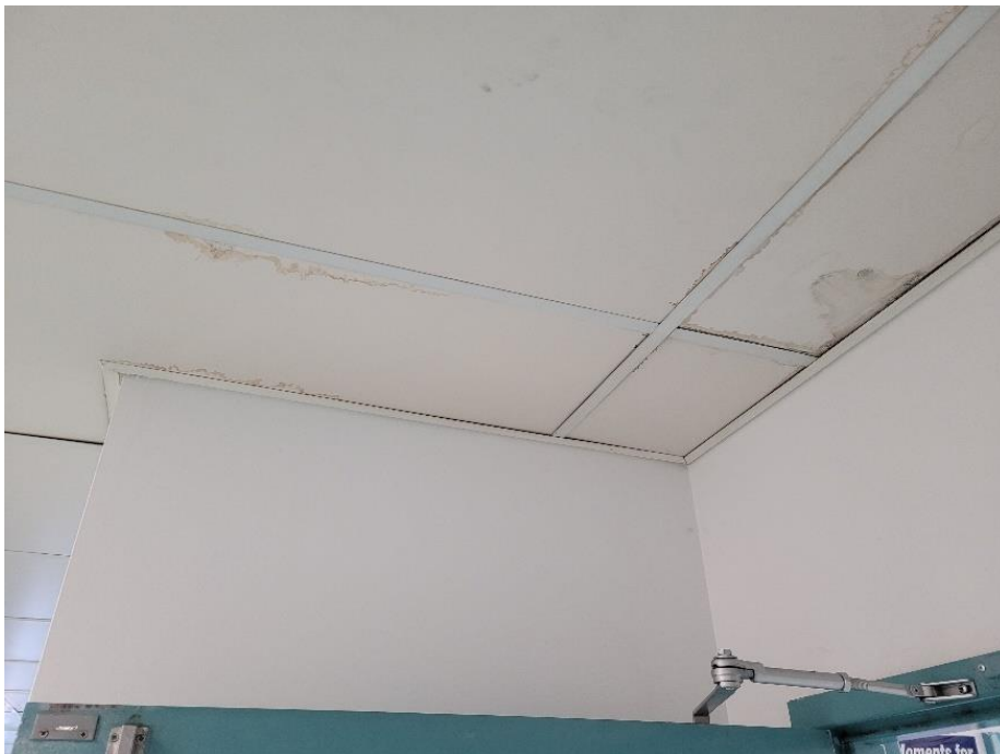
62. Water damage to false ceiling and cracks in plasterboard at wall and ceiling junction
