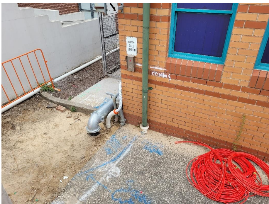
External 2. Cracking to masonry façade at corner and interface with slab on ground
