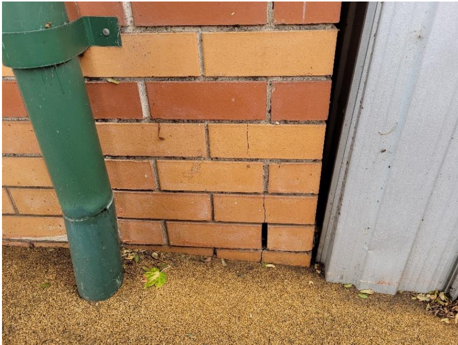
9. Cracks in brickwork
