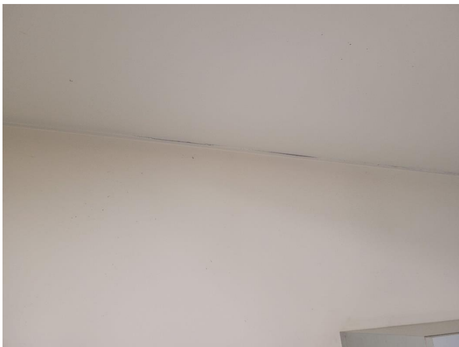
111. Crack in plasterboard at wall and ceiling junction
