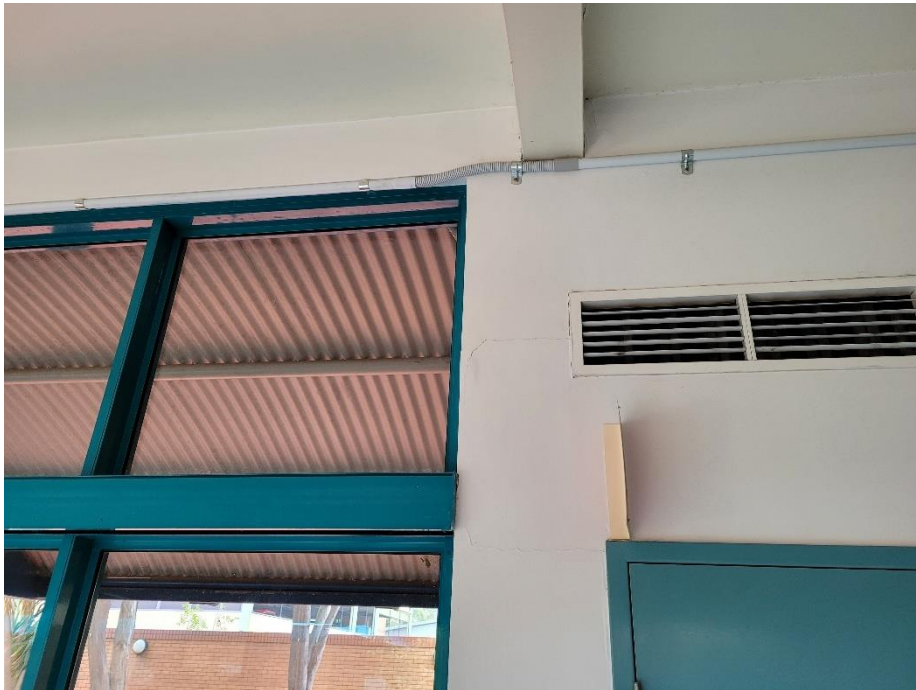
85. Cracking in plasterboard around vent opening
