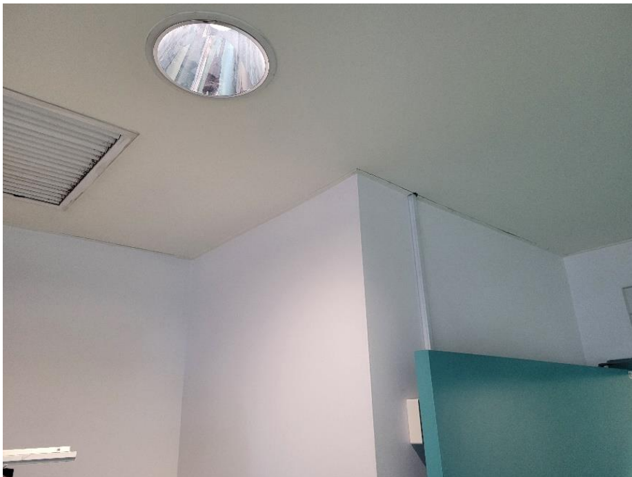
20. Crack in plasterboard at wall and ceiling junction
