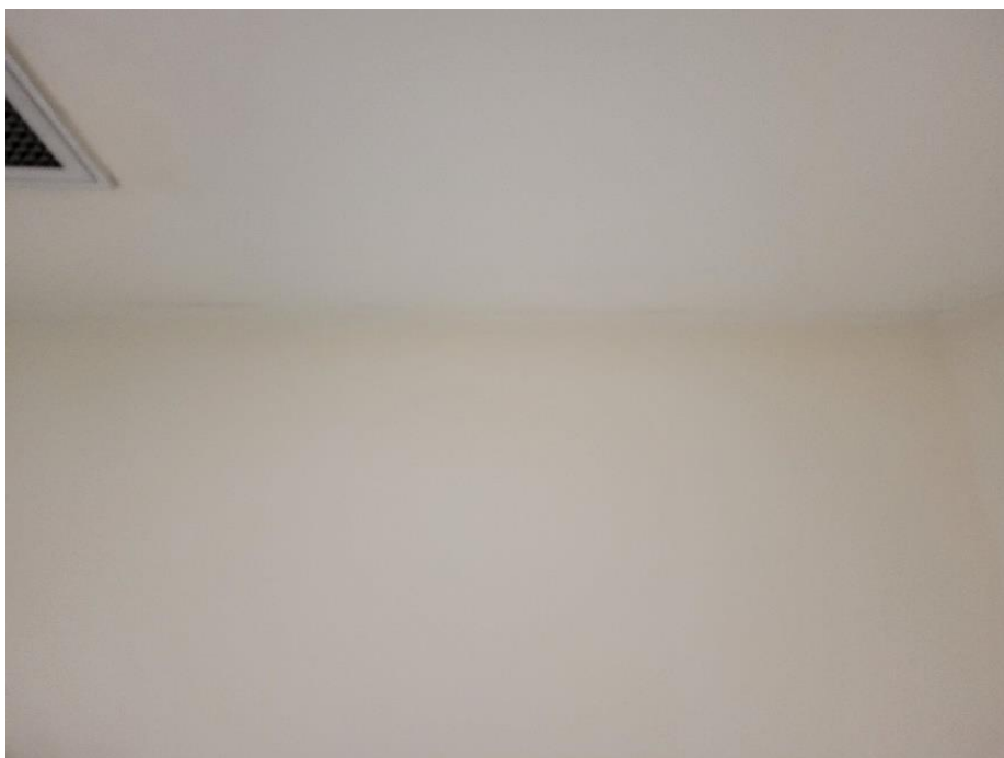
59. Crack in plasterboard at wall and ceiling junction
