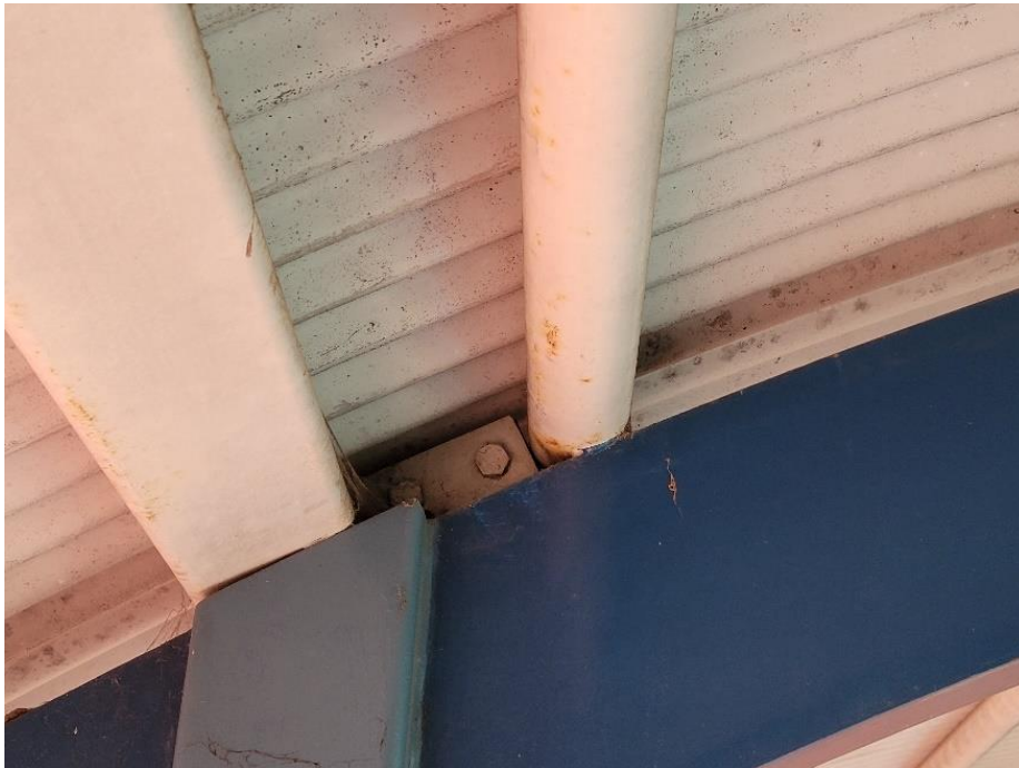
5. Surface rust and discolour
