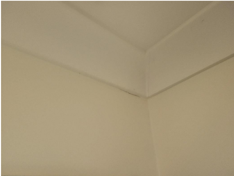
121. Crack in plasterboard around architrave
