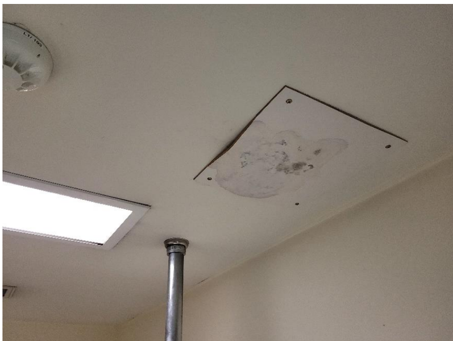
66. Water stains to ceiling path and damage to patch plate, crack in plasterboard at wall and ceiling junction
