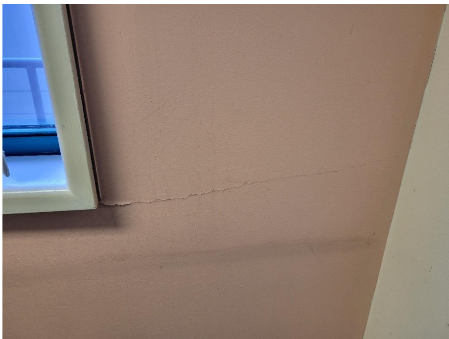
157. Horizontal crack in plasterboard from window opening to corner on external wall
