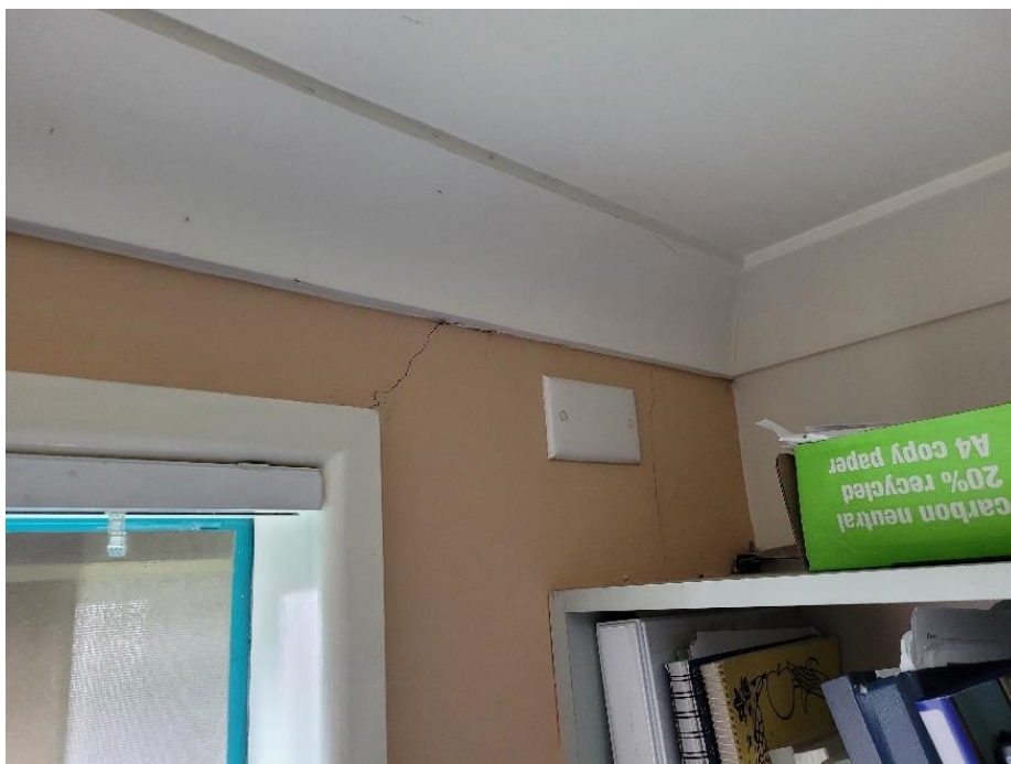
39. Cracking in plasterboard on external wall around window and vertical crack in corner, partially concealed behind furniture
