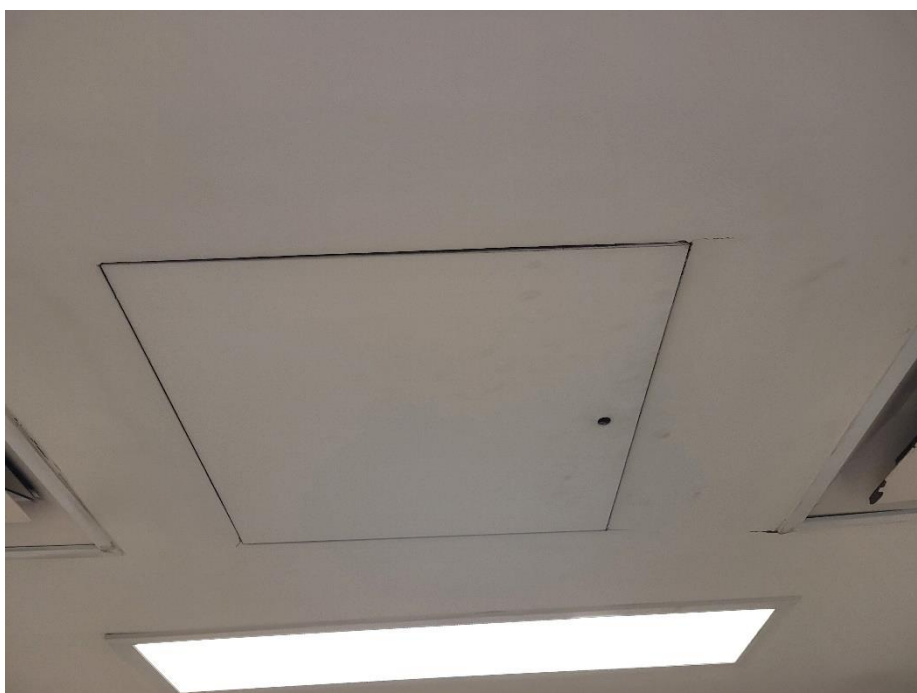
168. Cracking in ceiling around access panel, signs of discolouring
