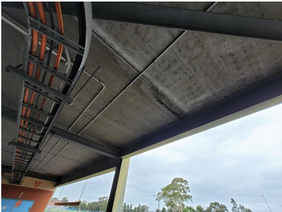
Existing Carpark 4. Cracks to soffit of first floor slab
