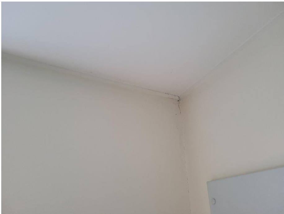
28. Crack in plasterboard at wall and ceiling junction
