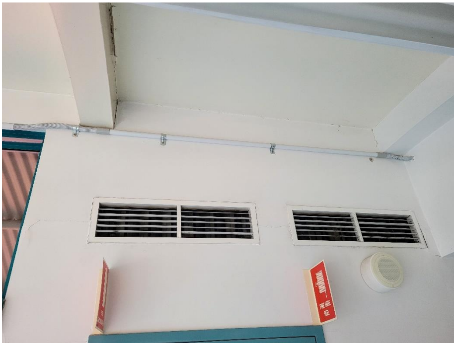
84. Crack in plasterboard at wall and ceiling junction
