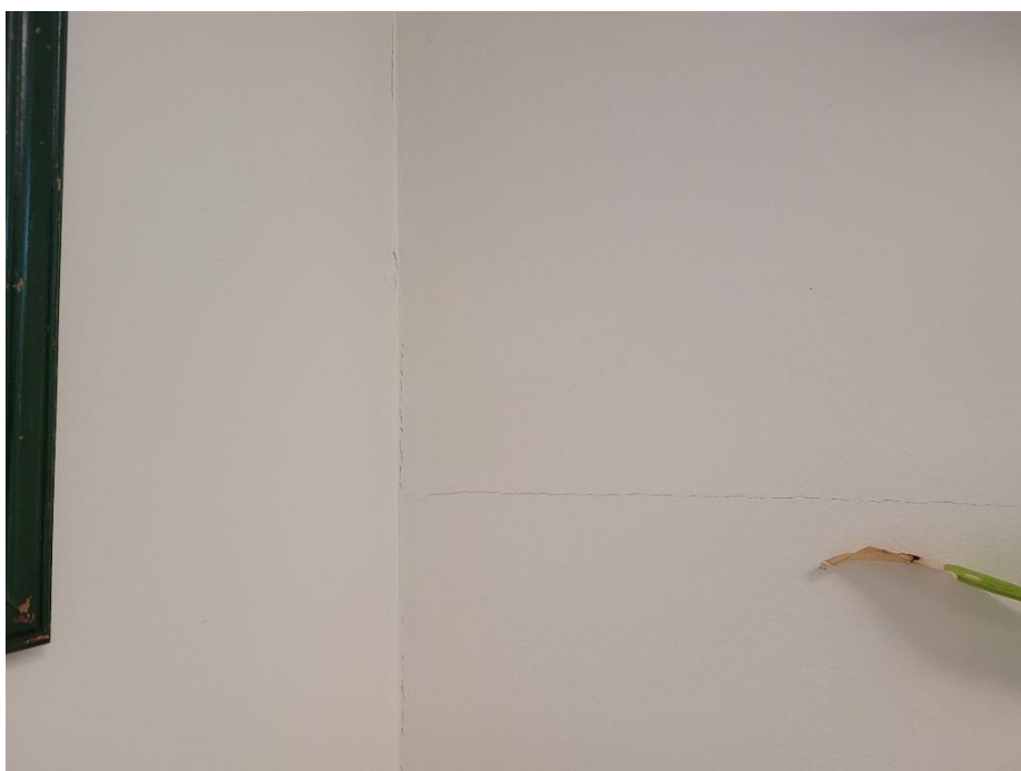
146. Horizontal cracking in plasterboard
