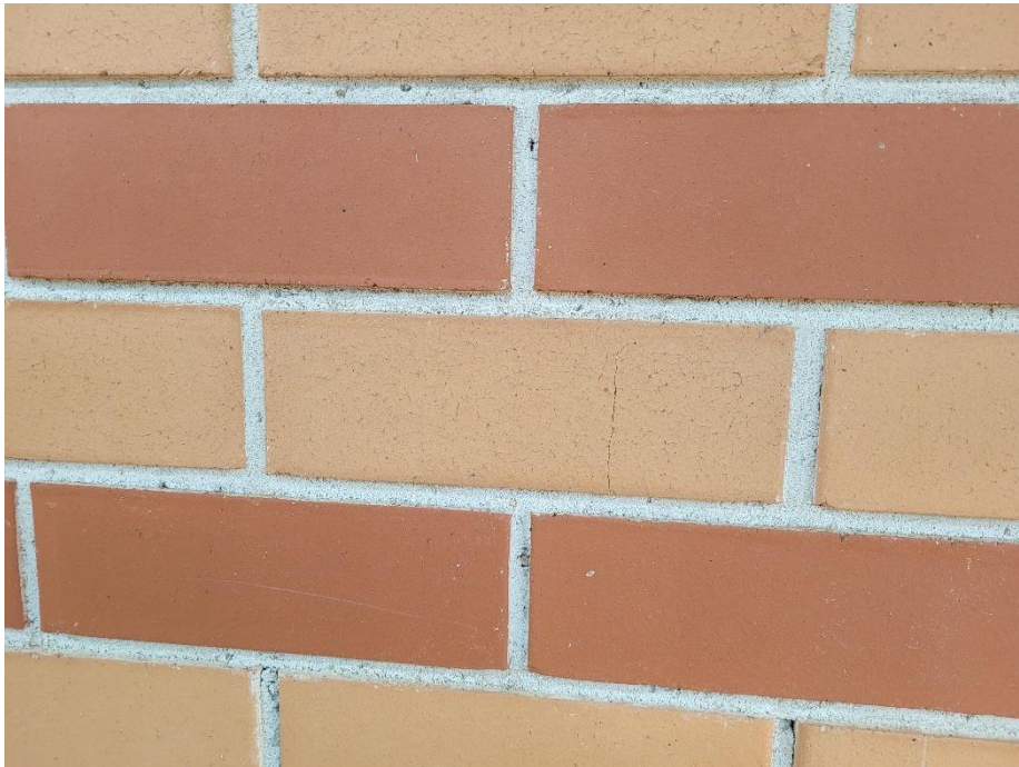
177. Minor cracking in external masonry wall
