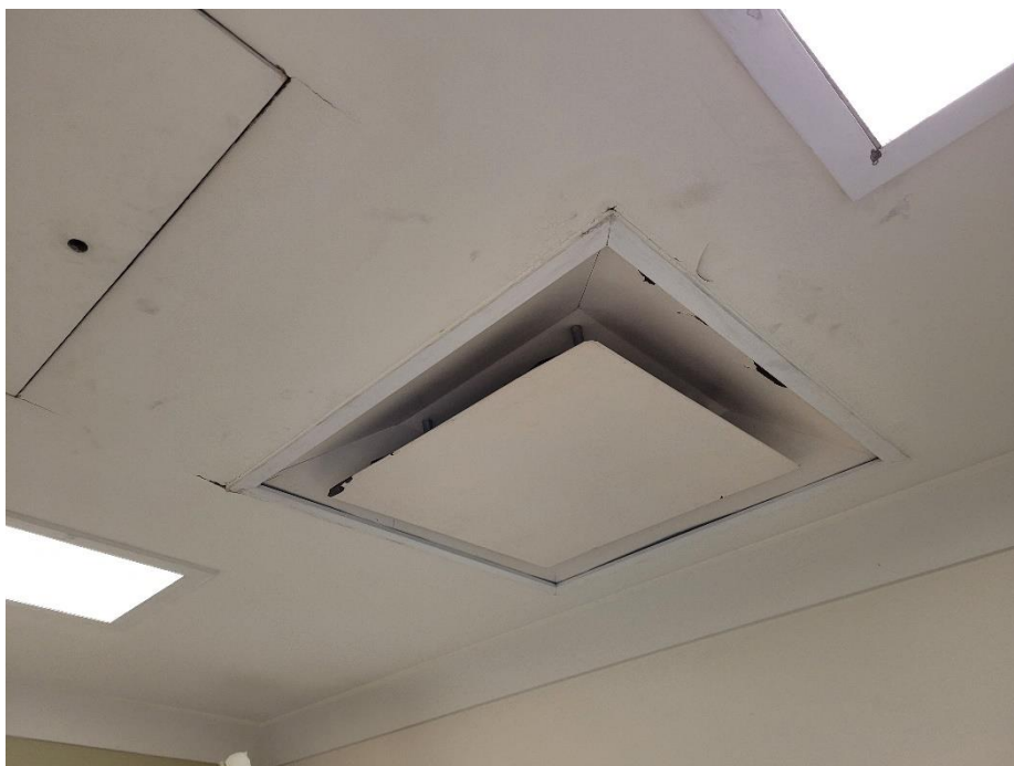
167. Cracking in ceiling around light fitting, signs of discolouring
