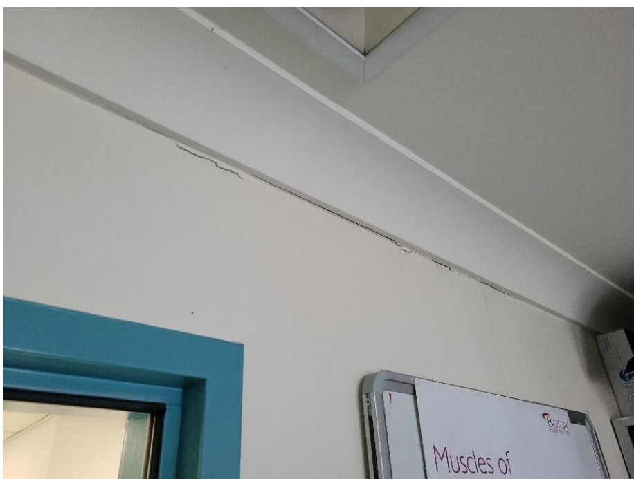
38. Crack in plasterboard at wall and ceiling junction
