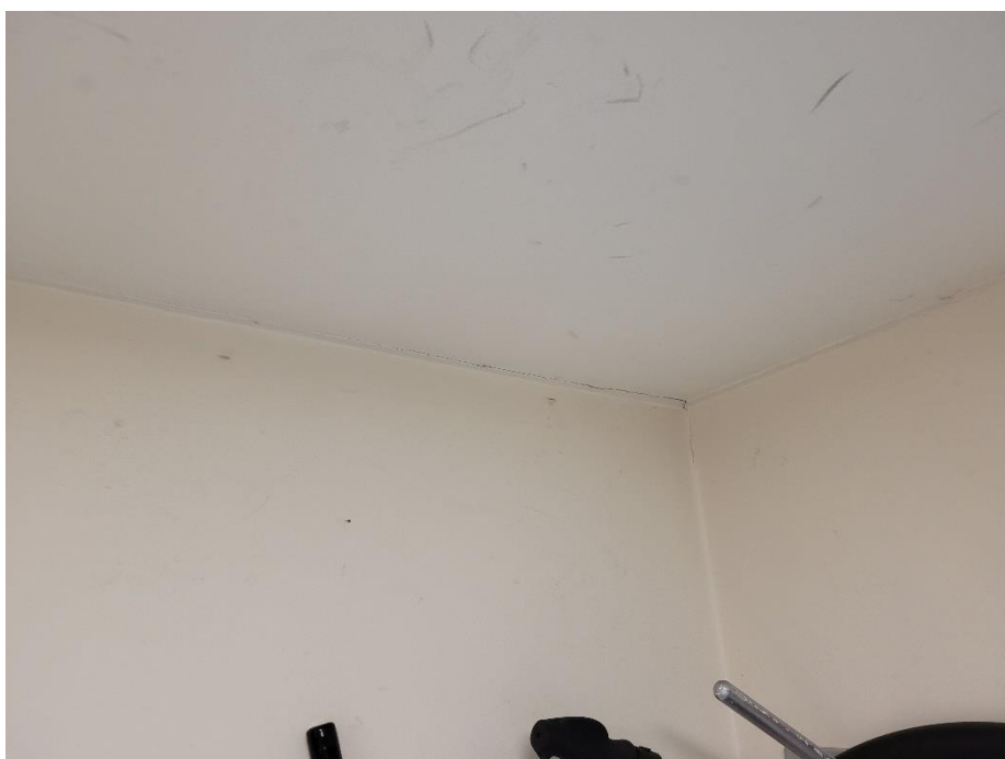
78. Crack in plasterboard at wall and ceiling junction
