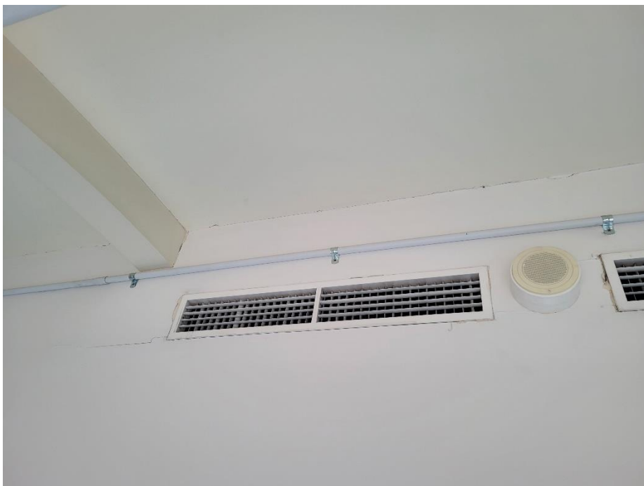
90. Crack in plasterboard at wall and ceiling junction, cracking around vent opening
