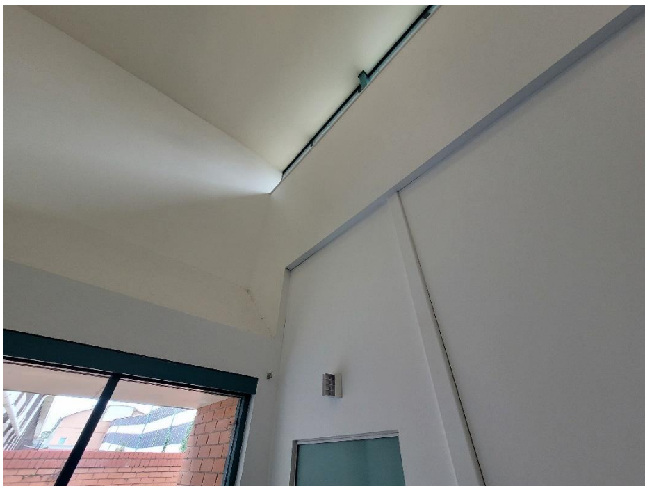
98. Cracking in plasterboard at various locations across wall junction
