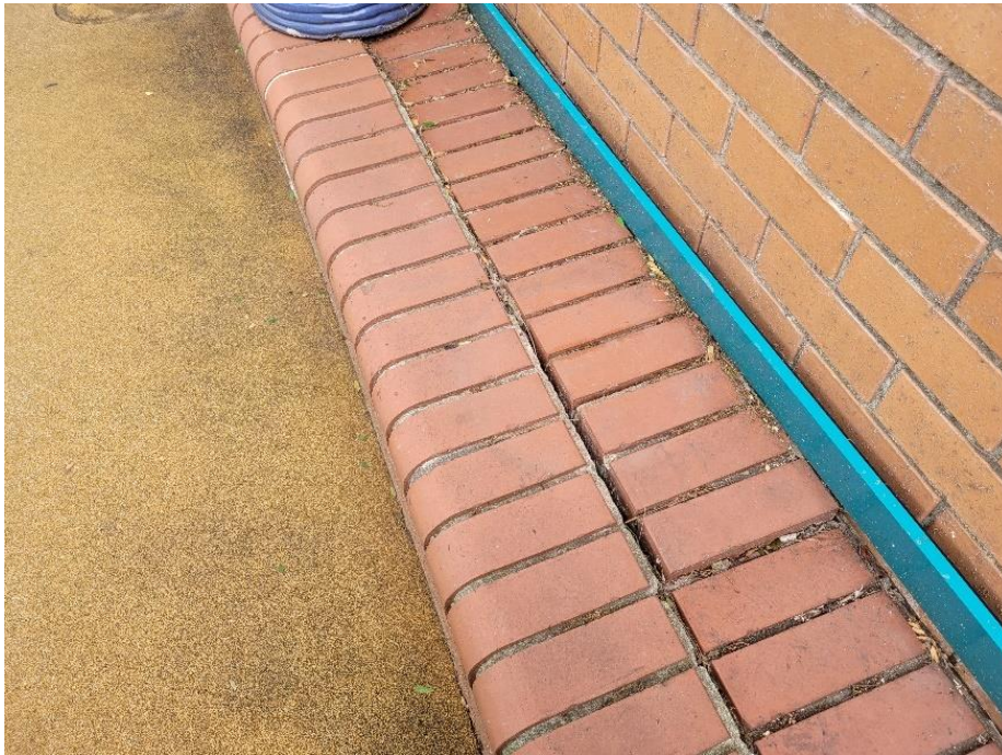
13. Brickwork damage, gap between courses
