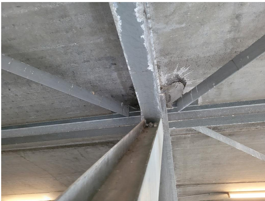
Existing Carpark 10. Water stains and potential surface corrosion to existing steel work
