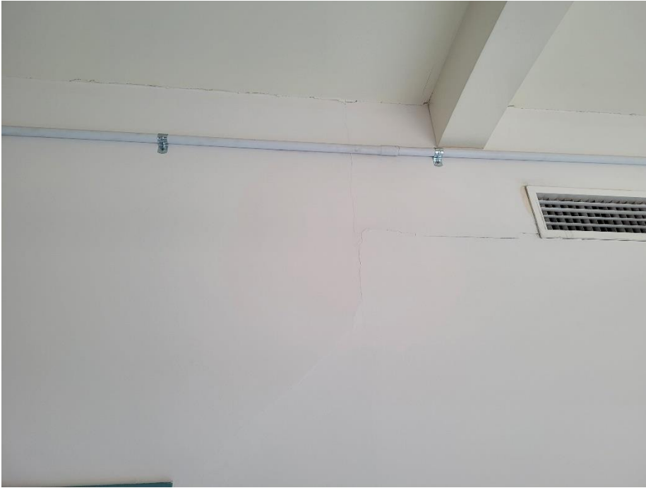
91. Crack in plasterboard at wall and ceiling junction
