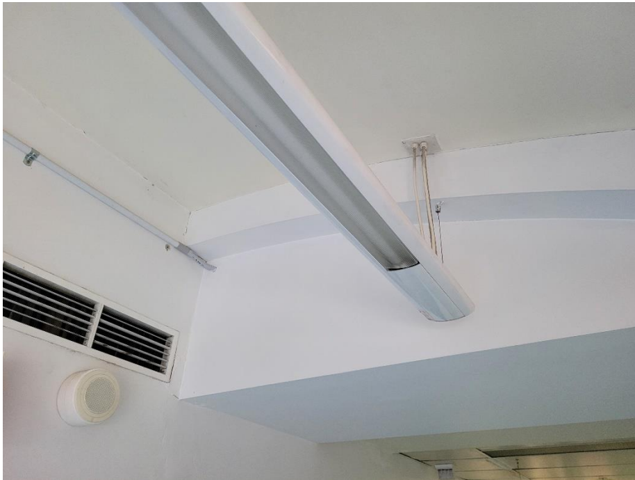
83. Crack in plasterboard at wall and ceiling junction
