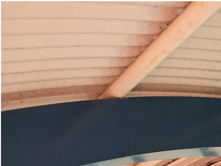
6. Surface rust and discolour
