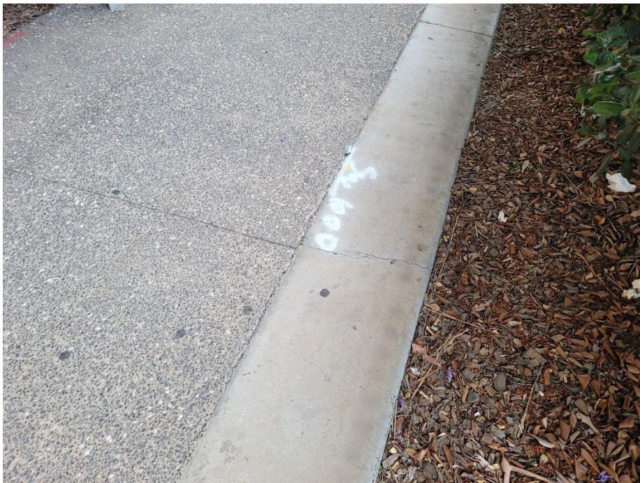
External 6a. Crack in kerb along walkway
