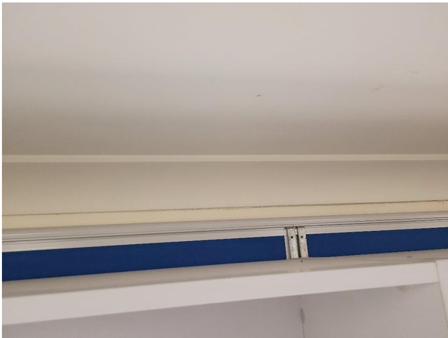
140. Crack in plasterboard at wall and architrave
