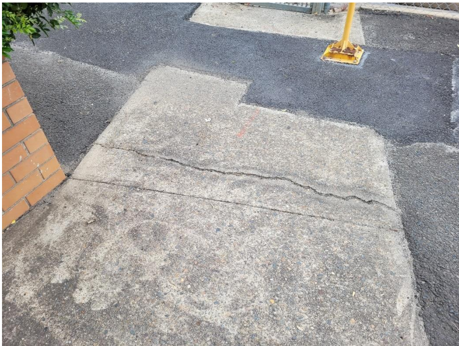
External 10. Cracking in footpath
