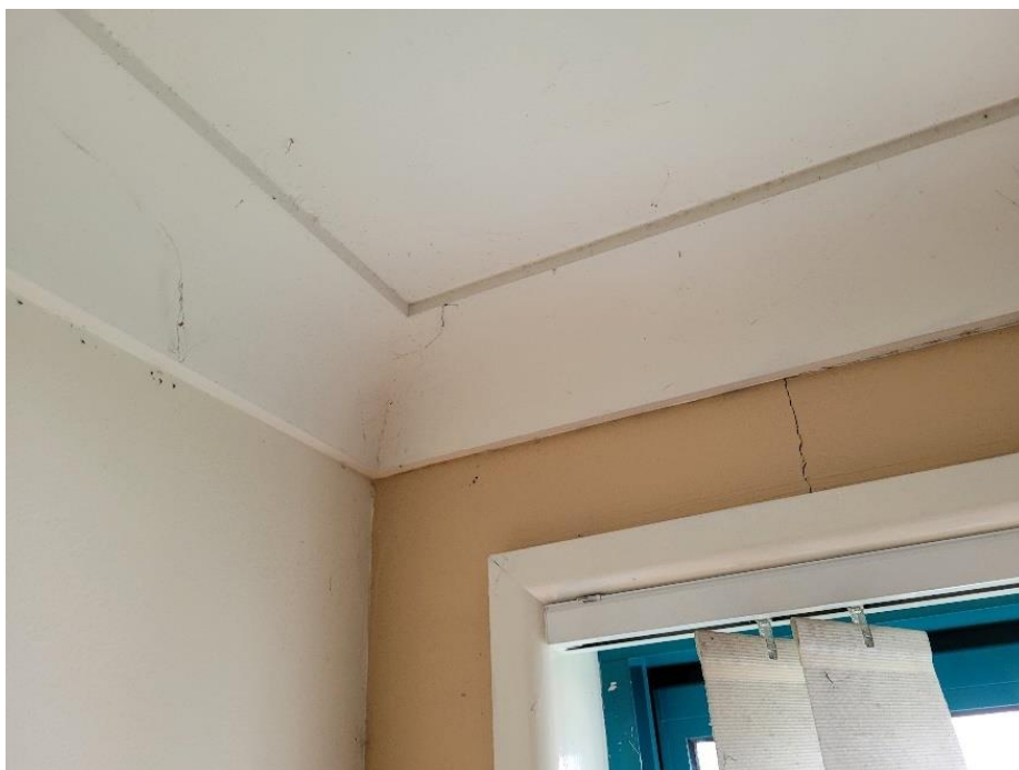
33. Vertical crack in plasterboard on external wall around window
