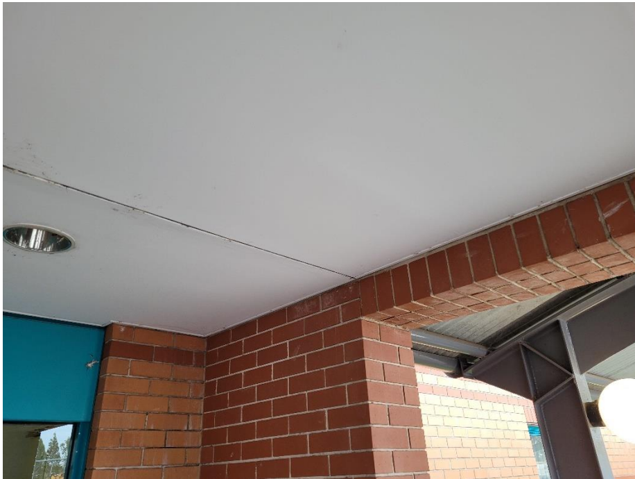
External 7. Damage and staining to external entrance way ceiling
