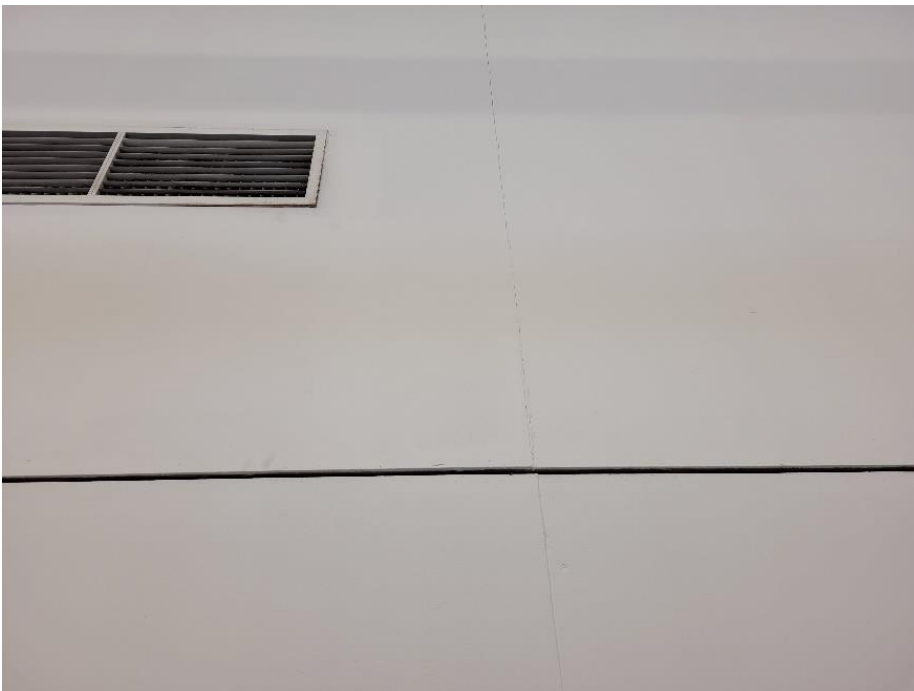
68. Vertical cracking from lower wall section to upper wall section, across shadow gap
