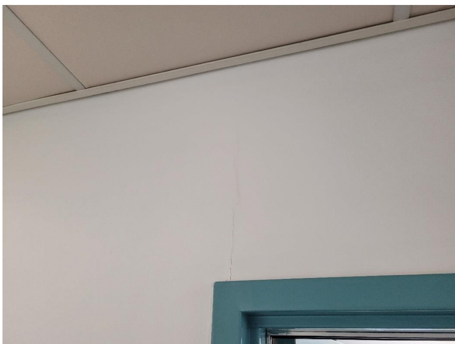
144. Vertical cracking in wall plasterboard from door frame to false ceiling
