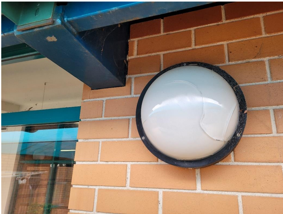
178. Damage to external light fitting
