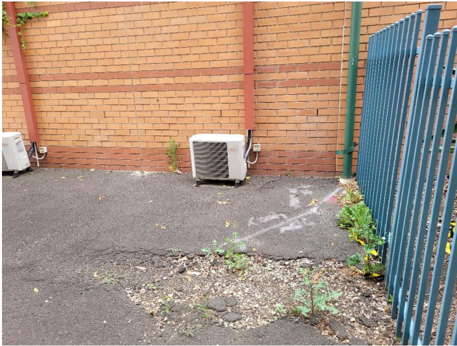
External 19. Damage to external ground bituminous layer, general cracking, and damage across building bounds.
