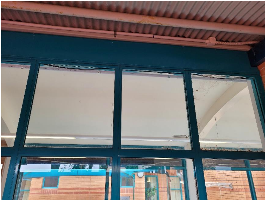
7. Window seals damaged
