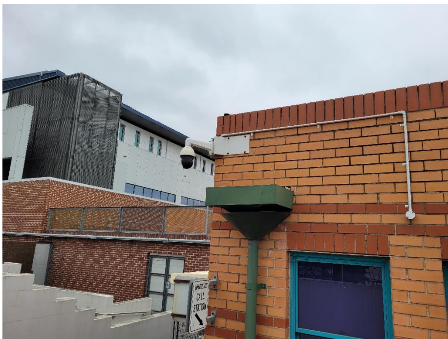
External 1. Cracking around parapet junction and opening for water outlet
