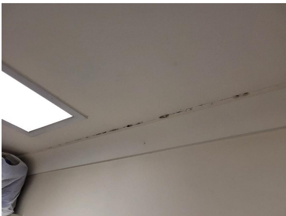
40. Crack in plasterboard ceiling at architrave edge
