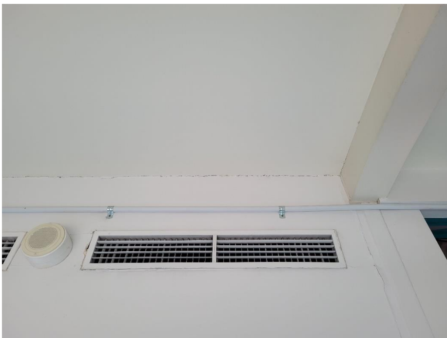
89. Crack in plasterboard at wall and ceiling junction, cracking around vent opening
