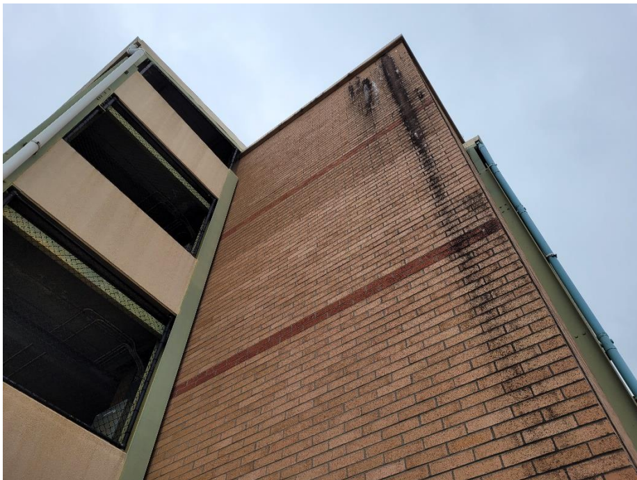
Existing Carpark 6. Staining to core structure
