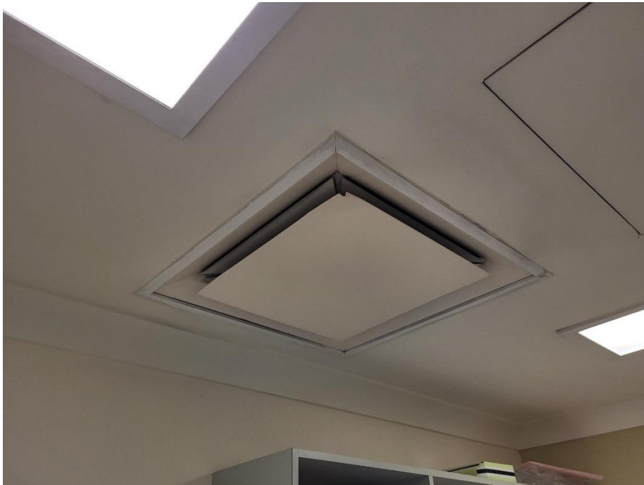
169. Cracking in ceiling around light fitting, signs of discolouring
