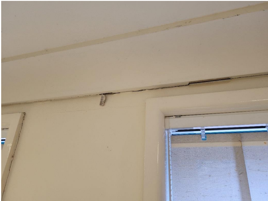
149. Crack in plasterboard at wall and architrave to external wall
