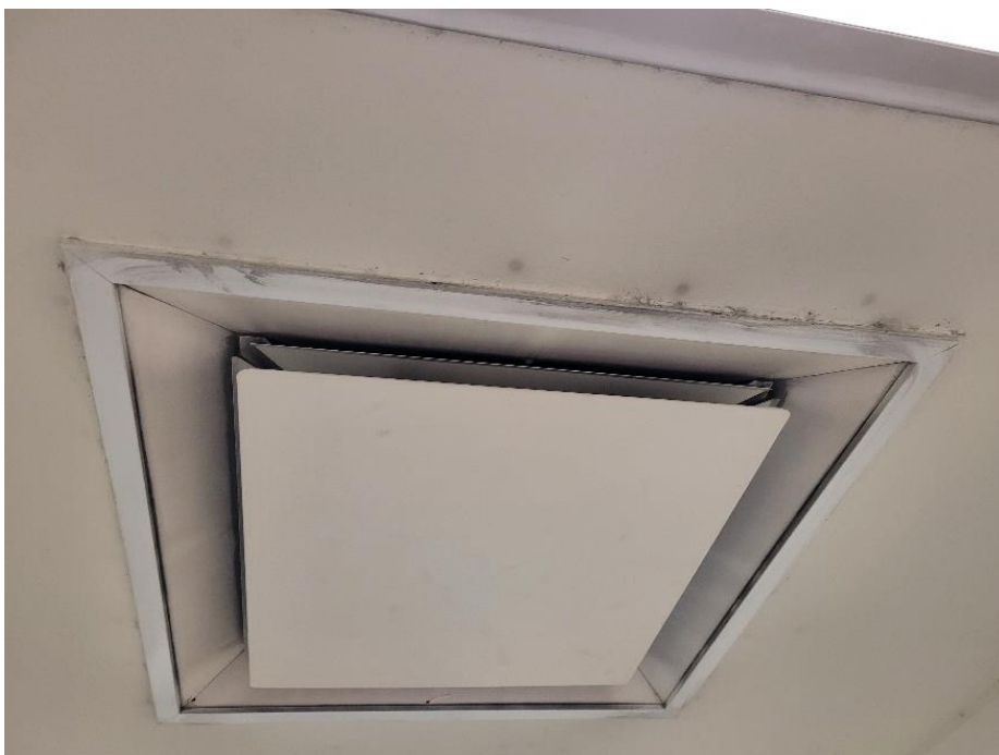
41. Discolouring around vent frame
