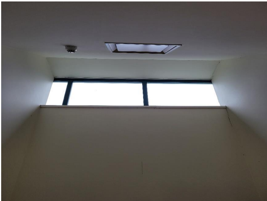
32. Crack in plasterboard around window
