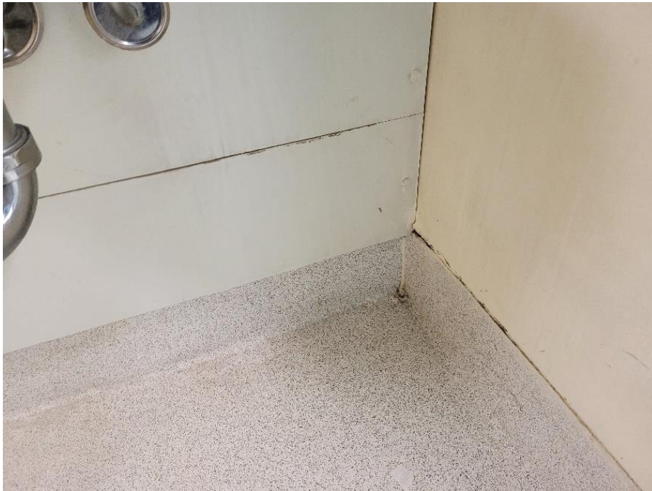
64. discolouration around floor finish and wall junction
