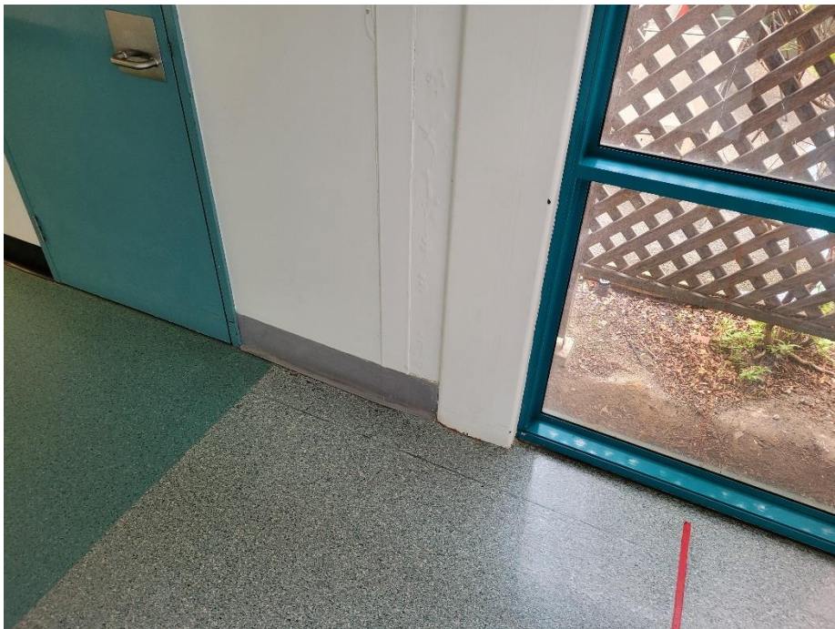
82. Cracking to plasterboard, water damage to wall finish, discolouration and staining to junction with floor finish.
