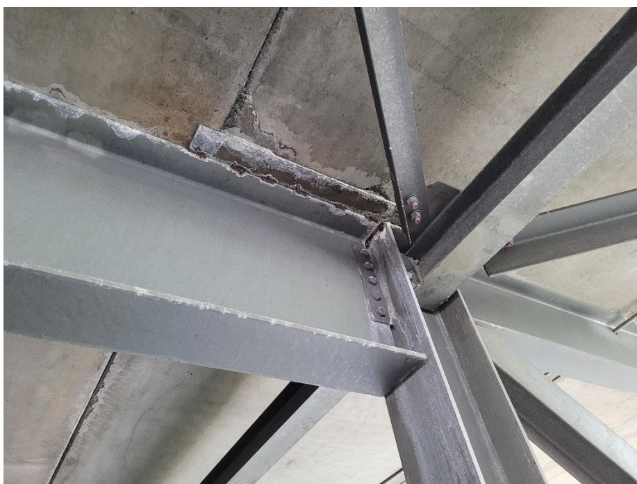
Existing Carpark 8. Water stains and potential surface corrosion to existing steel work
