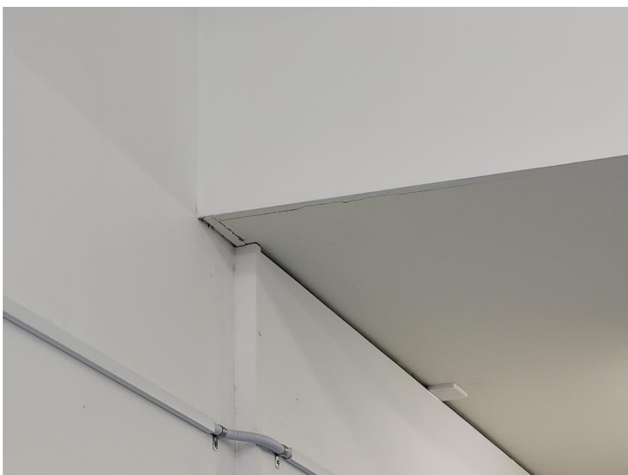
72. Cracking to various plasterboard junctions and wall joint
