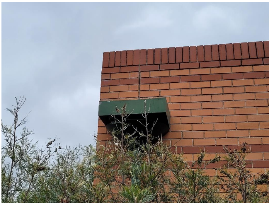
External 11. Cracking to parapet masonry and around water outlet
