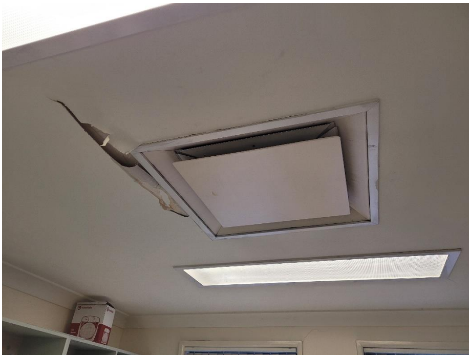
163. Damage to ceiling finishes around vent opening
