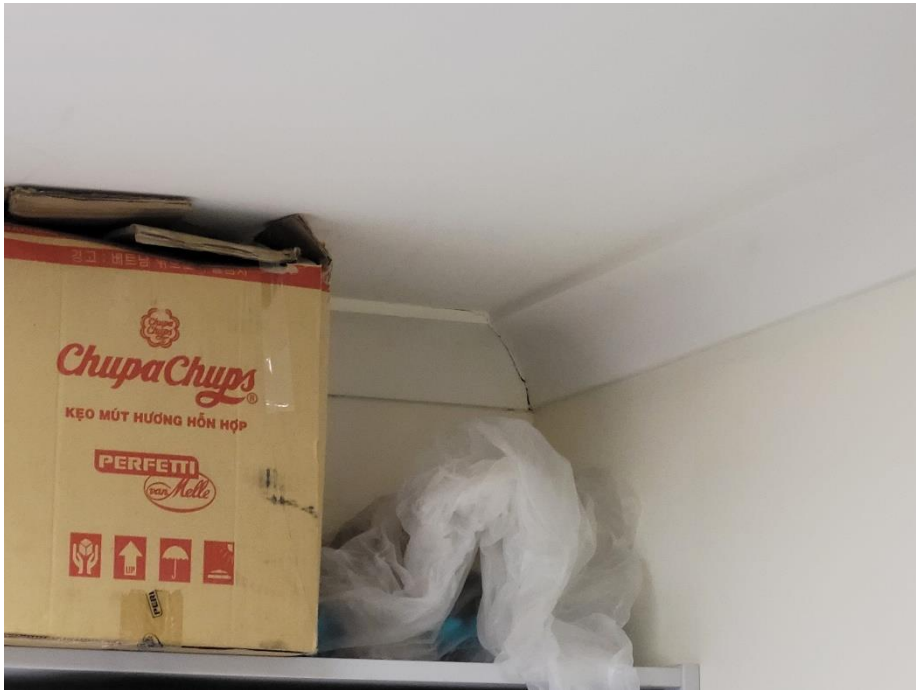
153. Crack in plasterboard at wall and architrave
