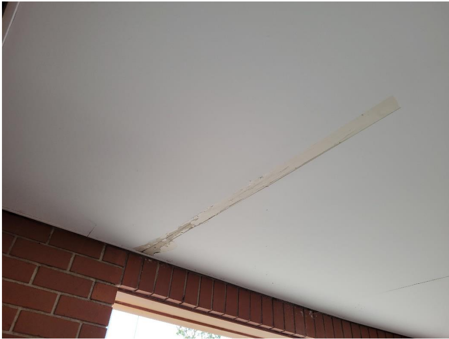
External 5. Damage and staining to external entrance way ceiling
