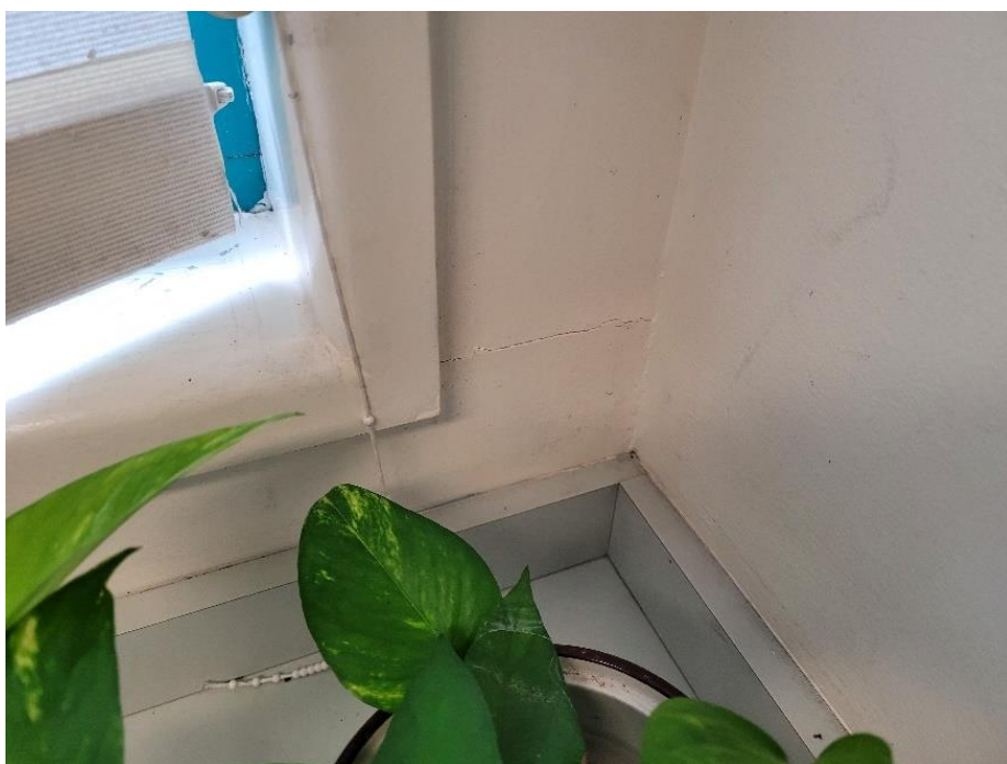
36. Horizontal cracks in plasterboard on external wall around window
