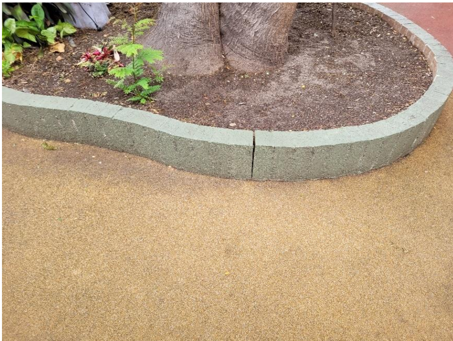
10. Garden bed brickwork damage
