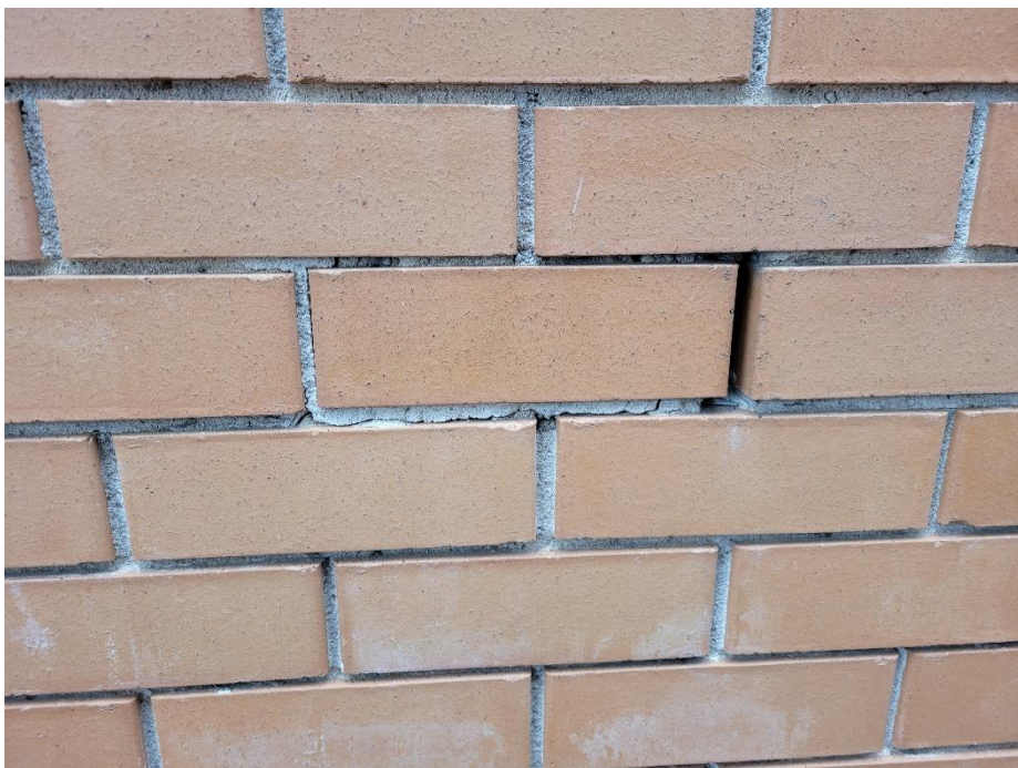
External 18. Cracking to mortar and mortar loss for external wall
