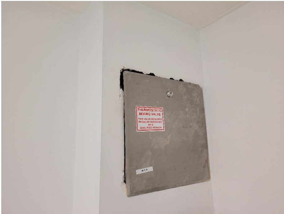
133. Wall cover plate loose in fitting
