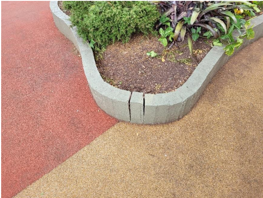
11. Garden bed brickwork damage
