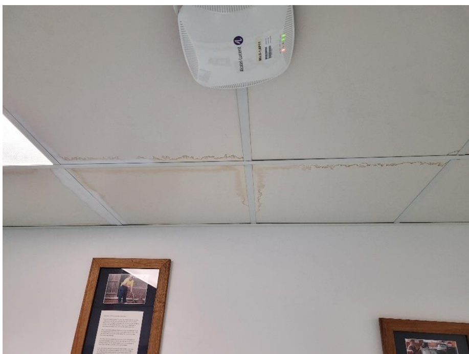
50. Water damage to false ceiling
