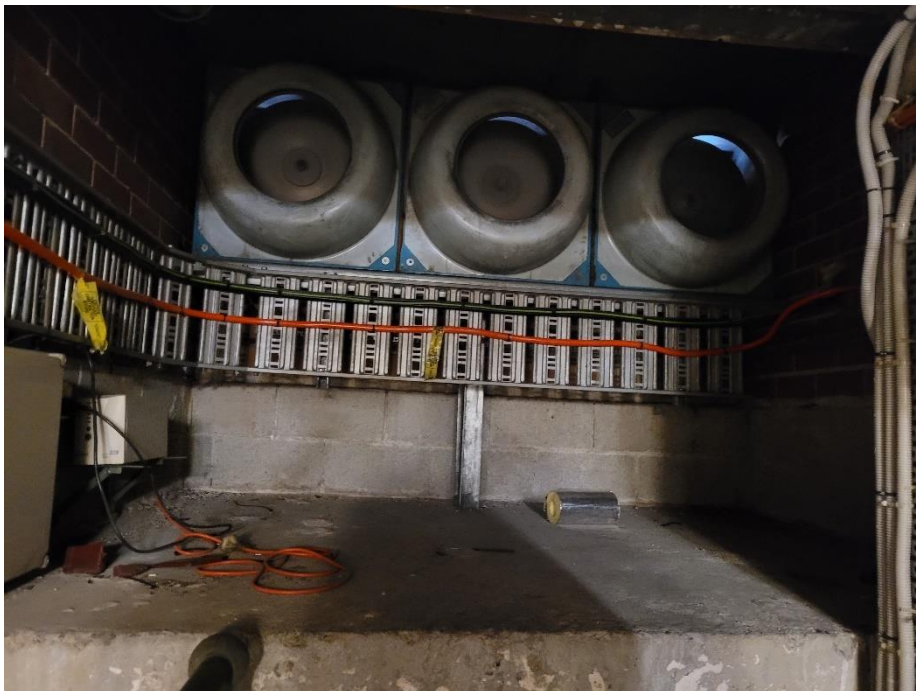
Service Tunnel 3. Air vent access point, general minor damage to concrete edges
