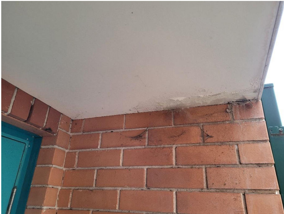
115. Water damage to eave soffit and cracking in masonry for external wall
