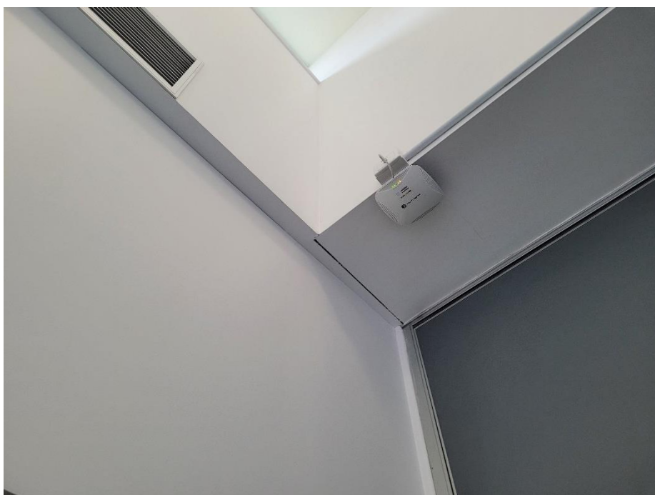
99. Crack in plasterboard at wall and ceiling junction
