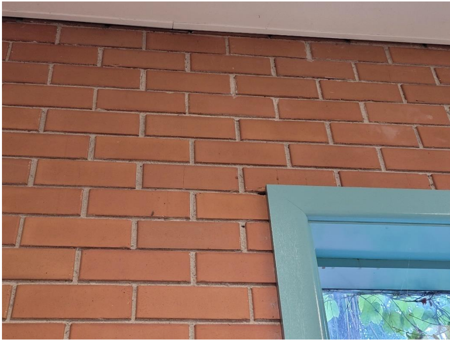
103. Cracking to bricks and across mortar joints in external wall
