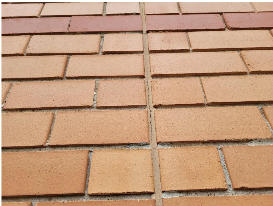
External 13. Cracking in mortar and vertical cracks/sign of wear in building joint
