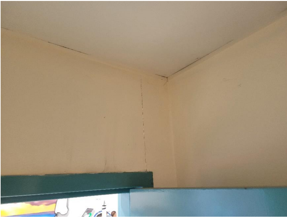
67a. Crack in plasterboard at wall and ceiling junction and vertical cracking above doorway
