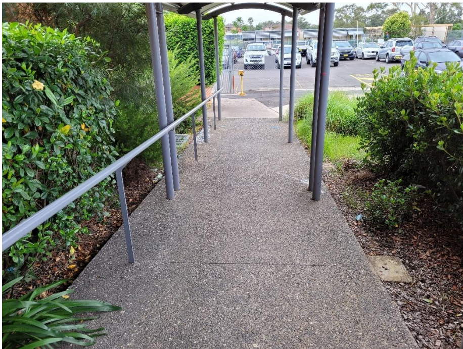
External 8a. General wear and tear of walkway, various minor cracks, and damage to edge along gardens
