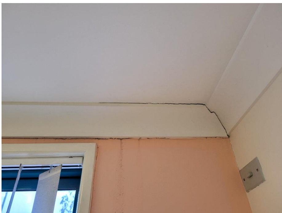
158. Crack in plasterboard at wall and architrave
