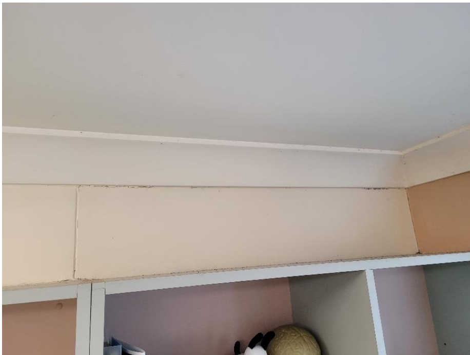
46. Crack in plasterboard at wall and ceiling junction
