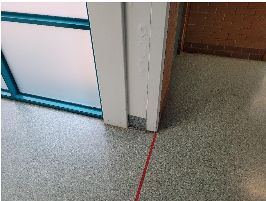
95. Water damage to wall and discolouring at junction with floor finish
