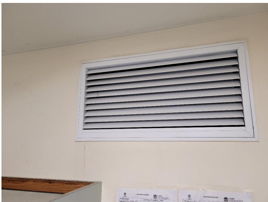
112. Cracking in wall plasterboard around vent opening
