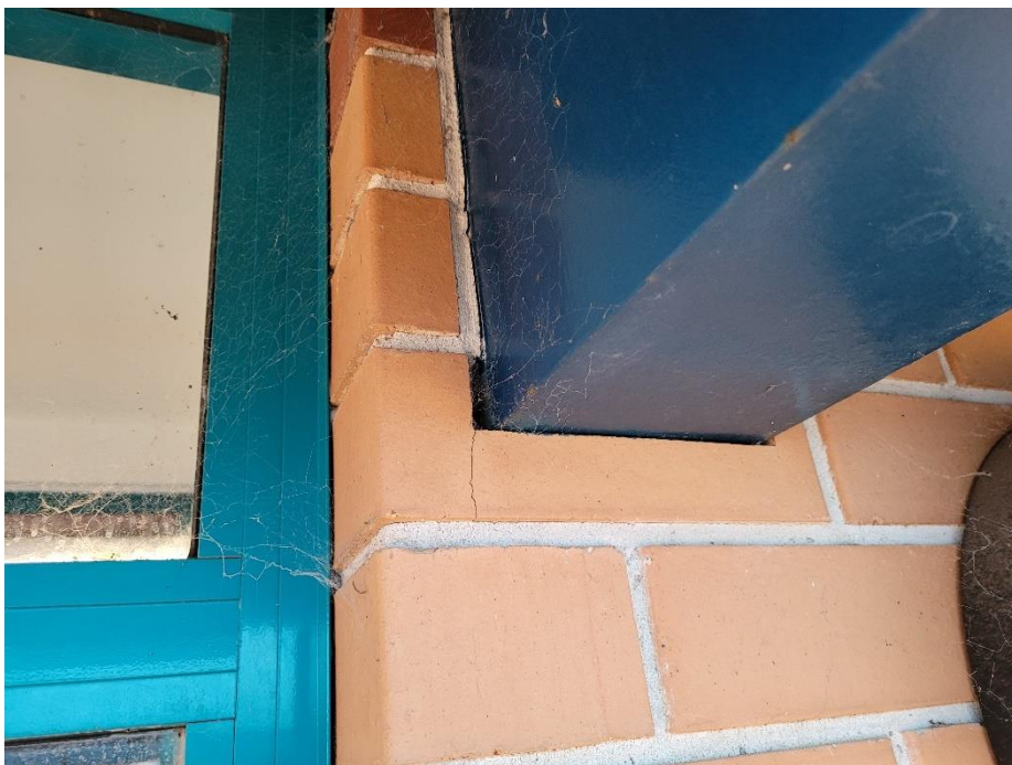
176. Cracking in external masonry around steel member penetration
