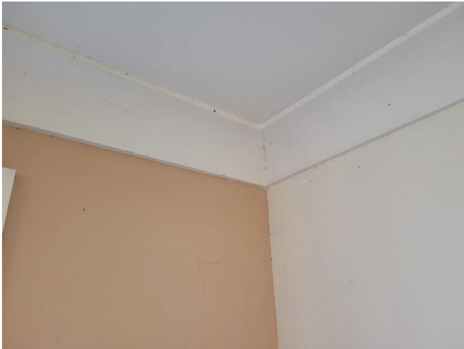
45. Crack in plasterboard at wall and ceiling junction
