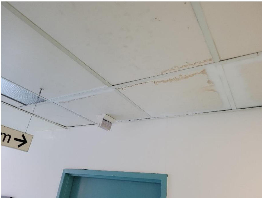
52. Water damage to false ceiling
