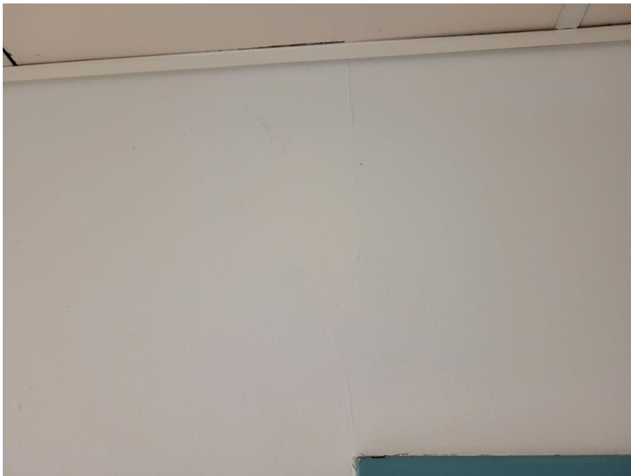
120. Vertical cracking from top of door frame to false ceiling
