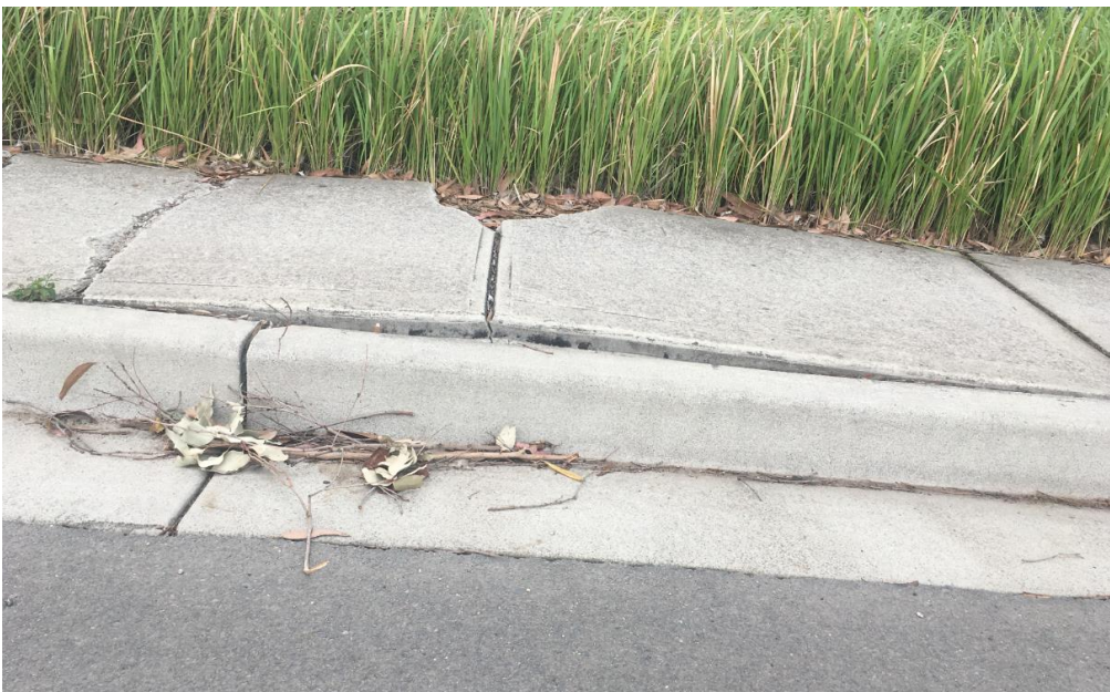
Burnside Drive 10. Footpath deformation
