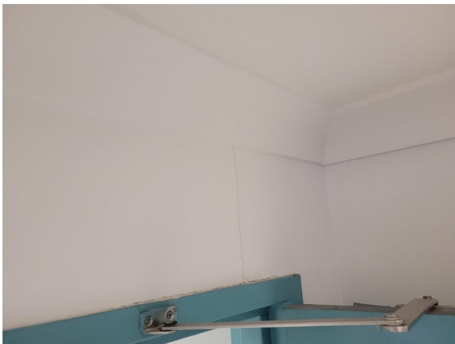
123. Vertical cracking from door frame to architrave
