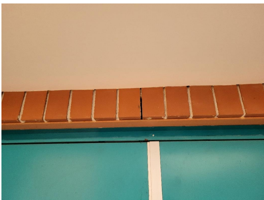
114. Minor cracking to mortar and gaps between soffit and external masonry
