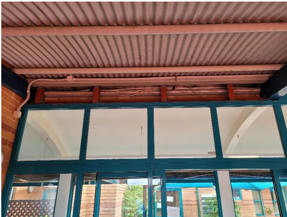
4. Faced panel missing
