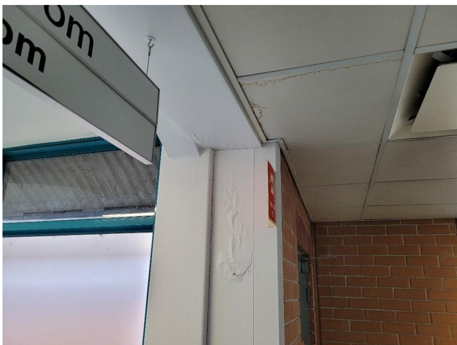
93. Crack in plasterboard at wall and ceiling junction, water damage to wall and false ceiling
