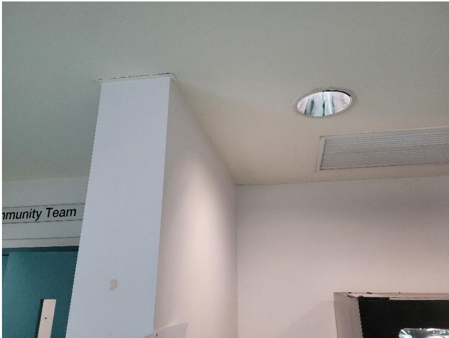
19. Crack in plasterboard at wall and ceiling junction
