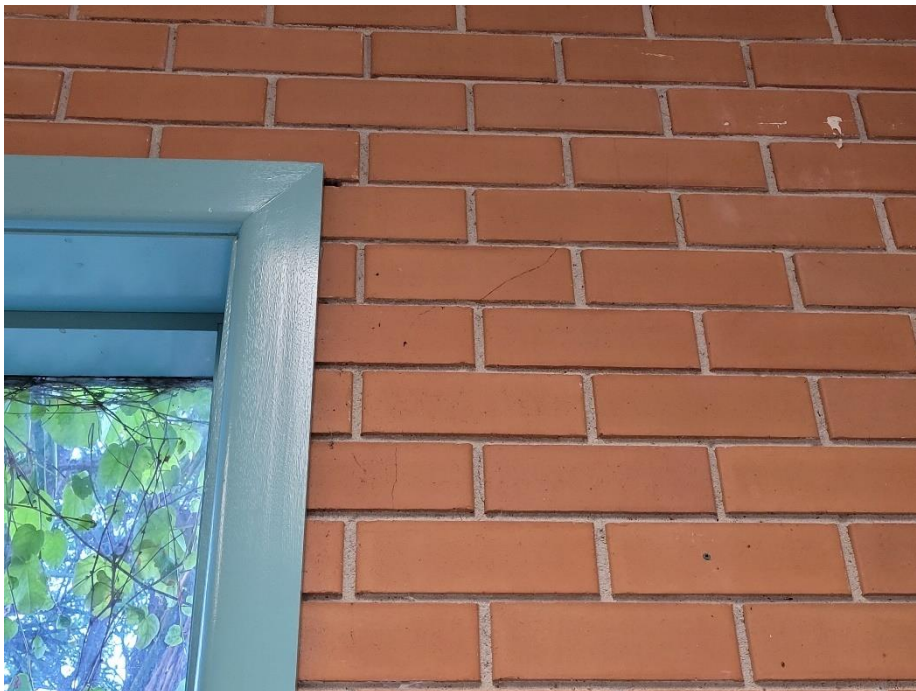
102. Cracking to bricks and across mortar joints in external wall
