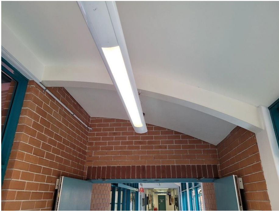
87. Crack in plasterboard at wall and ceiling junction
