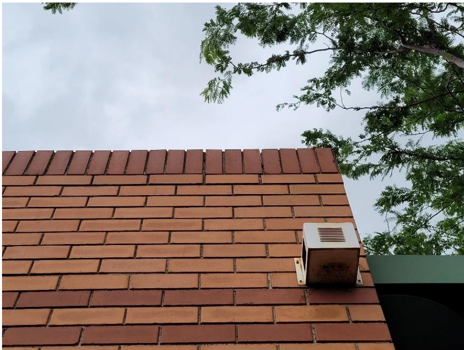
14. Crack to parapet brickwork
