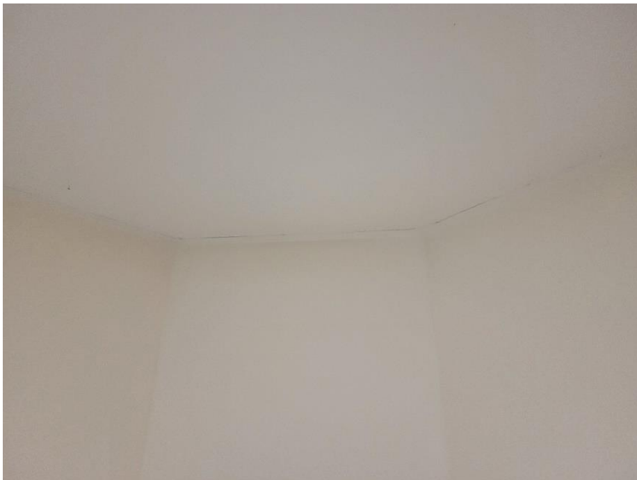
58. Crack in plasterboard at wall and ceiling junction
