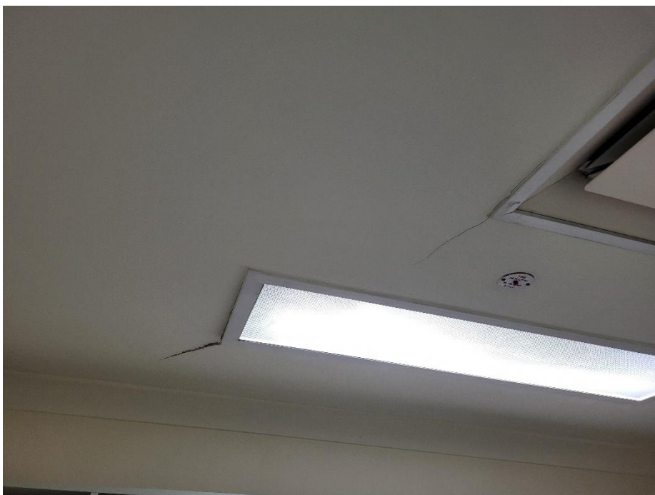
175. Cracking in ceiling around light fitting
