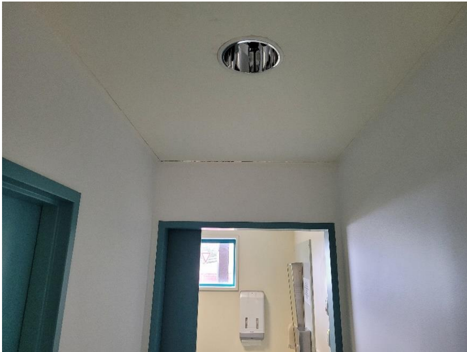
27. Crack in plasterboard at wall and ceiling junction above door opening
