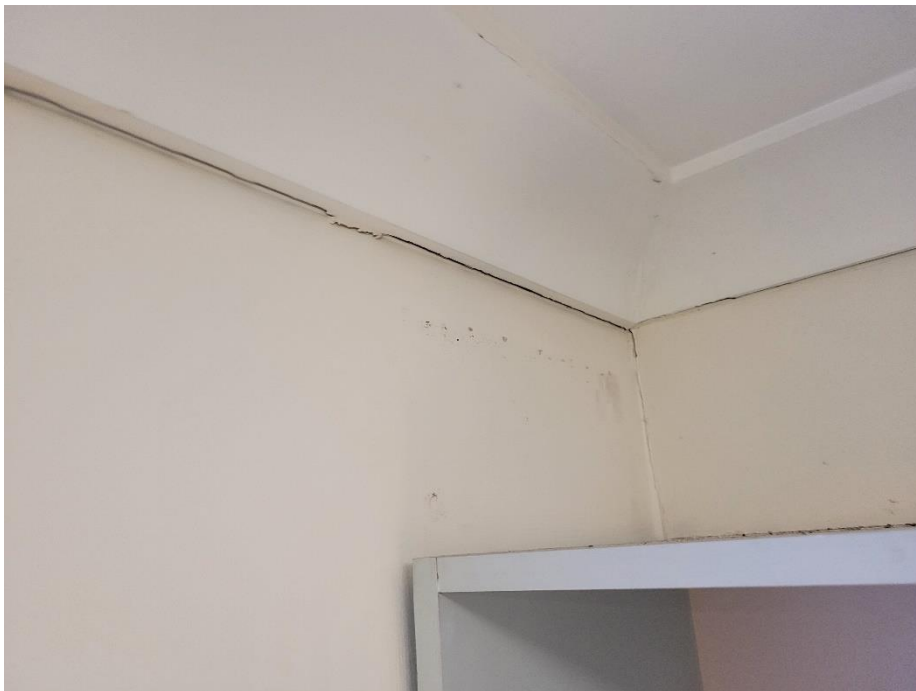
148. Crack in plasterboard at wall and architrave
