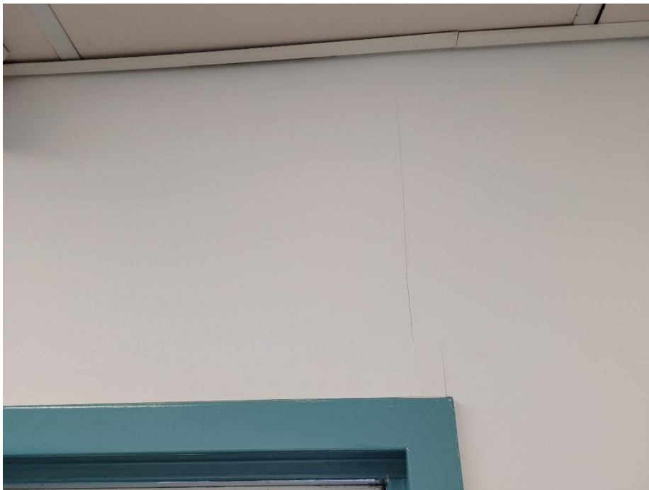
156. Vertical crack in plasterboard from door frame to false ceiling
