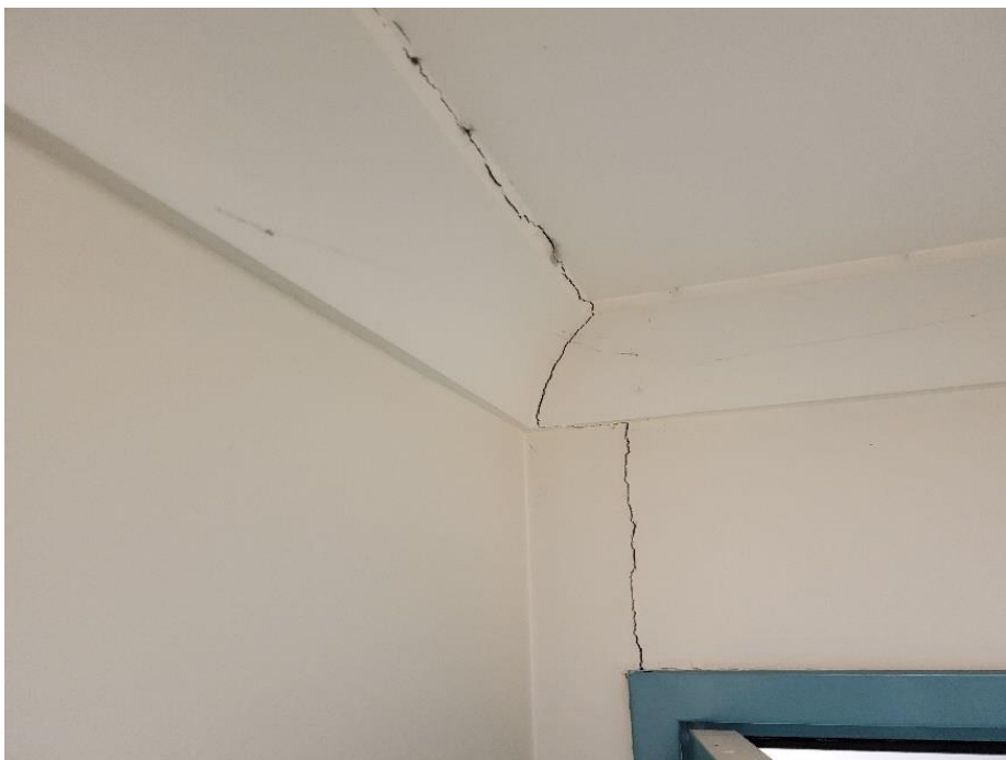
42. Crack in plasterboard at wall and ceiling junction, cracking running from window through into ceiling at joins, partition wall with hallway
