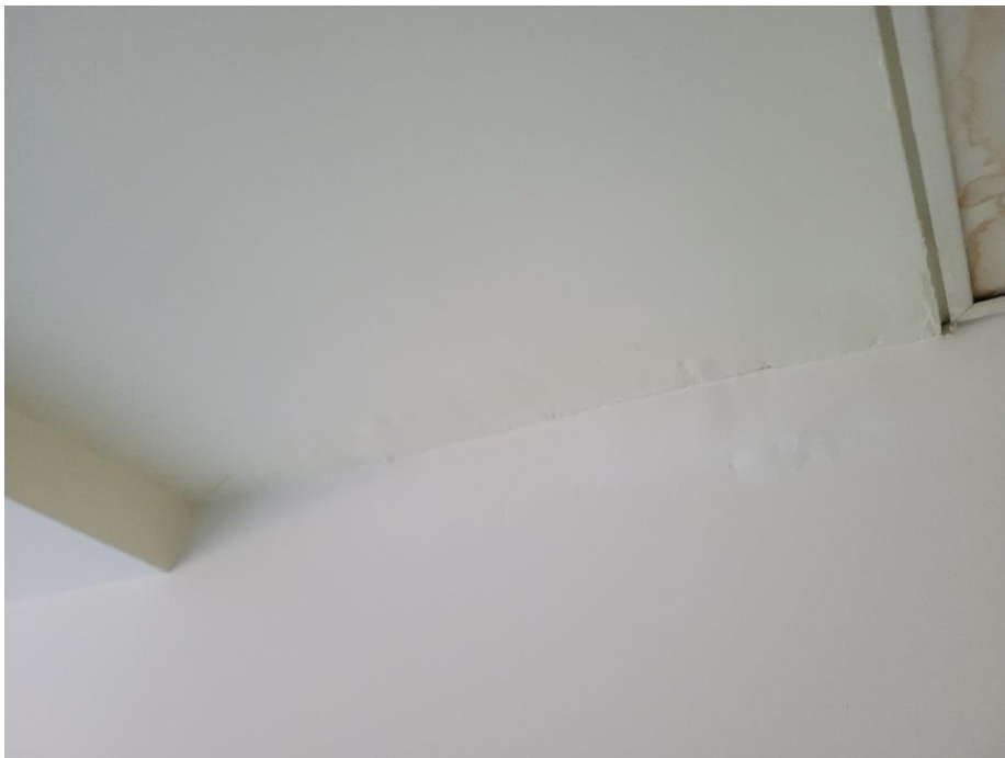
86. Crack in plasterboard at wall and ceiling junction
