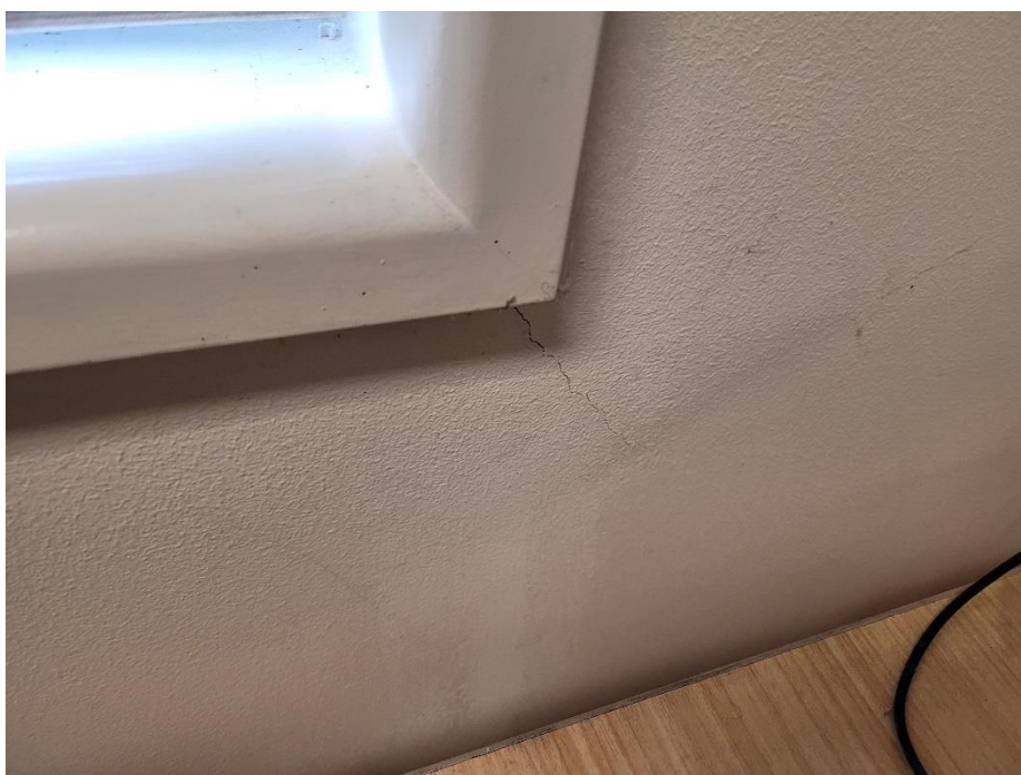
136. Cracking around window in external wall plasterboard
