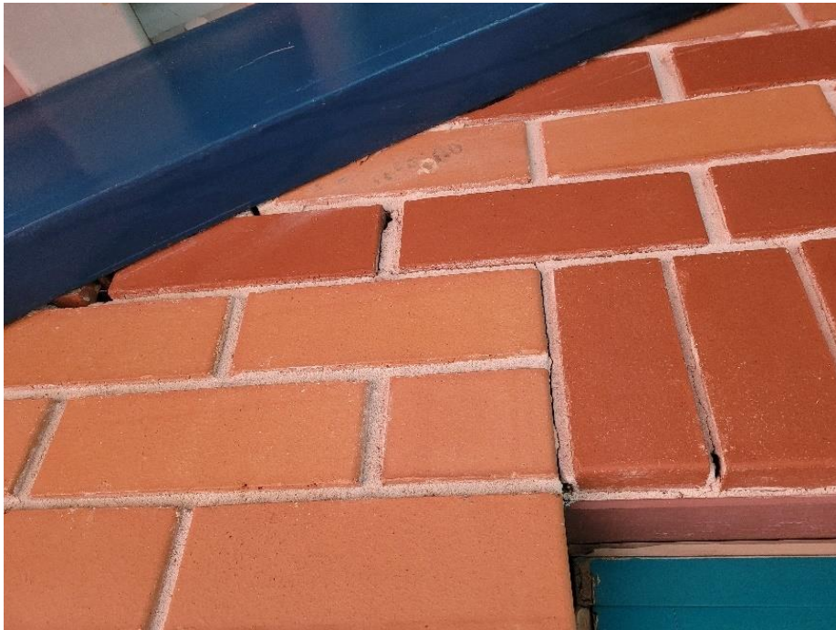
3. Cracks in mortar
