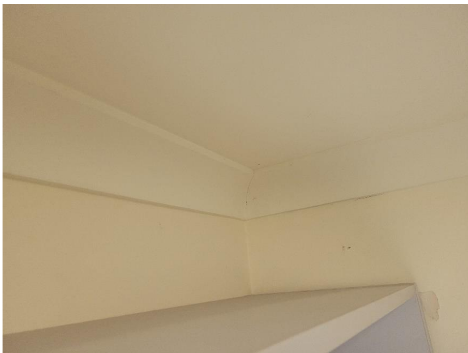
49. Crack in plasterboard at wall and ceiling junction
