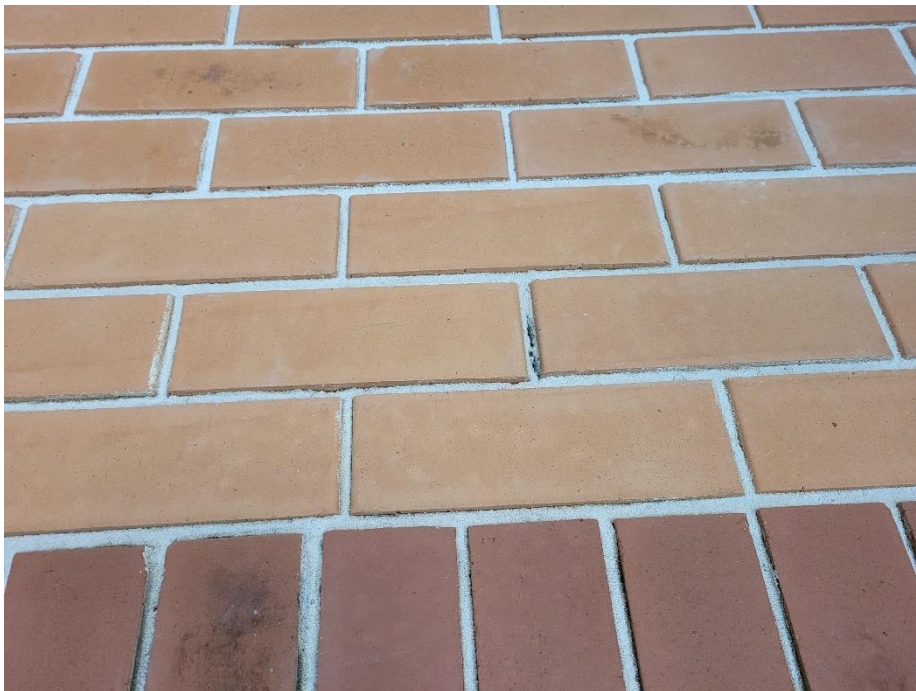
88. Minor cracking to mortar
