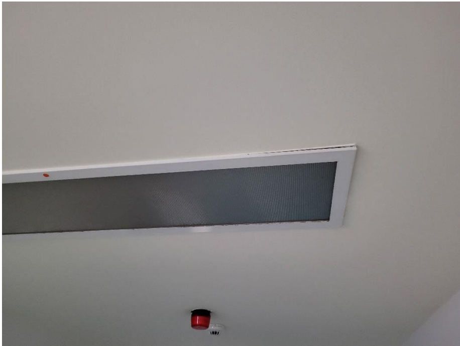
131. Light fixing coming away from ceiling
