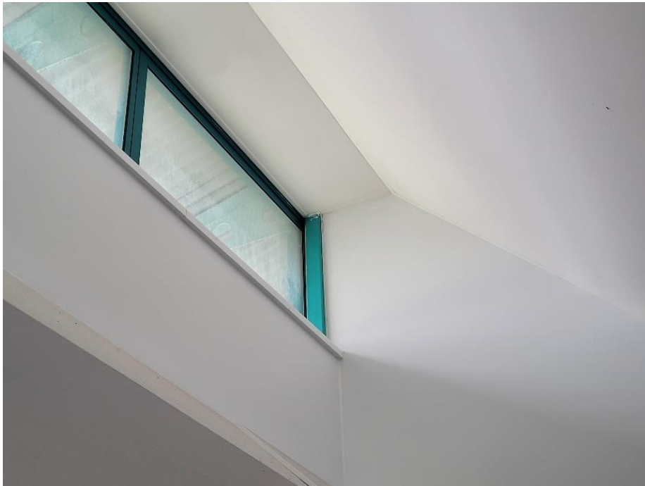
31. Crack in plasterboard at wall and ceiling junction
