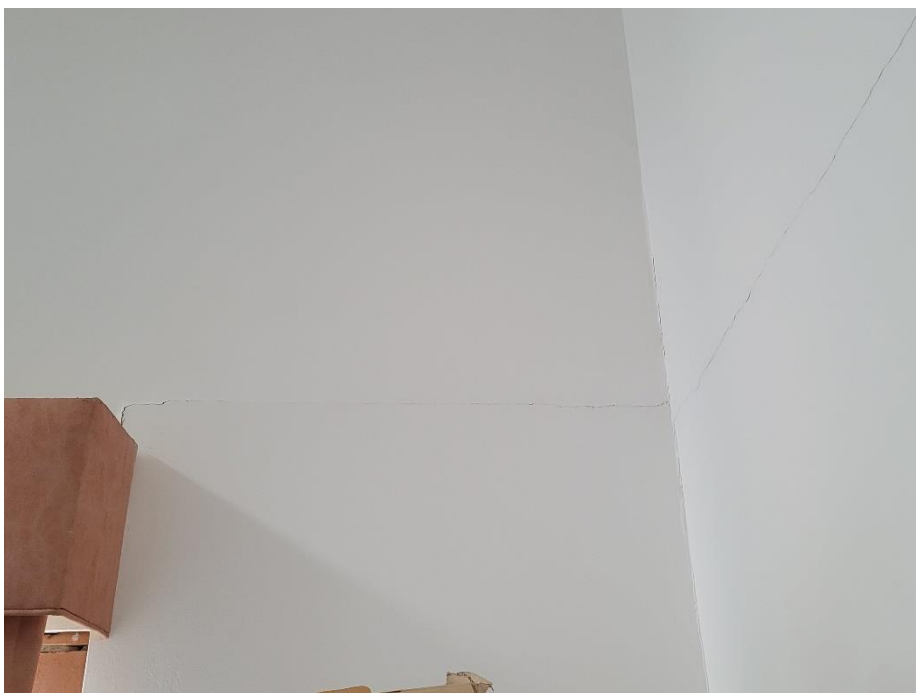
107. Horizontal cracking in plasterboard from door opening to adjacent wall, external wall
