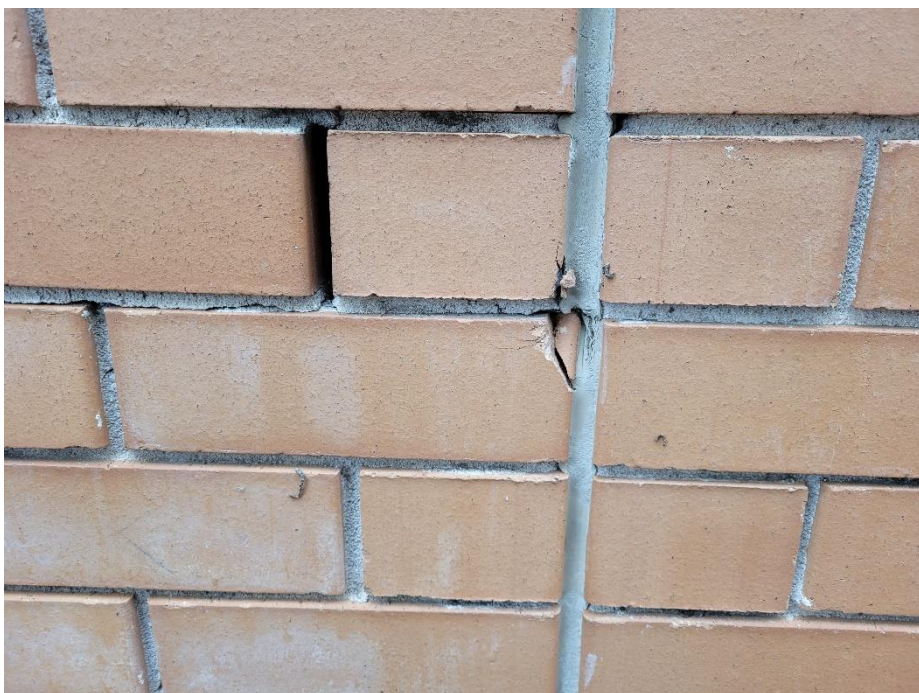
External 17. Cracking to mortar and mortar loss for external wall
