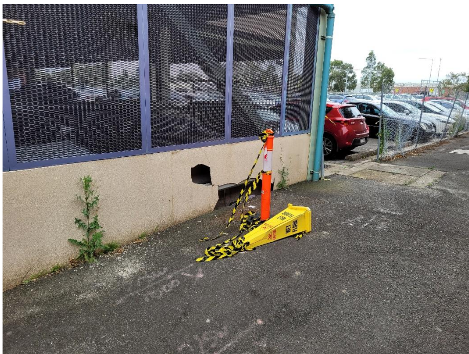
Existing Carpark 1. Damage to external cladding
