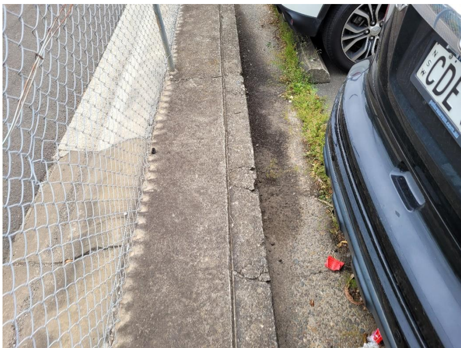
Existing Carpark 7. Numerous cracks to kerbing
