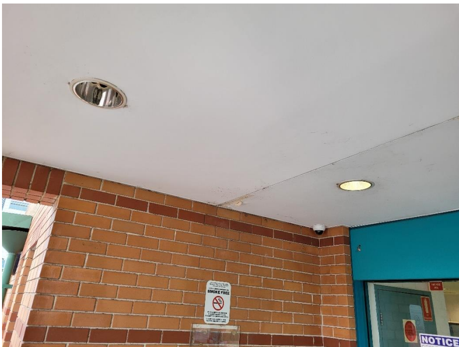
External 8. Damage and staining to external entrance way ceiling
