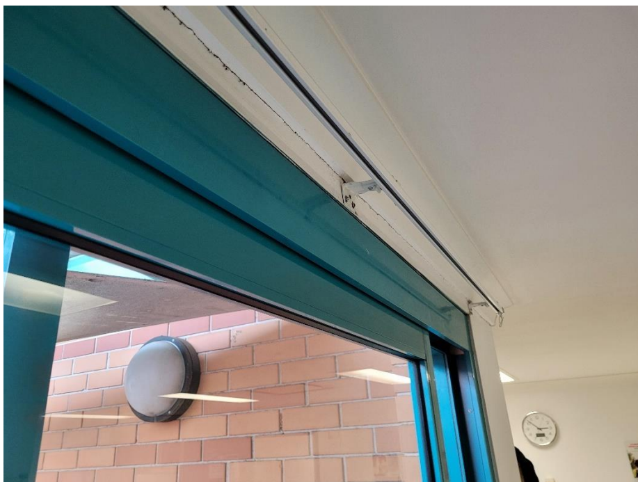
125. Cracking along doorframe
