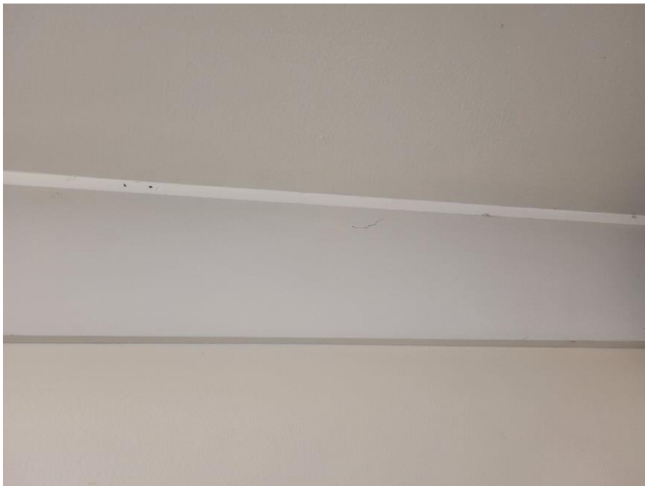
44. Slight damage and cracking in architrave
