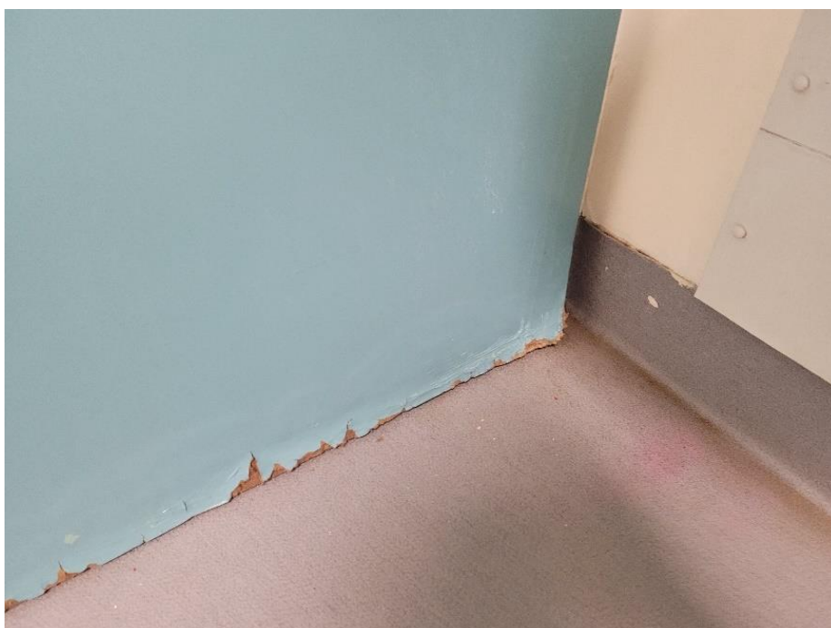
60. Water damage to door at bottom part of door
