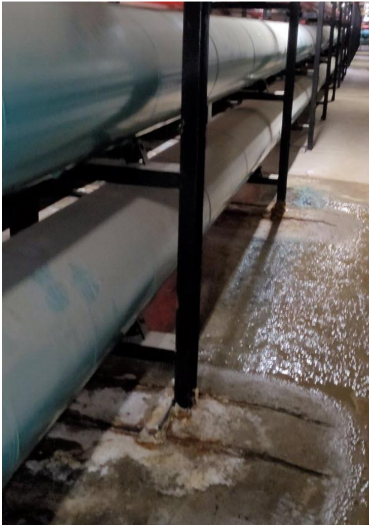
Service Tunnel 5. Leak noted in tunnel to East of BIU access point on southern side of central pipework, unknown origin
