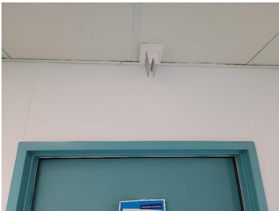
35. Vertical cracks from top of door frame corners to ceiling
