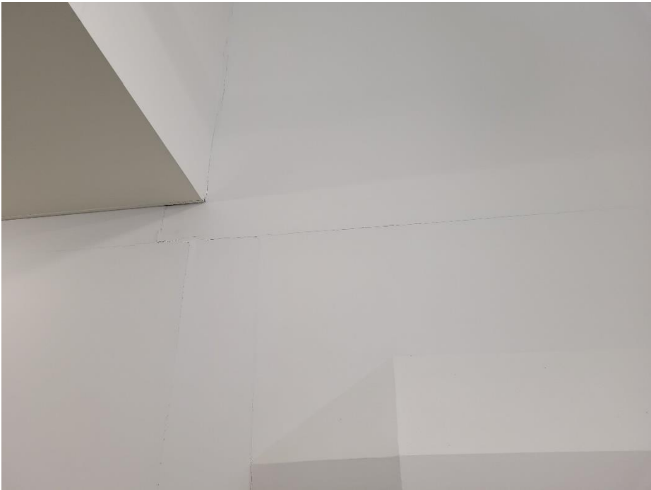
76. Extensive cracking to plasterboard around junction with ceiling, high wall section, lower wall section, light fitting, and external wall to lower ceiling
