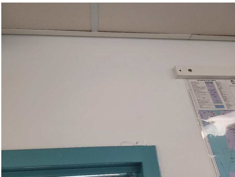
143. Vertical cracking in wall plasterboard from door frame to false ceiling
