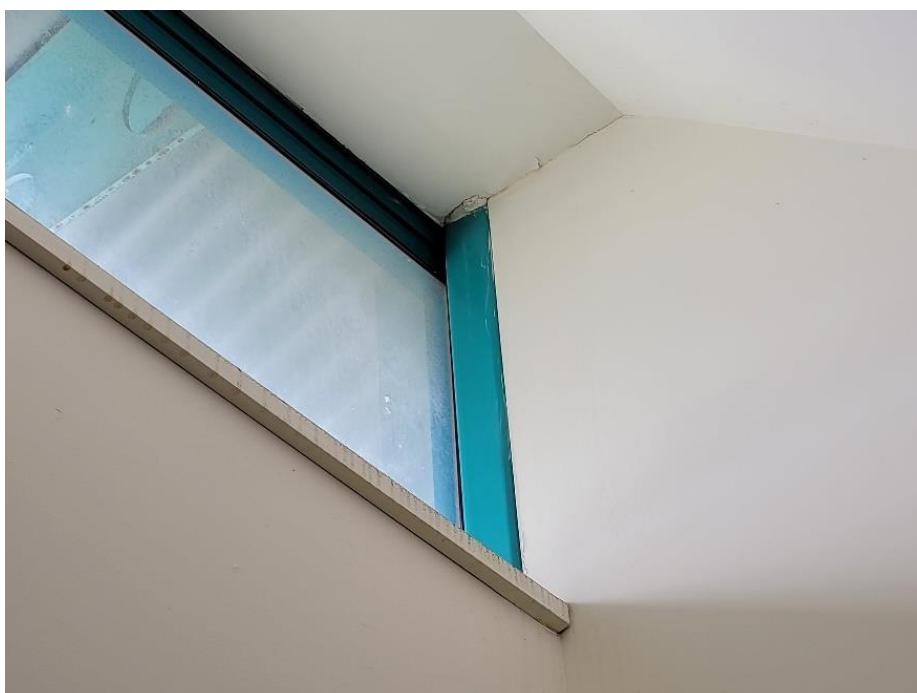
34. Damage to plasterboard around window at junction with steel post.
