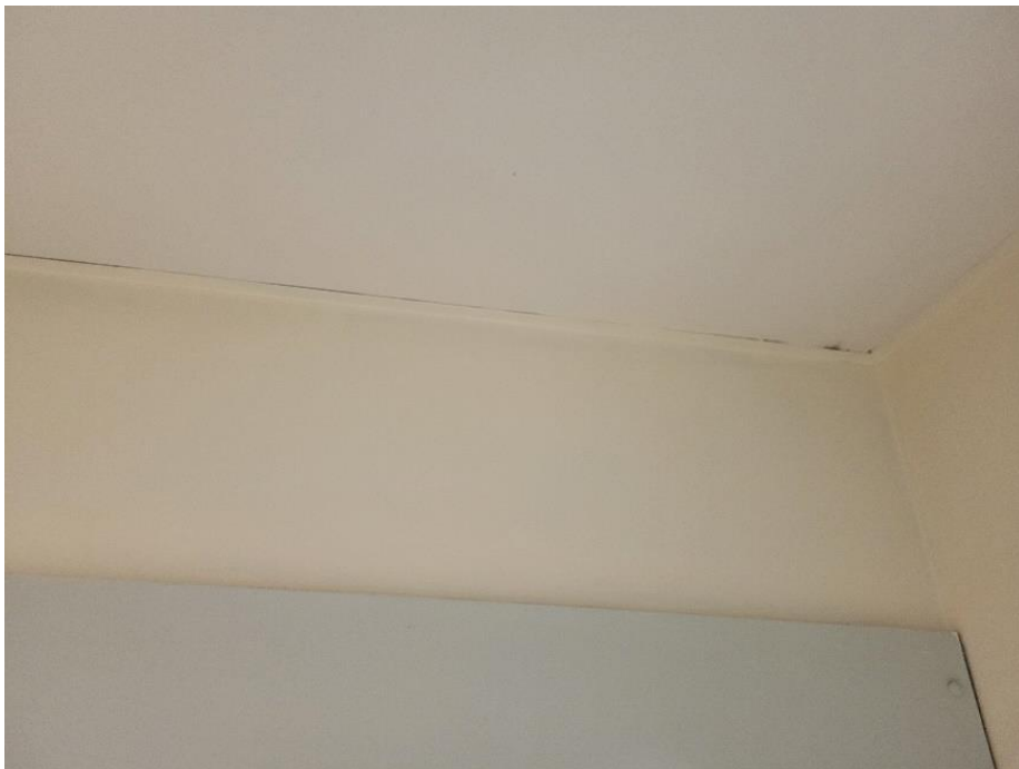
65. Crack in plasterboard at wall and ceiling junction
