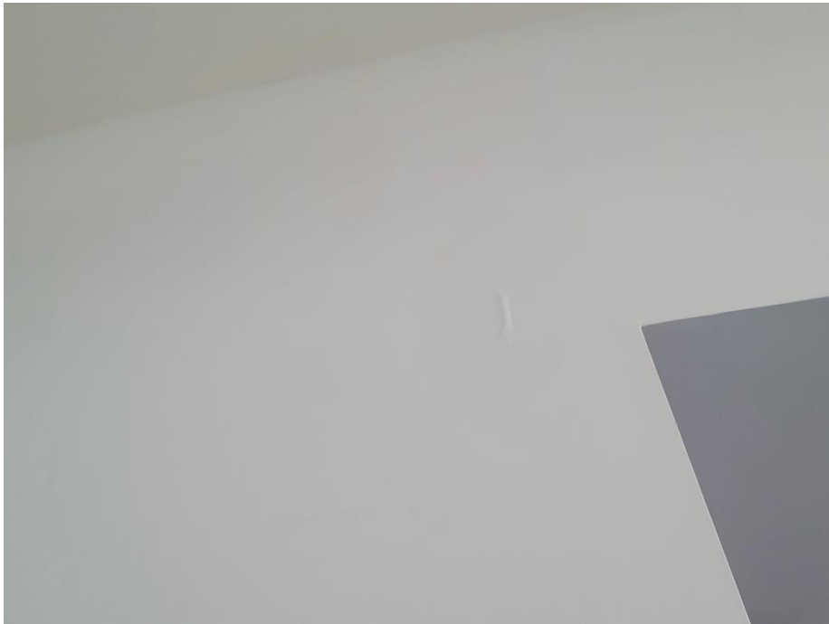
105. Minor cracking next to door opening
