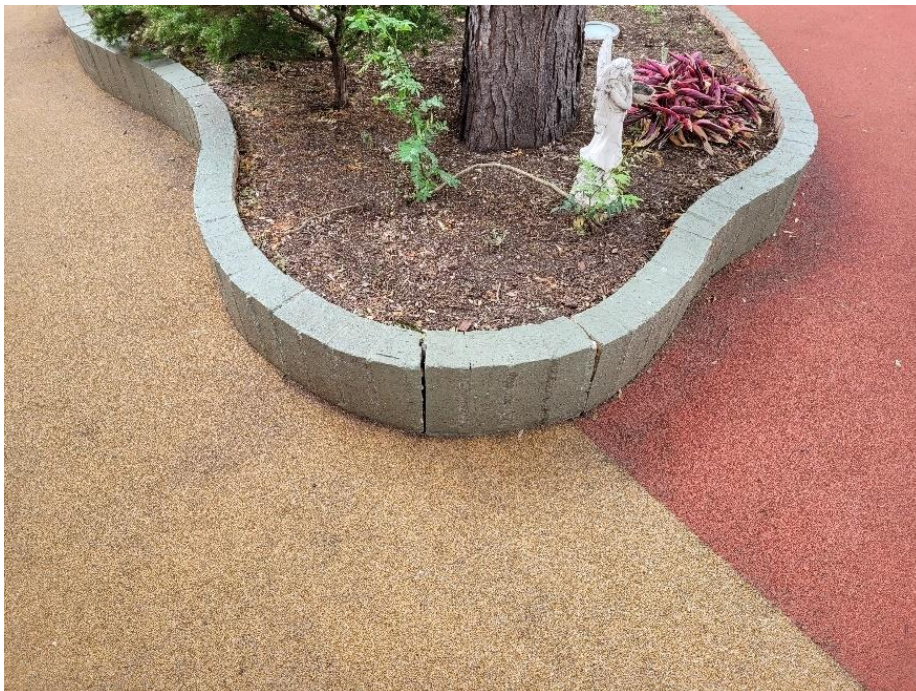
12. Garden bed brickwork damage
