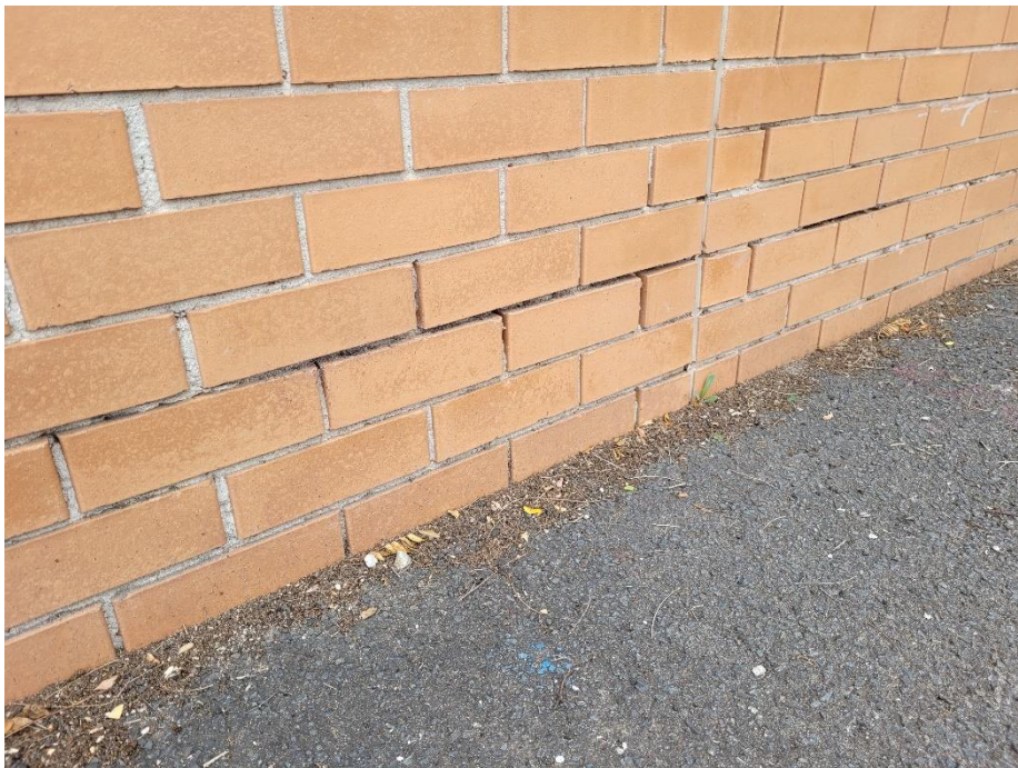
External 16. Cracking to mortar and mortar loss for high external wall
