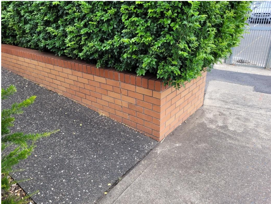
External 9. Minor cracking in planter wall mortar
