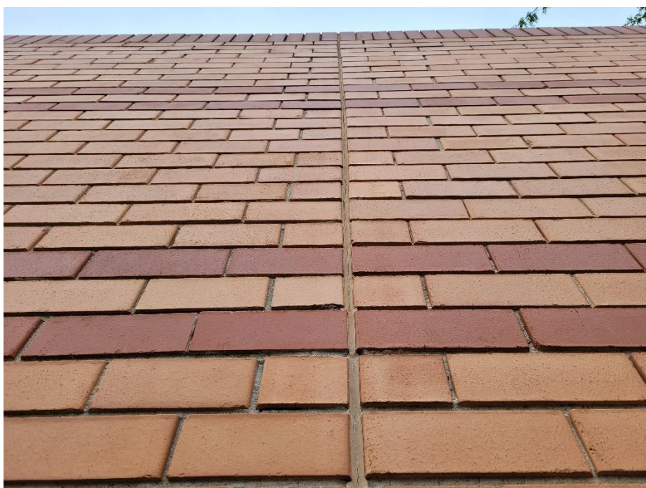
External 14. Cracking in mortar and vertical cracks/sign of wear in building joint
