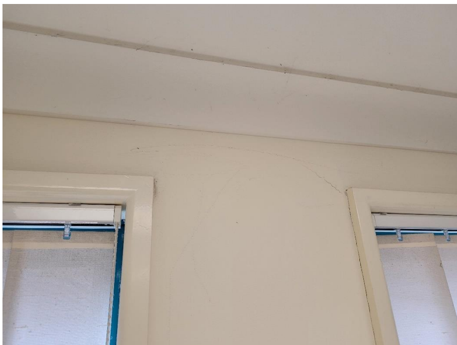
135. Cracking in wall plasterboard on external wall between window openings
