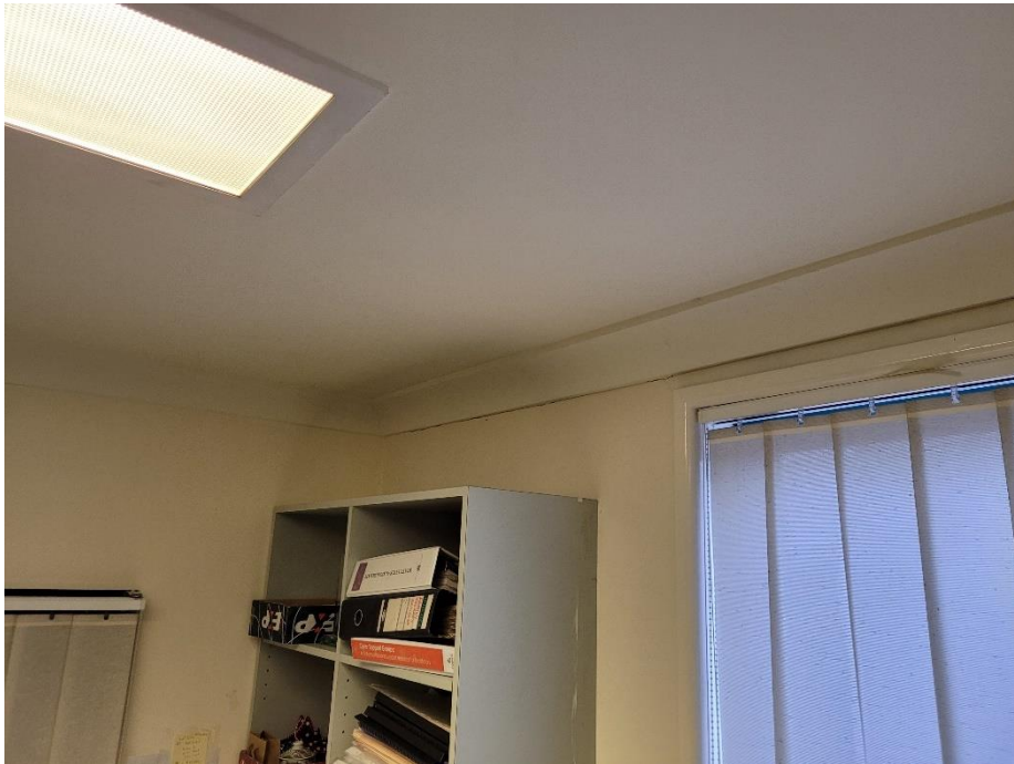
151. Crack in plasterboard at wall and architrave to external wall
