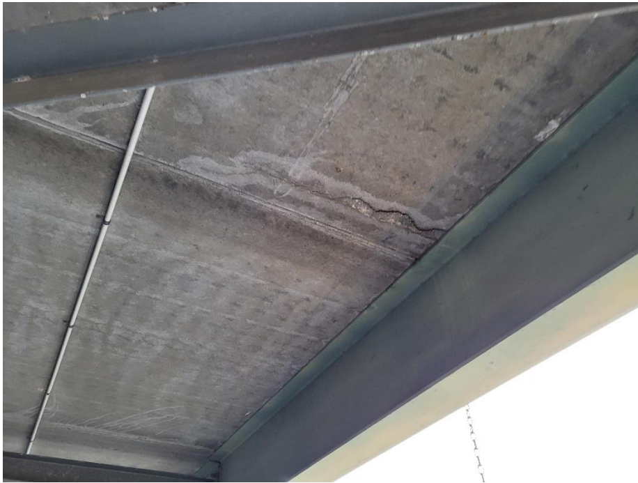
Existing Carpark 11. Cracks to soffit of first floor slab
