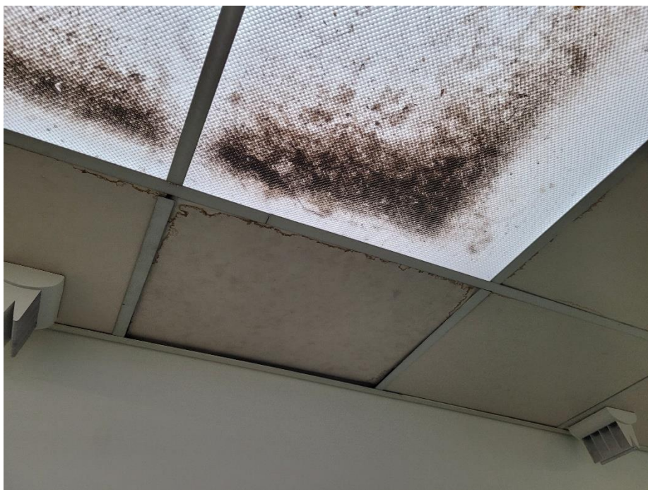
173. Water stains to false ceiling panels and collection of dust/dirt/mess in skylight
