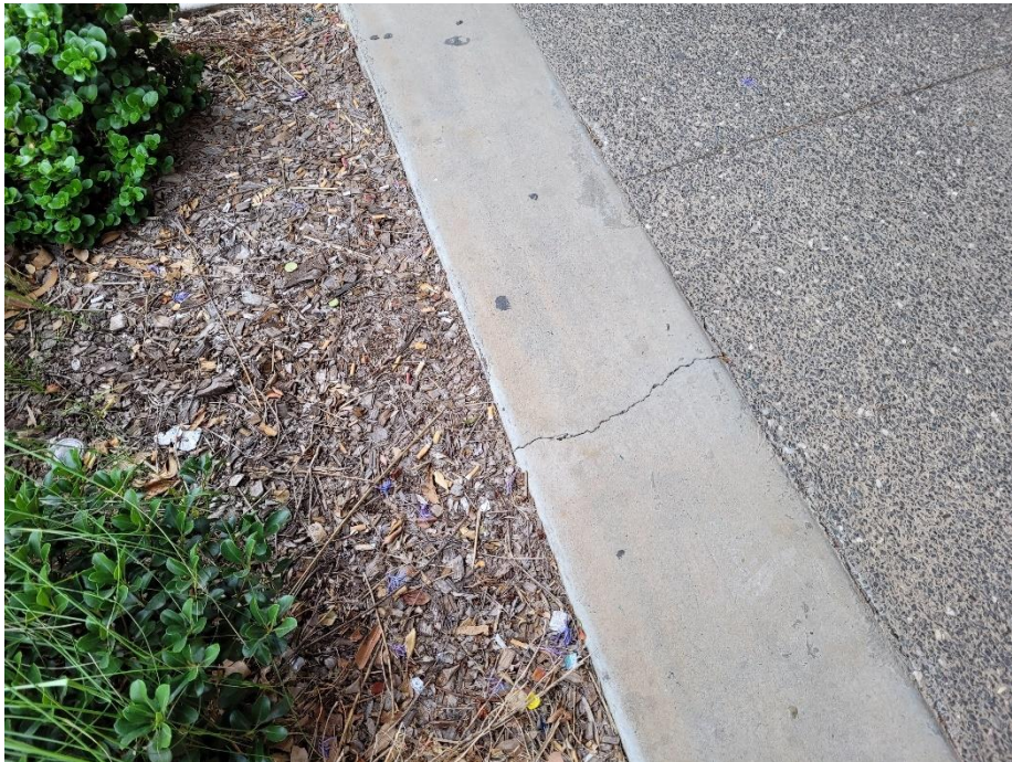
External 5a. Crack in kerb along walkway
