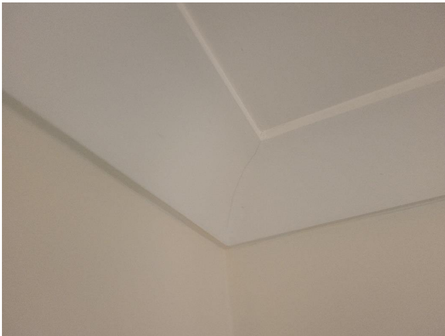
152. Crack in architrave
