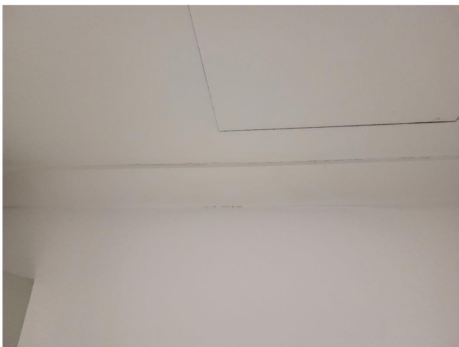
124. Crack in plasterboard around architrave
