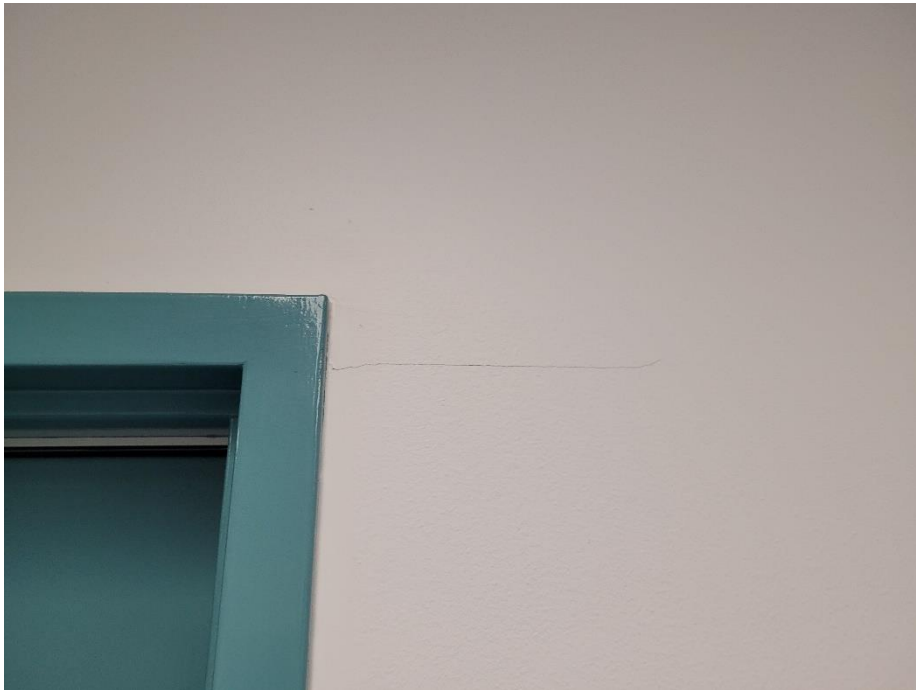
155. Horizontal crack in plasterboard from doorframe
