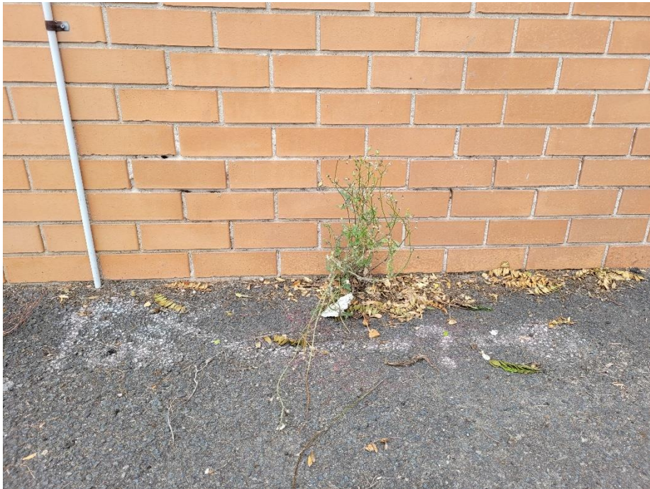
External 15. Cracking to mortar and mortar loss for high external wall
