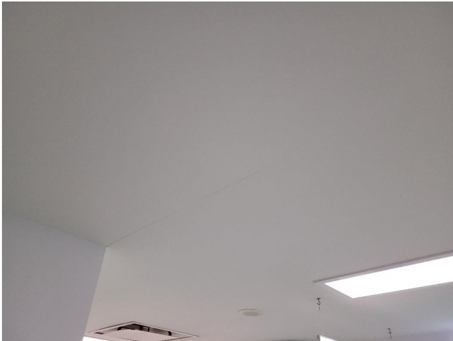
129. Cracking in ceiling plasterboard from corner of wall
