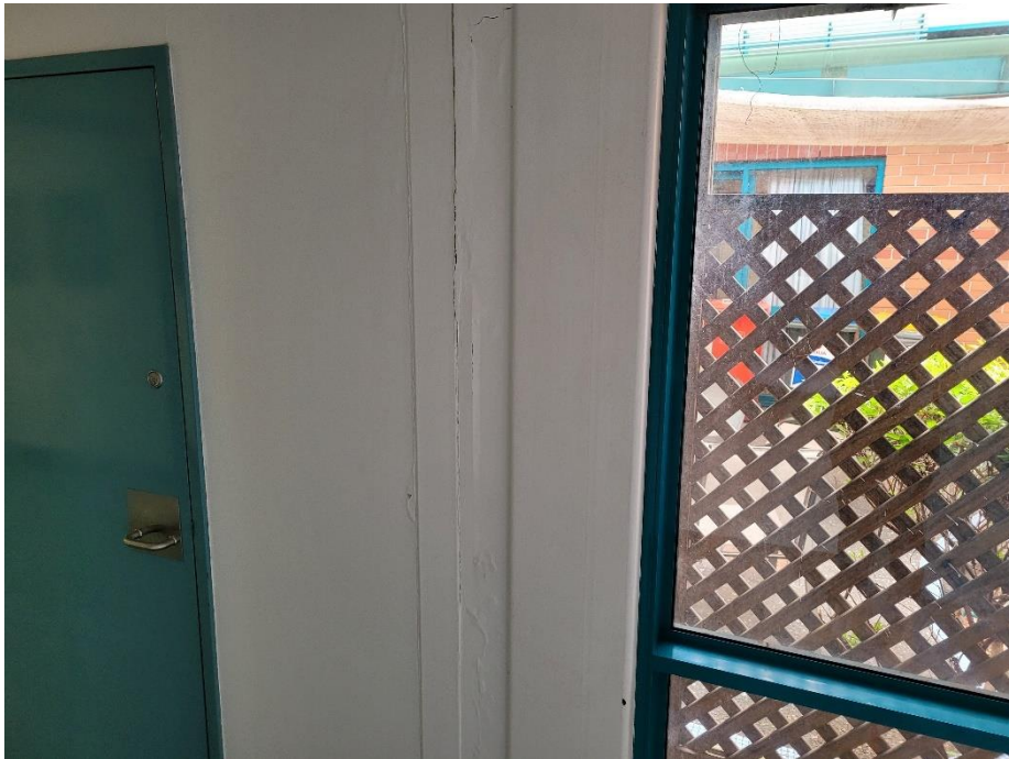
81. Cracking to plasterboard
