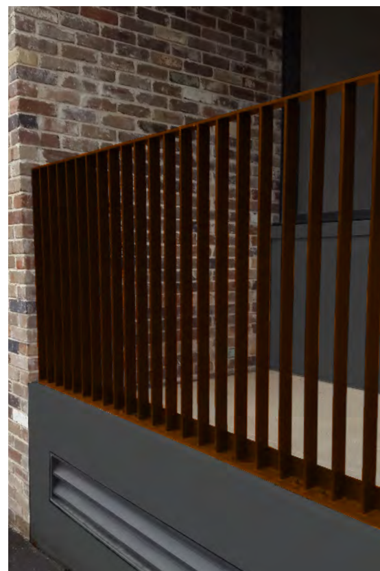
STEEL PALISADE FENCE
