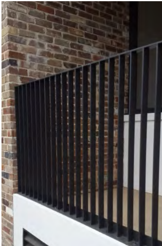
STEEL PALISADE FENCE
