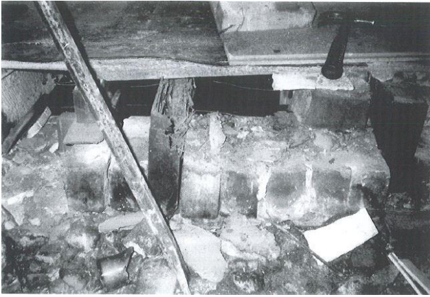
Figure 25 – image from monitoring program showing exposed subfloor area
