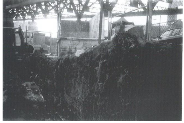
Figure 26 – exposed soils behind eastern boundary wall
