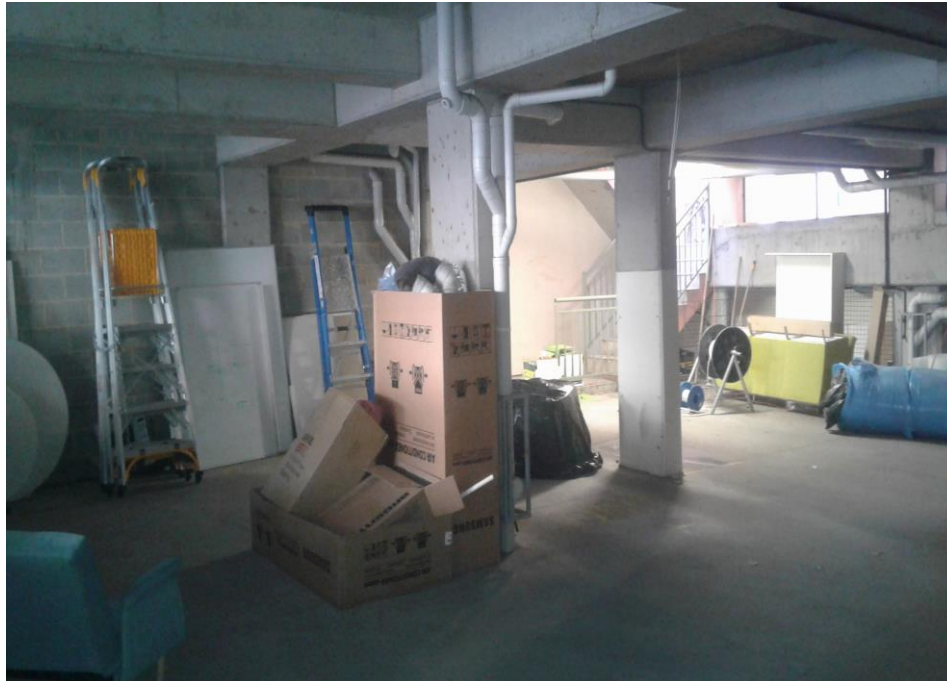
Photograph 1: Basement carpark used as a storage area
