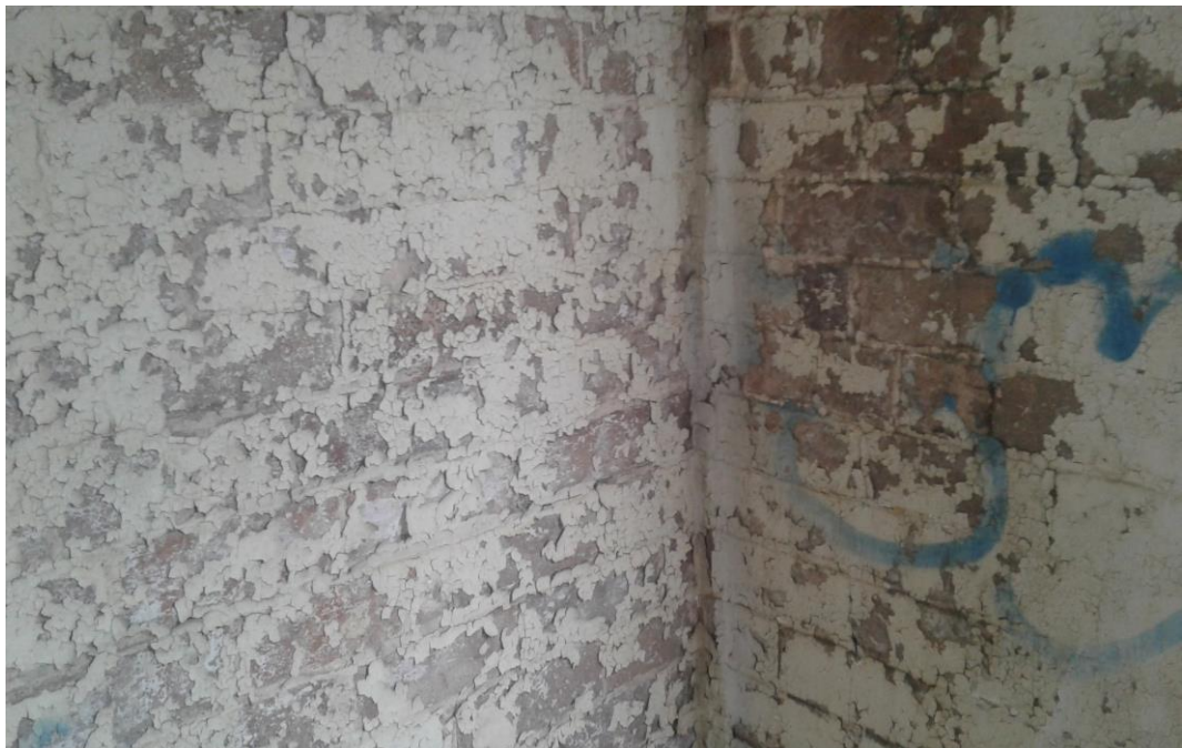
Photograph 4: No. 92 Regent Street - Flaking Paint
