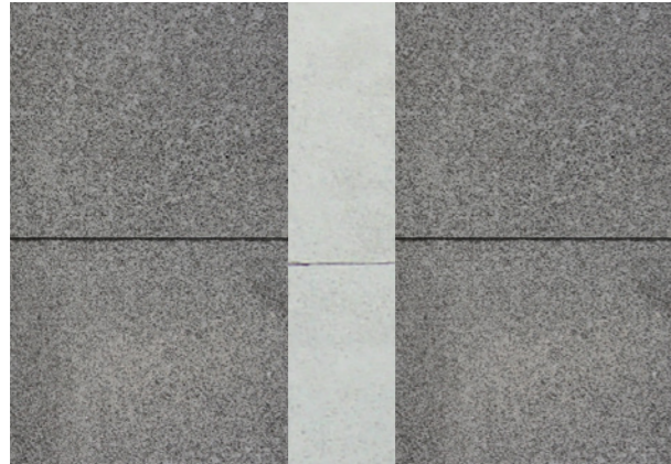
COS CONCRETE UNIT PAVER DETAIL (HONED EXPOSED AGGREGATE) WITH CONCRETE BANDING - GROUND FLOOR PAVING
