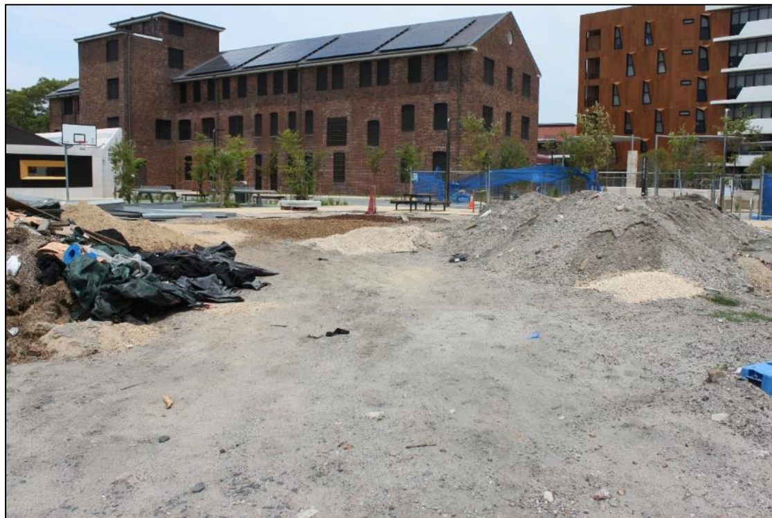
Figure 5-3 Southern quadrant of the study site, fronting Portman Street, facing south. AMAC IMG_2136, (22/01/2018).
