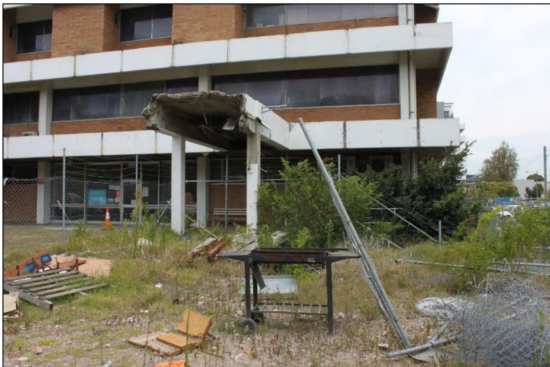
Figure 5-8 Rehabilitation Centre (Namoi Wing) and the south western quadrant of the study site, facing south. AMAC Group IMG_2145, (22/01/2018).
