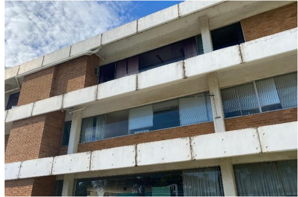
Figure 14: Western façade showing facebrick exterior with horizontal bands and white cement projecting awnings (CPH, 26 June 2020).
