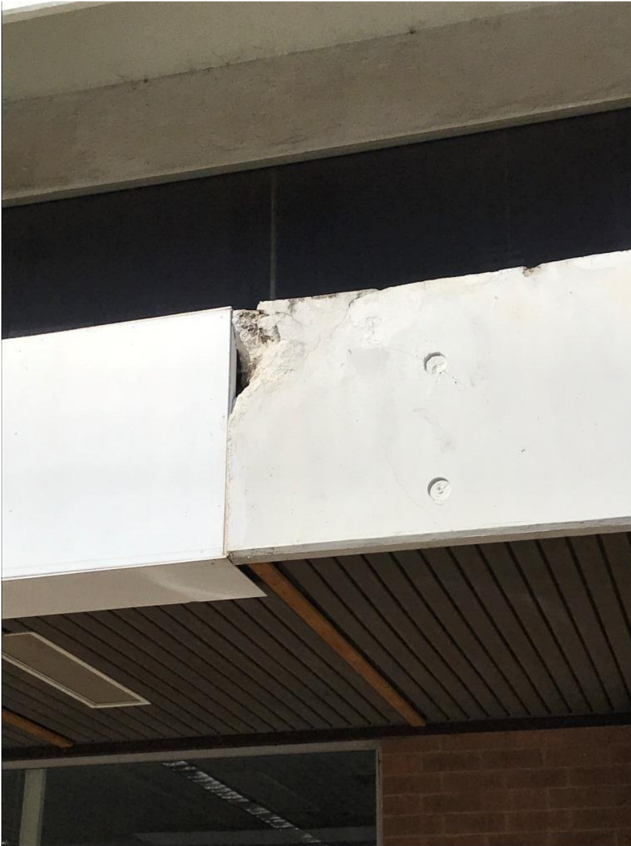
Photograph 5 Cracked concrete proving potential bat entry point
