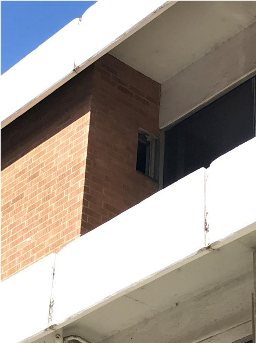
Photograph 6 Broken second floor window providing potential fauna entry point
