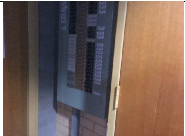
Photo 22 Internal Electrical Boards No asbestos observed
