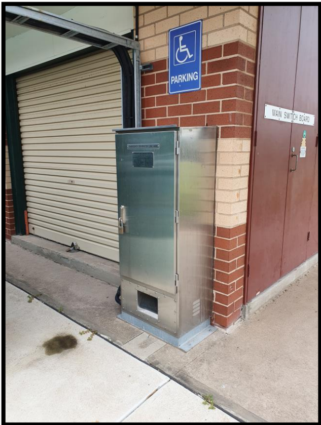
Figure 8-5 Building switch board
