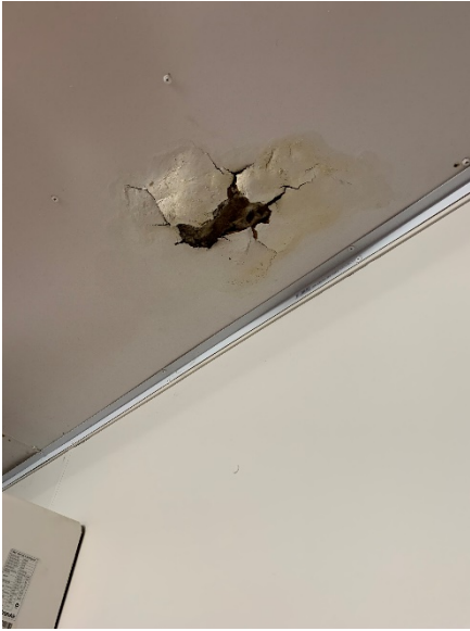
19. Insulation within E4 demountable ceiling cavities contains SMF.
