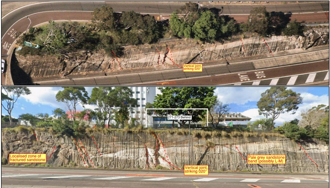
Figure 3: Ortho photo dated 5 May 2018 (above) and Google Maps Street View dated June 2021 (below) showing rock face prior to Waringah Freeway works, and marked up joints (red). Both photos looking east.
