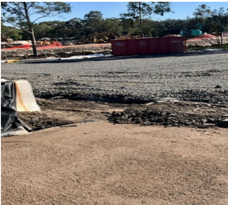
Example of gap in bunding (leachate holding tank in background)
