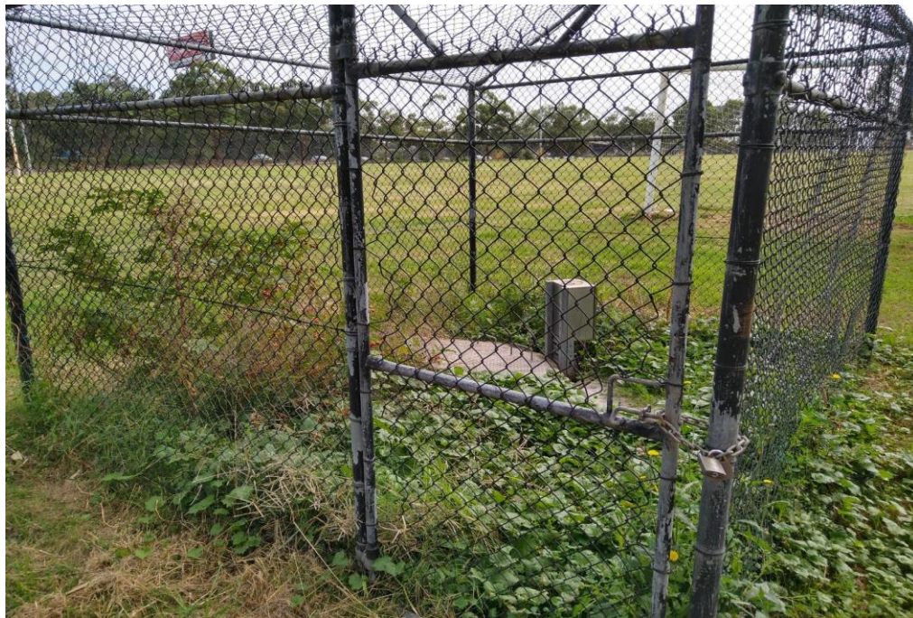
Photograph 2: Grandstand to main rugby oval, southeastern corner, interception and valve pit, materials in general, inaccessible.
