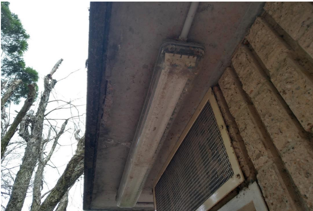
Photograph 8: Central amenities block, exterior, fluorescent light fitting(s), internal components (e.g. capacitors, ballasts), insulating oil, PCB (assumed).
