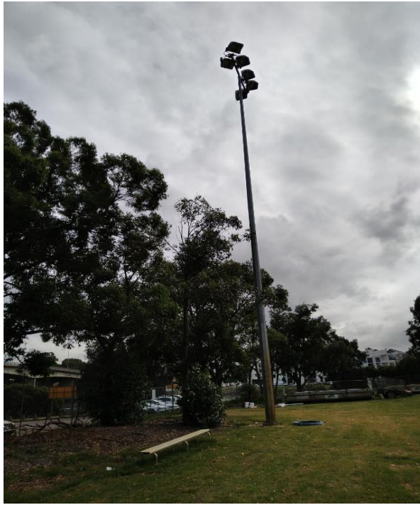
Photograph 3: Main rugby oval, perimeter, field lights x 4 (approx.), internal components (e.g. capacitors, ballasts), insulating oil, PCB (assumed).
