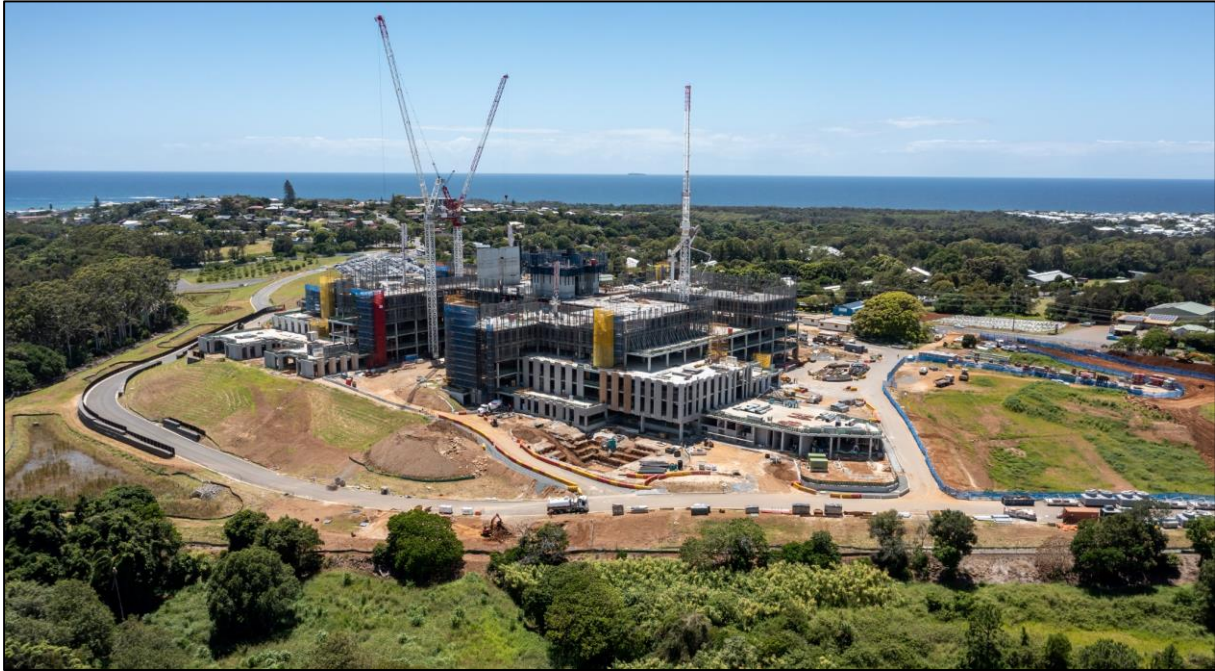
Plate 1.1 Photo showing the Tweed Valley Hospital under construction in December 2021 (source HI).
