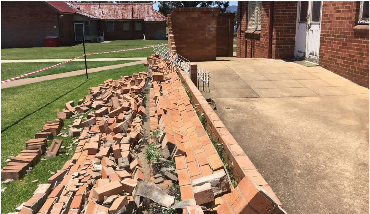
Image 2: Brick wall collapse due to rotor downwash pressurisation
