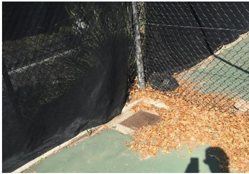
Figure 2 Blocked pit in southern tennis court
