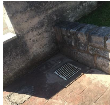
Figure 3 Blocked pit between buildings E and A
