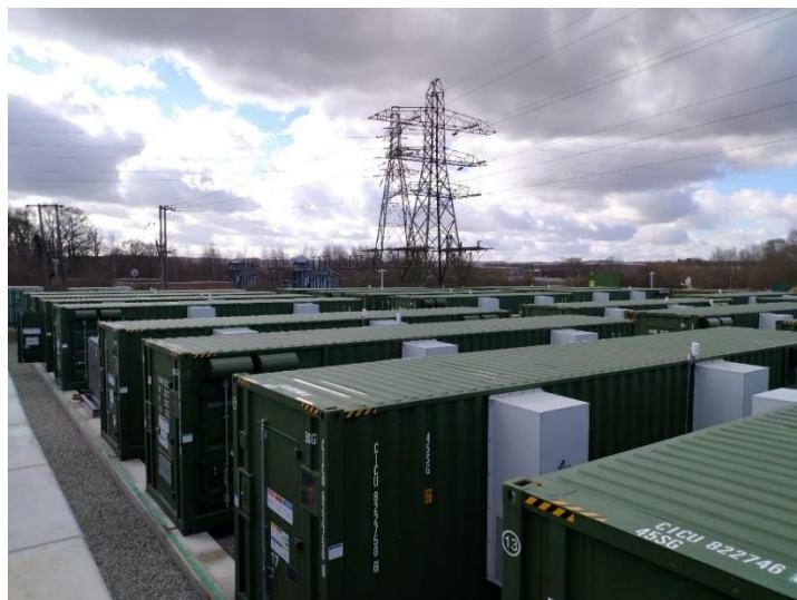
Figure 3-2 Typical battery storage units, located together.
