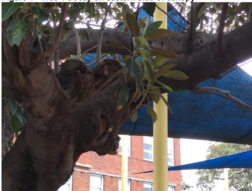
Figure 2 - Decay in secondary branch north of Tree 1
