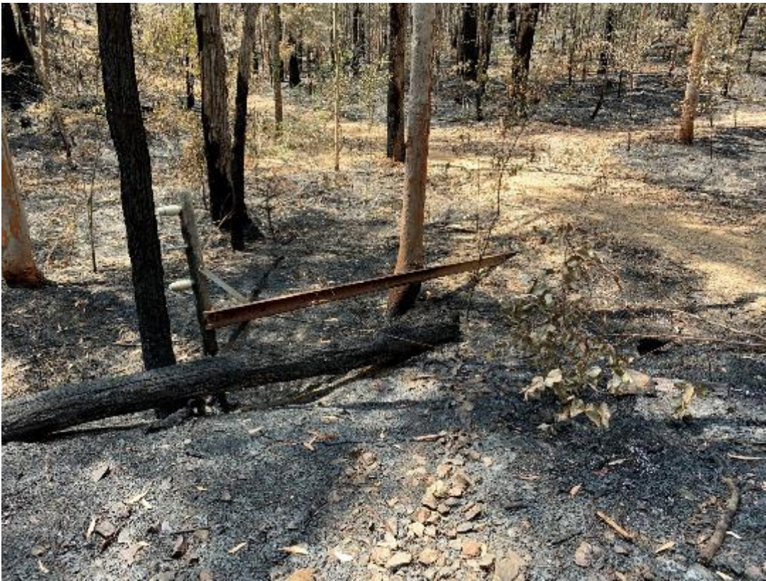
Plate 5.23 Power pole associated with the Line burnt and no longer in situ
