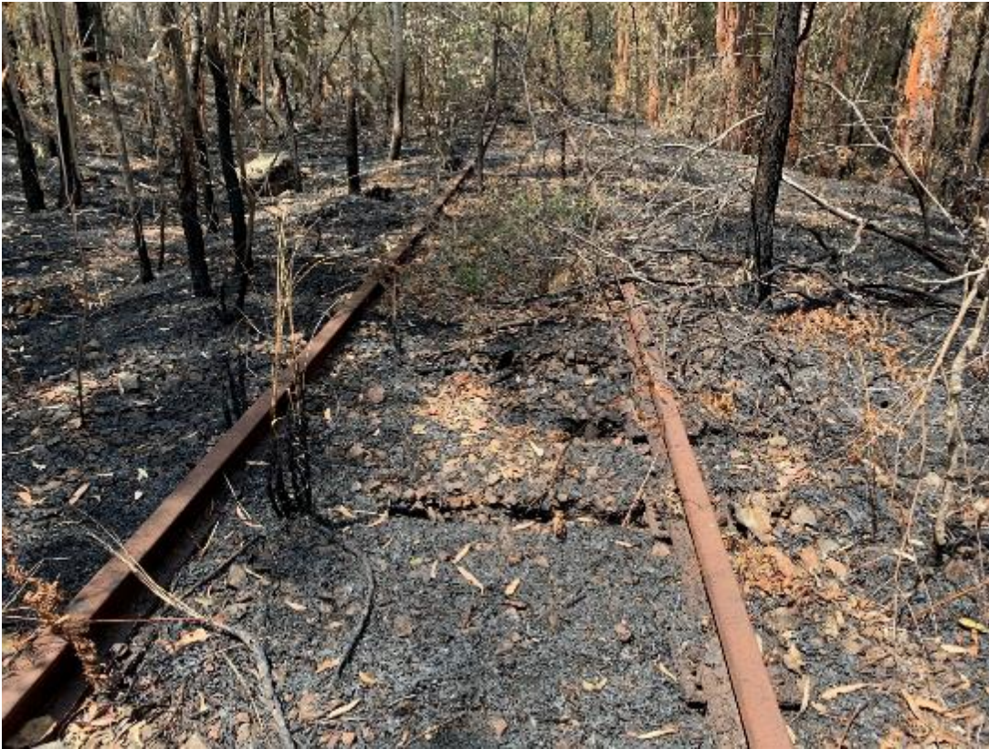
Plate 5.22 View of the Line during the one-day survey, following bushfire damage. Note the absent sleepers.
