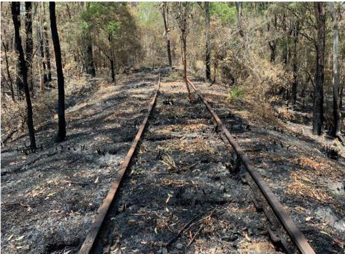
Plate 5.21 View of the Line during the one-day survey, following bushfire damage. Note the absent sleepers.
