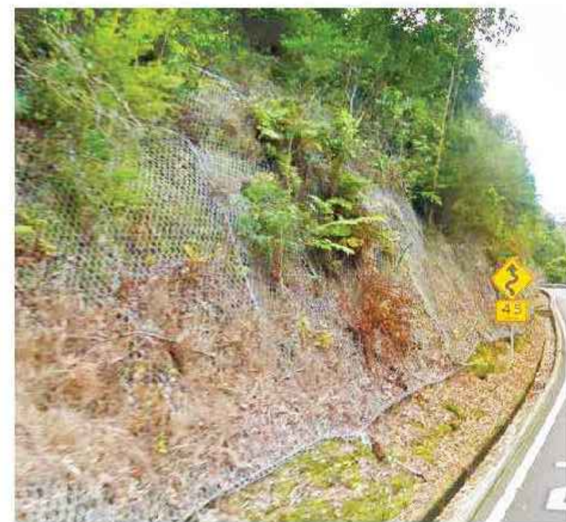
Rock face stabilised mesh
