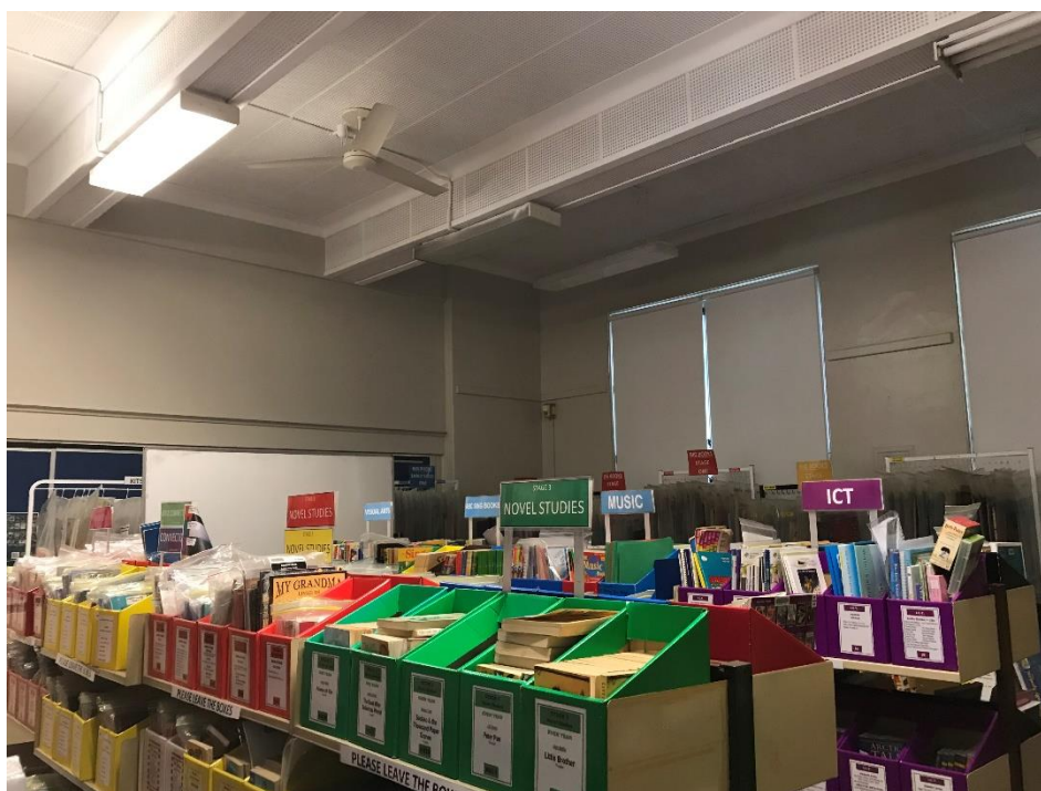
Figure 29 Ground floor classroom which has been converted for use as a store room for teachers resources. An acoustic tile treatment has been installed on the ceiling (January 2019)
