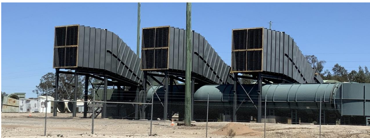
Plate 2-4 Existing Upcast Ventilation Infrastructure
