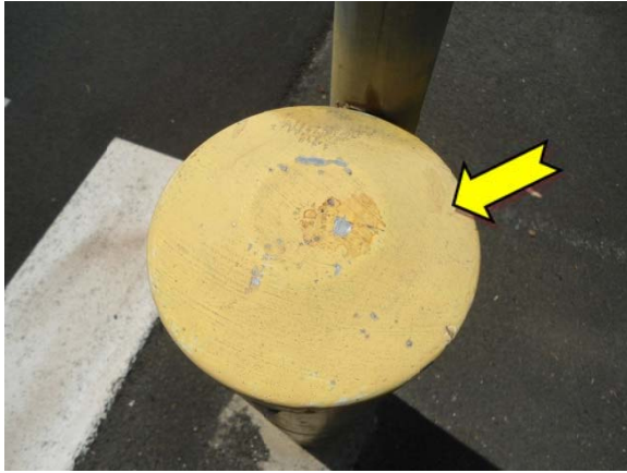
Photo 1. Ground level, various areas throughout car park, steel bollards – lead-containing yellow upper coloured paint system
