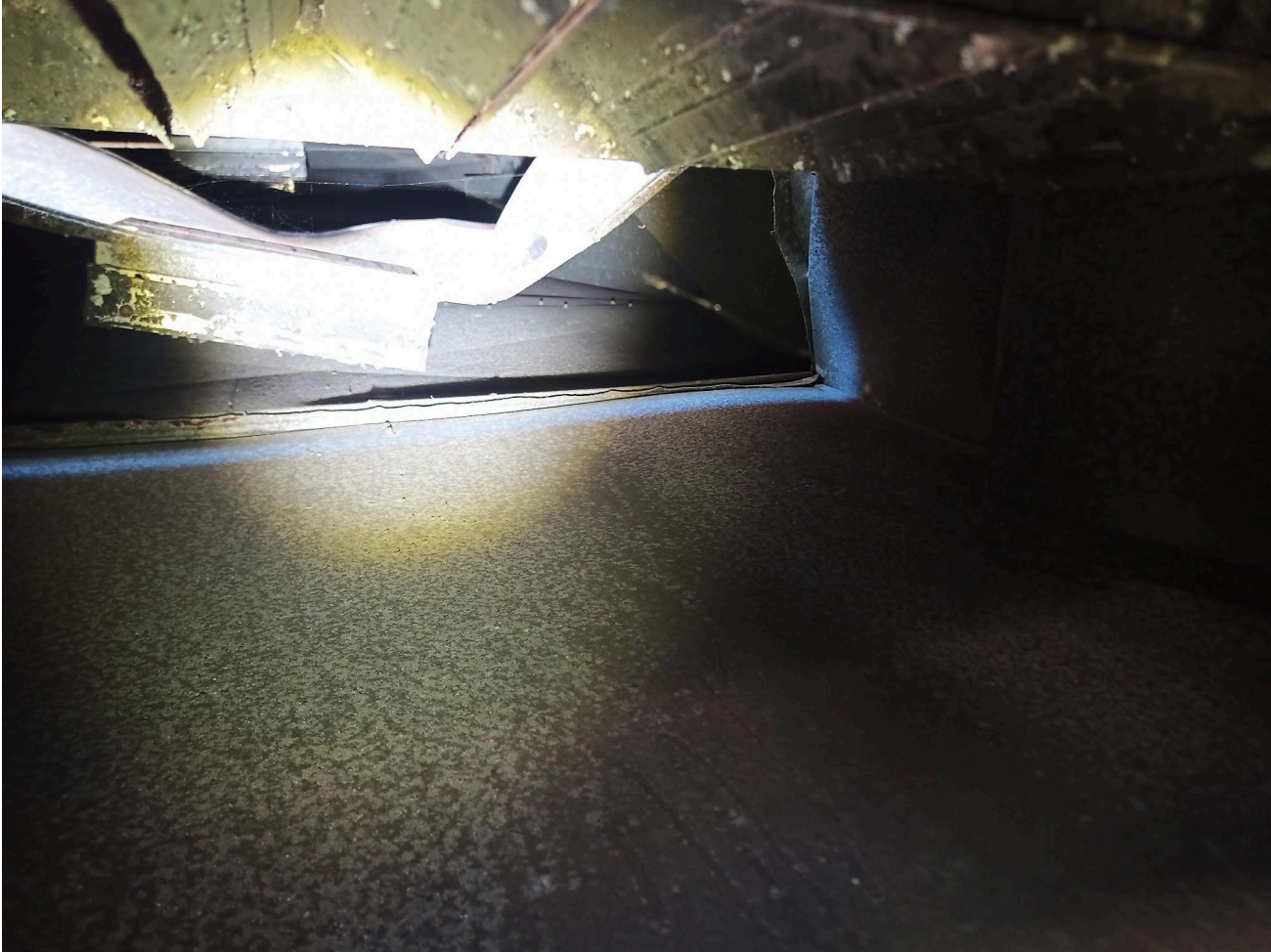
Photo 5 - representative photo of inspections of derelict air conditioning vents undertaken within the semi-demolished structure
