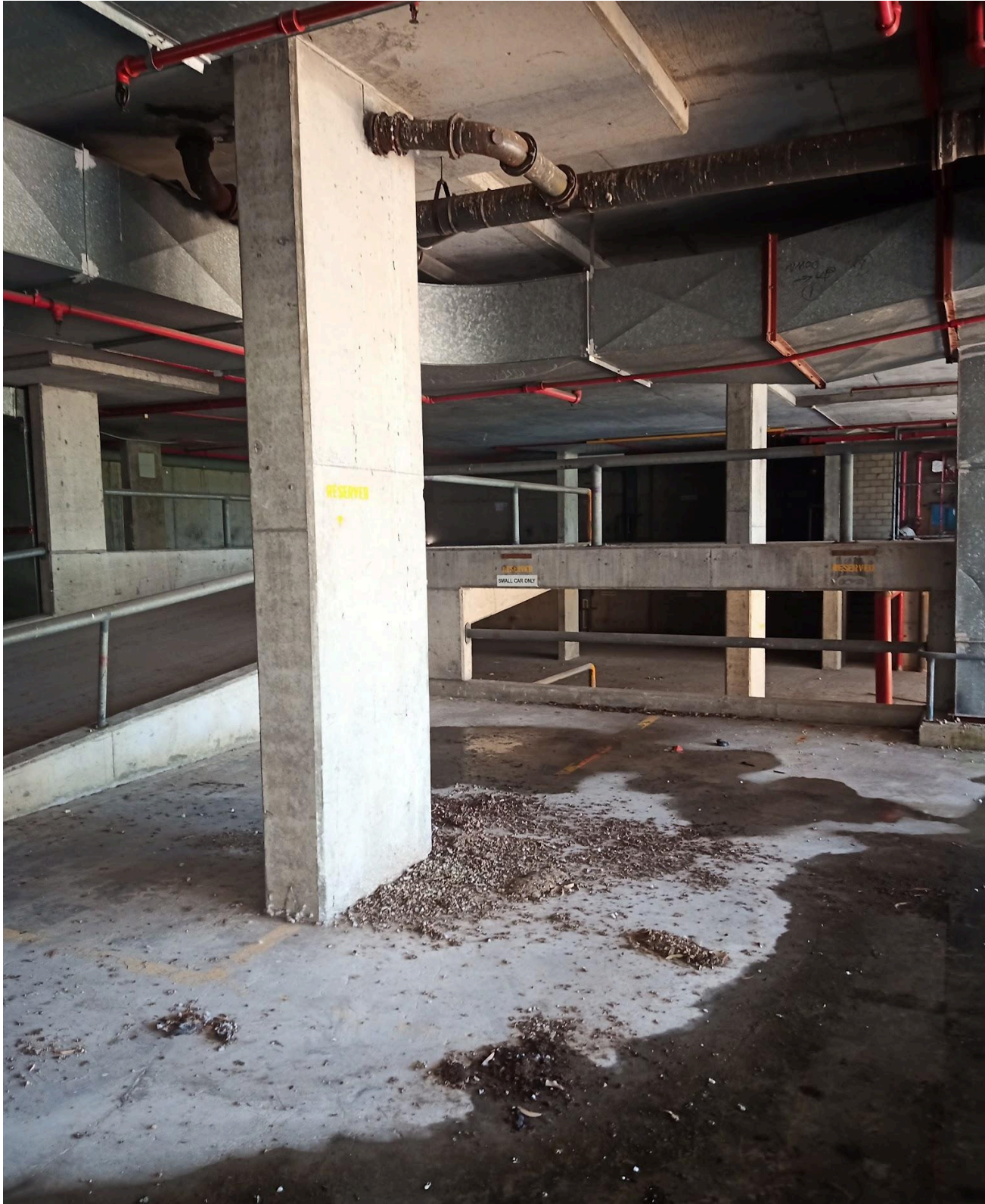
Photo 7 - Pigeon guano observed within the top level of the semi-demolished structure
