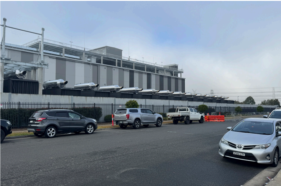
CDC DATA CENTRE
