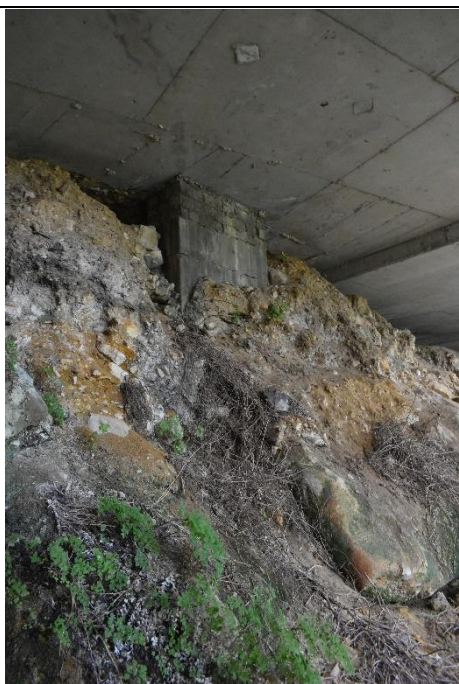
Figure 13: View North of debris under office building
