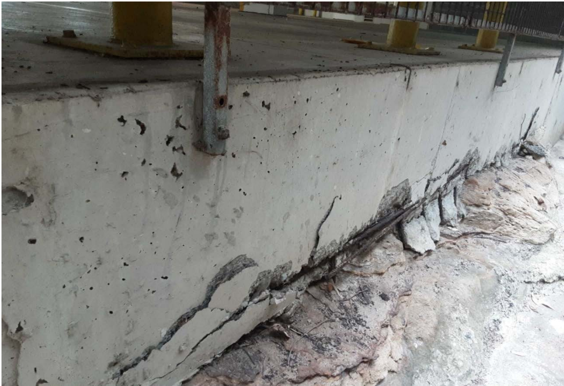
Photograph 3: Iron support beams exposed from concrete slab in north eastern corner of building (9 September 2024).
