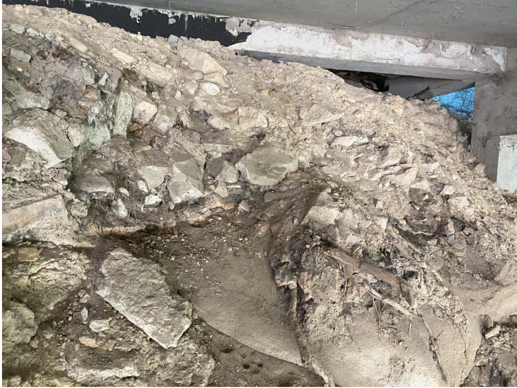
Photograph 7: View of fill material (containing demolition waste) beneath suspended slab under eastern end of car park area, facing north (9 September 2024).
