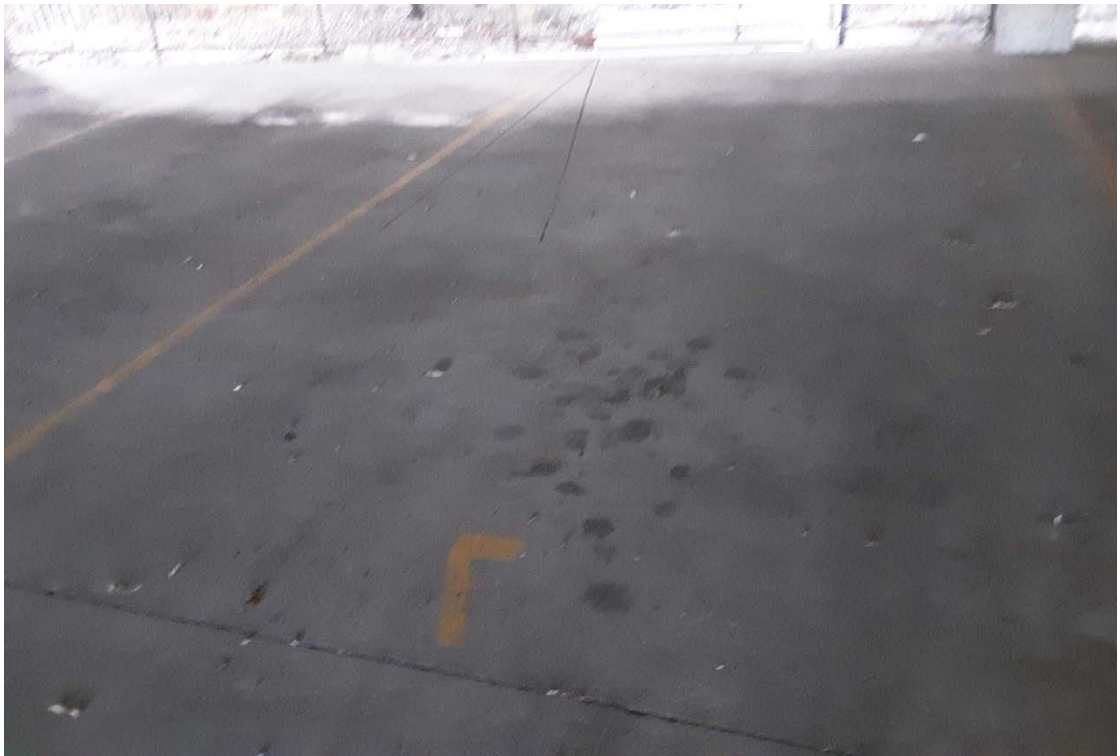
Photograph 5: Some staining in beneath building car parking area (9 September 2024).
