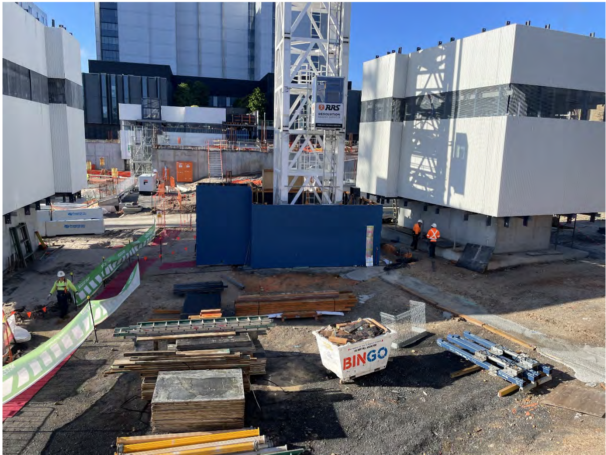
Figure 6 General waste bins in place
