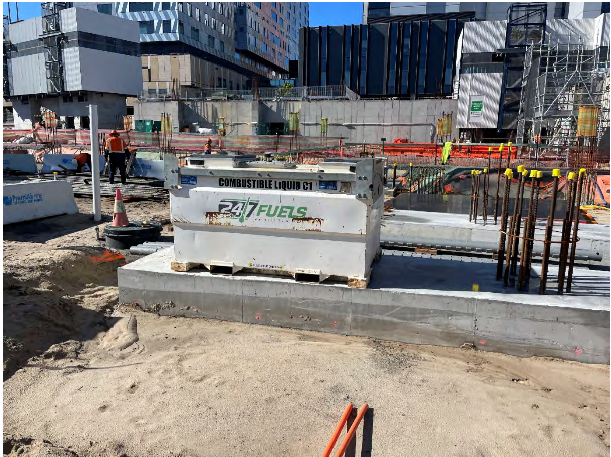
Figure 15 Self bunded refuelling container for cranes
