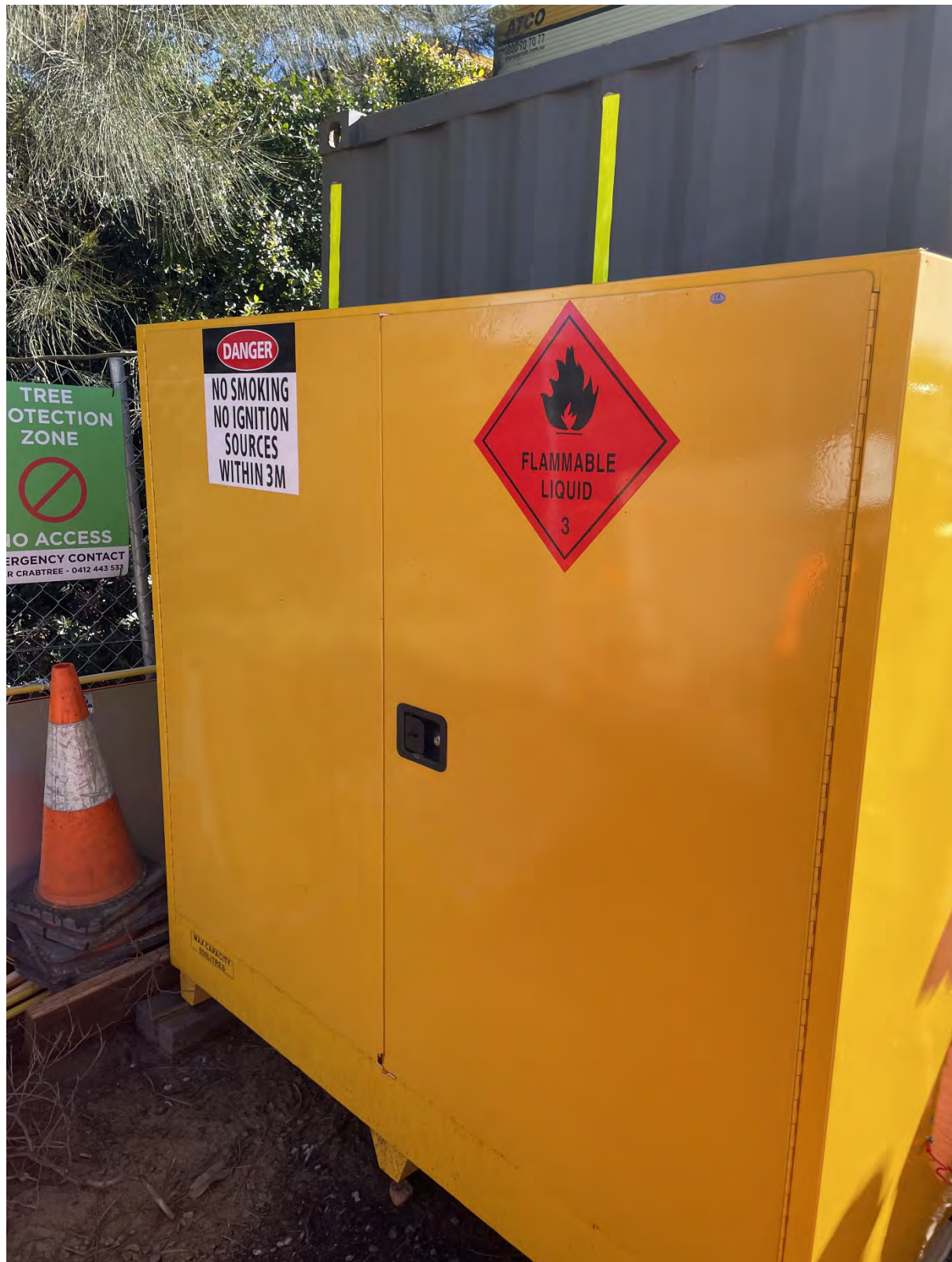
Figure 13 Flammable liquid storage
