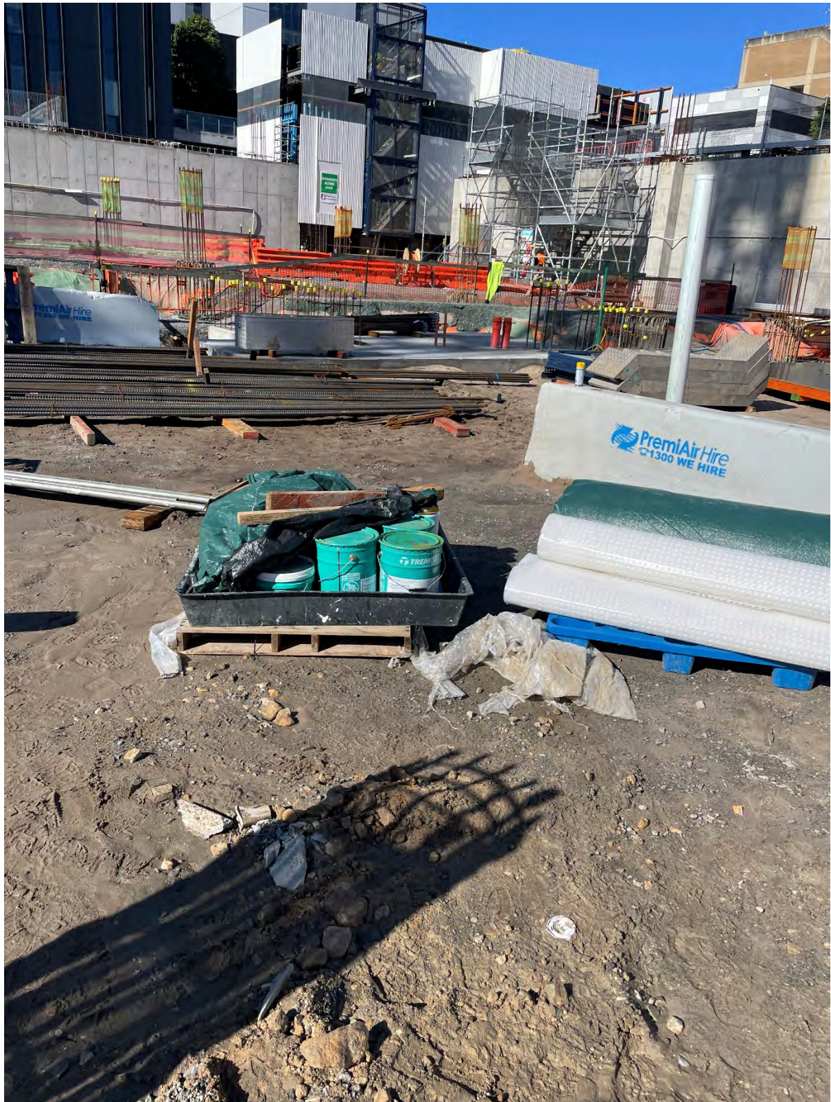
Figure 16 Bunded fuel and chemical storage with cover
