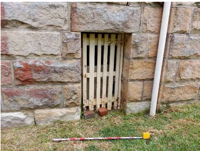
Photo 31 Facing southeast in 14 Bent Street showing disturbance from the construction of the 14 Bent Street cellar
