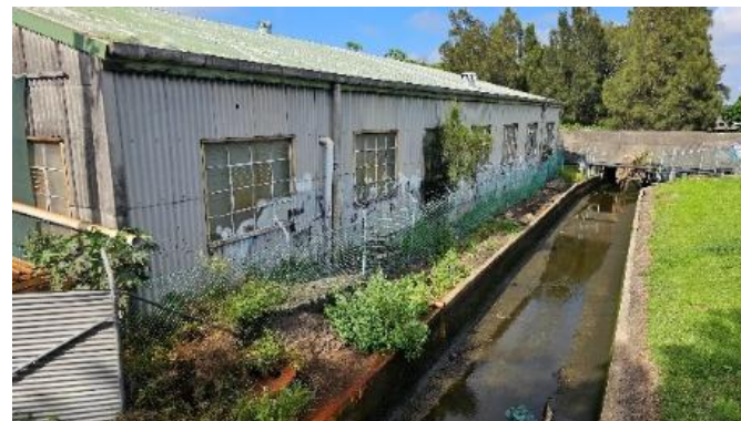
Figure 3. Current site conditions, north of the existing building, showing existing downpipe connections (to be removed).
