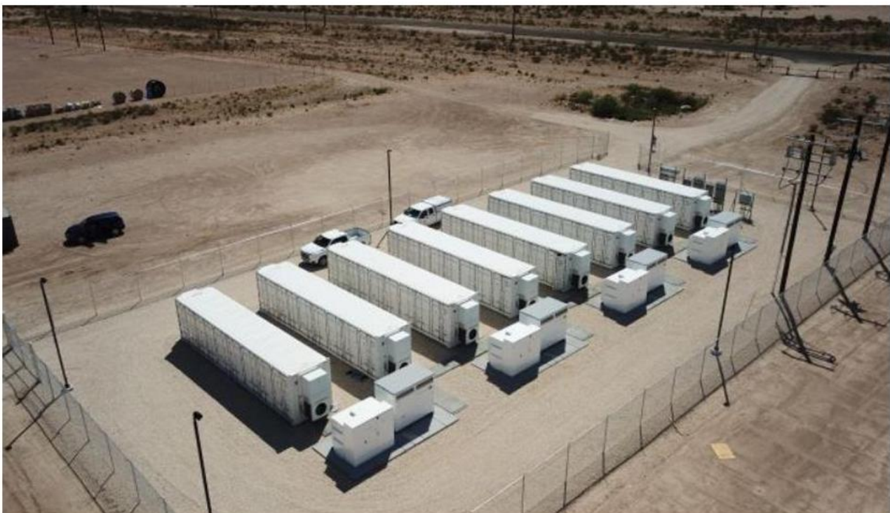
Photo 1.3 Typical Battery Storage Arrangement
