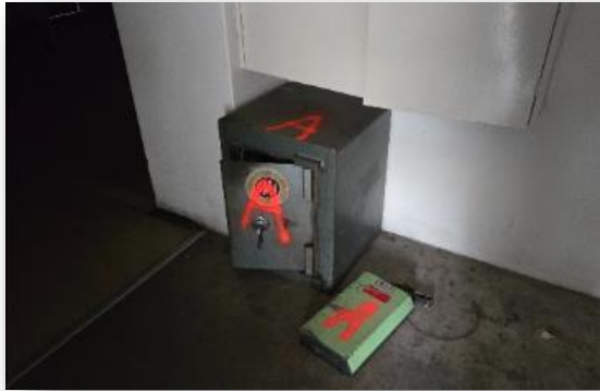
Example: Asbestos Millboard insulation to Safe
