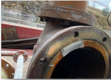
Exposed orange pipe (302-7) - Friable
