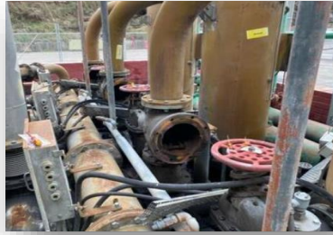
Yellow pipework (301-26) - Friable
