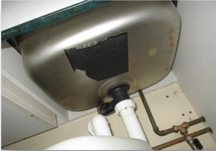
Example: Bituminous material under sink
