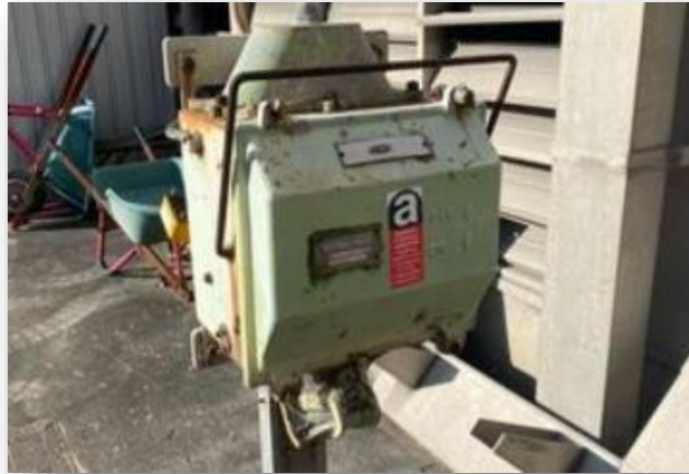
Example: Electrical switch with Asbestos woven rope
