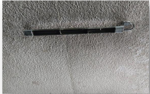
Example: Asbestos Millboard backing to Strip Heaters
