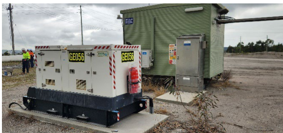
Generator near Southern Extension weather station
