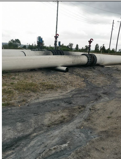
Pipe near weather station with stains indicative of previous leak.
