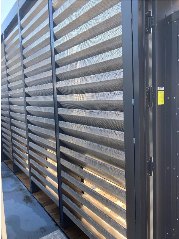
Noise softening panels, rooftop HVAC area
