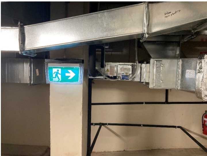
Ducted air conditioning
