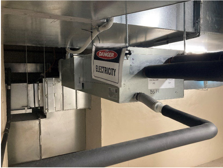
Ducted air conditioning
