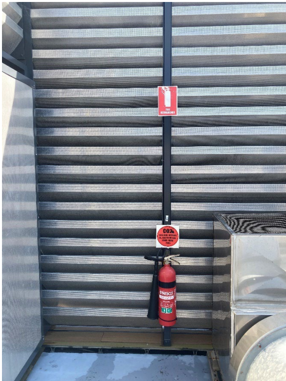
Noise softening panels and unobstructed fire extinguisher, rooftop HVAC area
