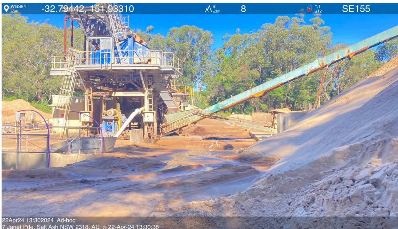
Sand screening and wash plant
